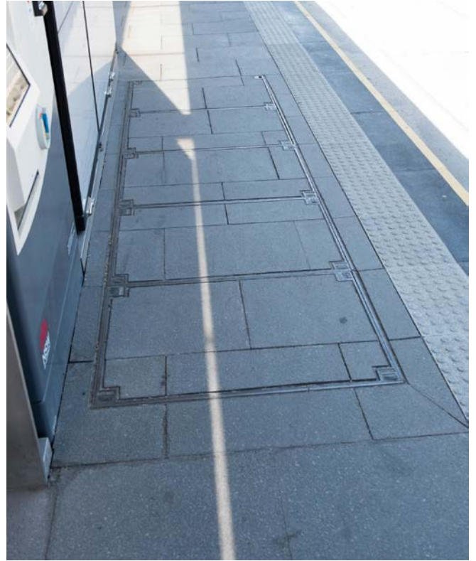
Figure 168. Service cabinet pit access on platform (CSELR)
