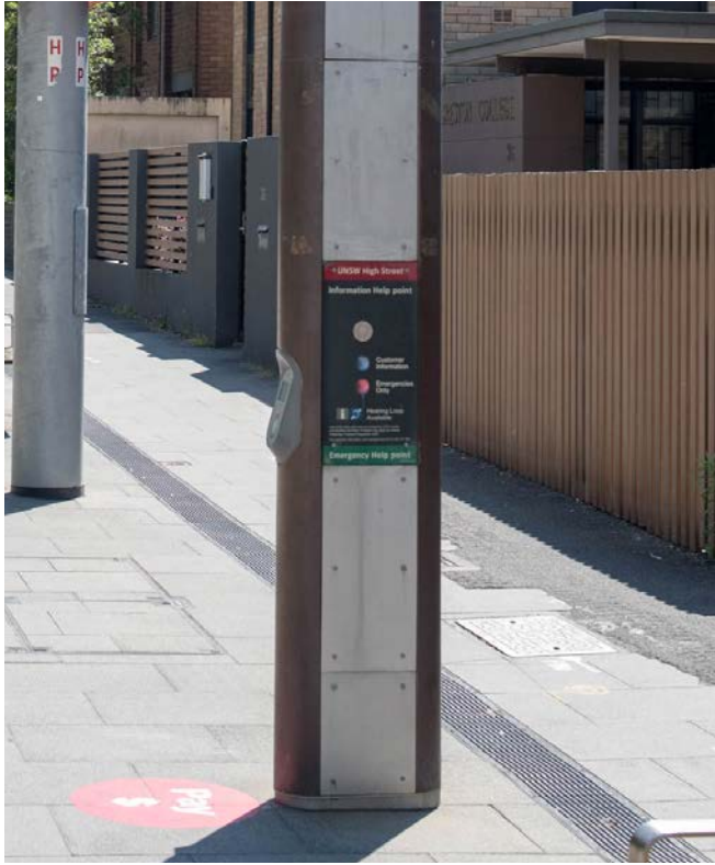
Figure 167. Help Point integrated into totem (CSELR, UNSW High Street)
