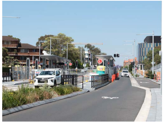
Figure 62. Non-signalised crossing across a single travel lane with balustrade dog-leg (PLR, Westmead Hospital)
