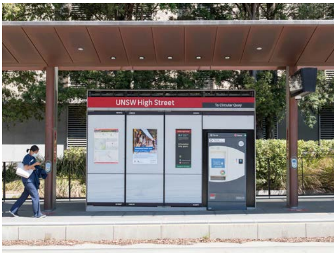
Figure 156. 4 module services cabinet (CSELR, UNSW High Street)
