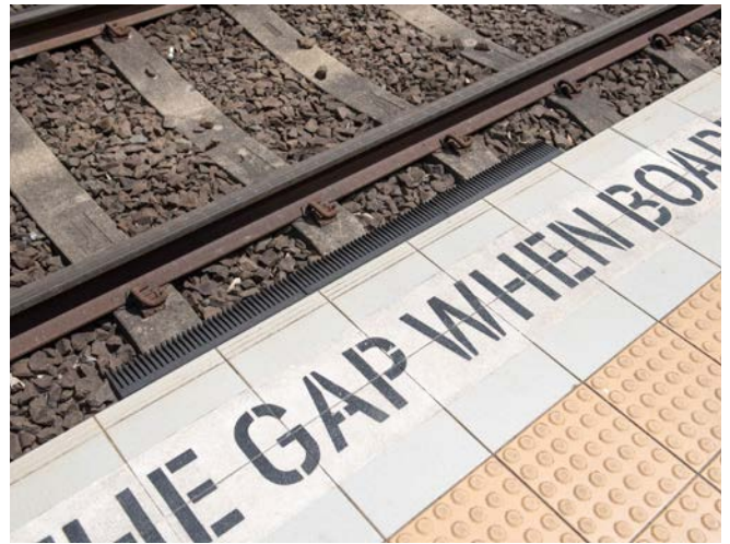
Figure 189. Gap filler as a retrofit solution on the older IWLRL line system; should not be necessary on new projects
