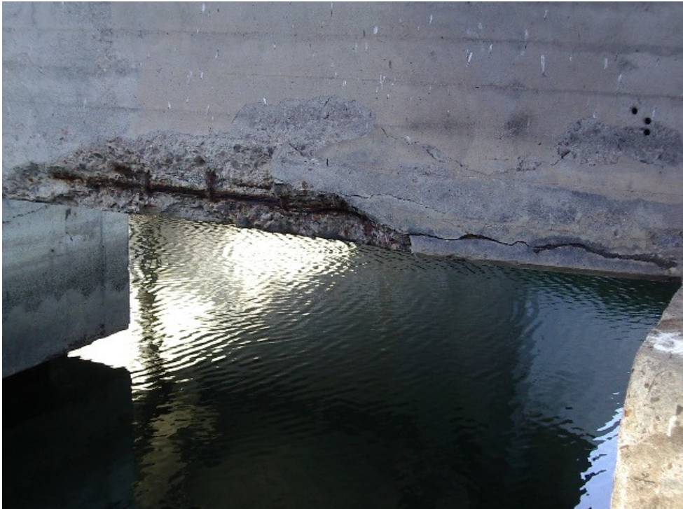
Significant spall with corrosion of exposed reinforcement.
