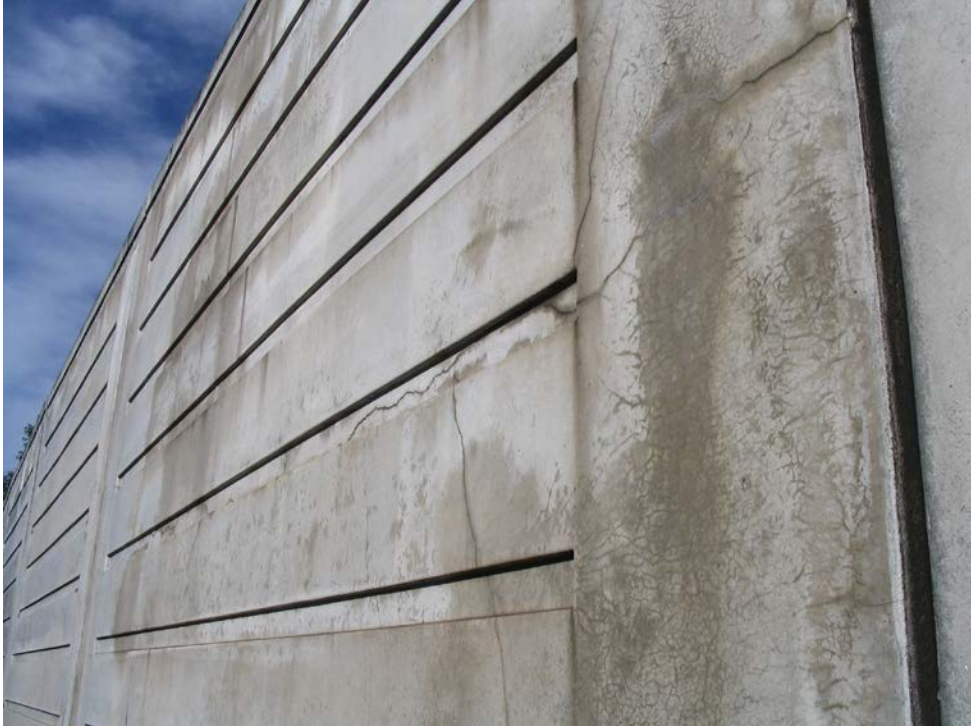
Cracks on a noise wall and supporting frame.
