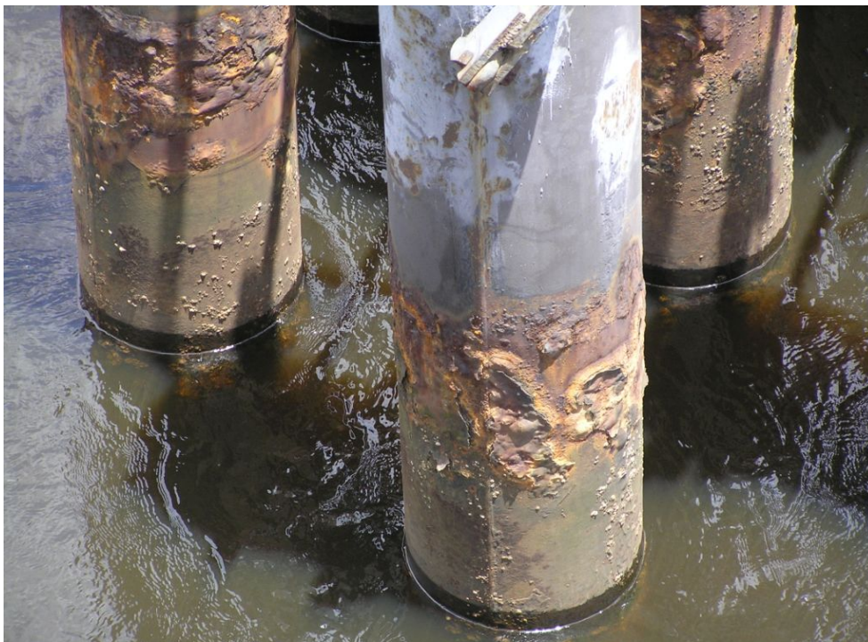
Heavy pitting on piles localised to the splash line.
