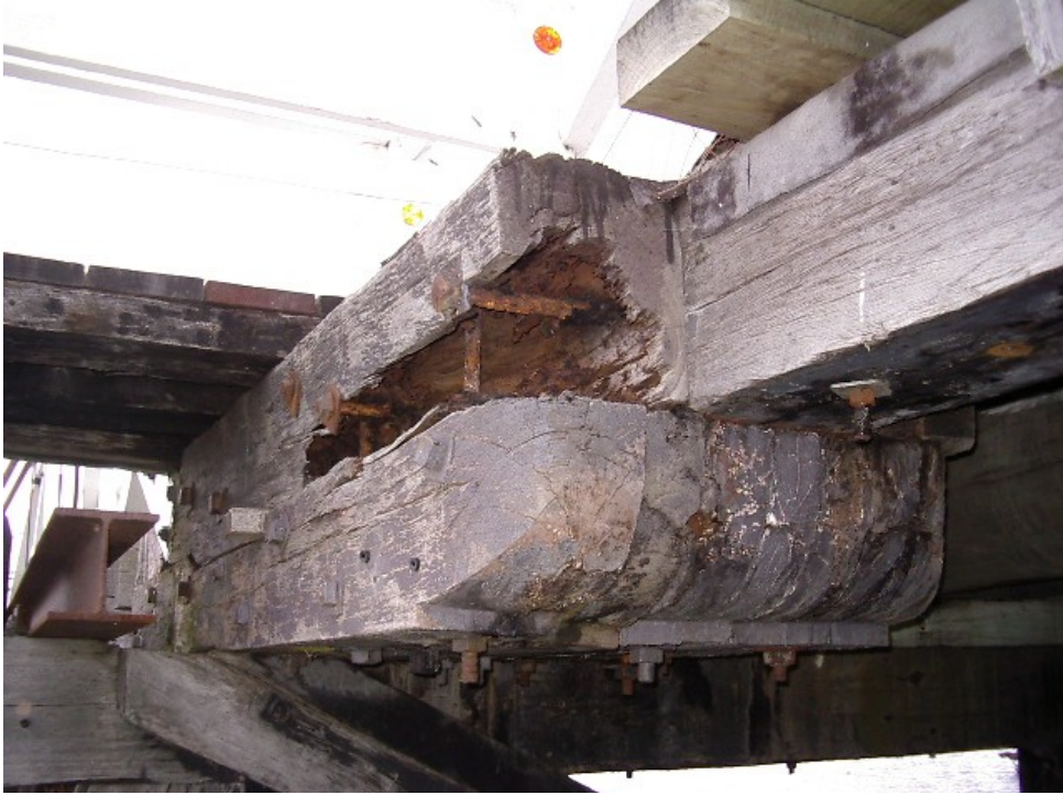
Badly rotten butting block.
