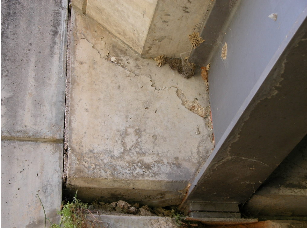
Significant crack ready to delaminate.
