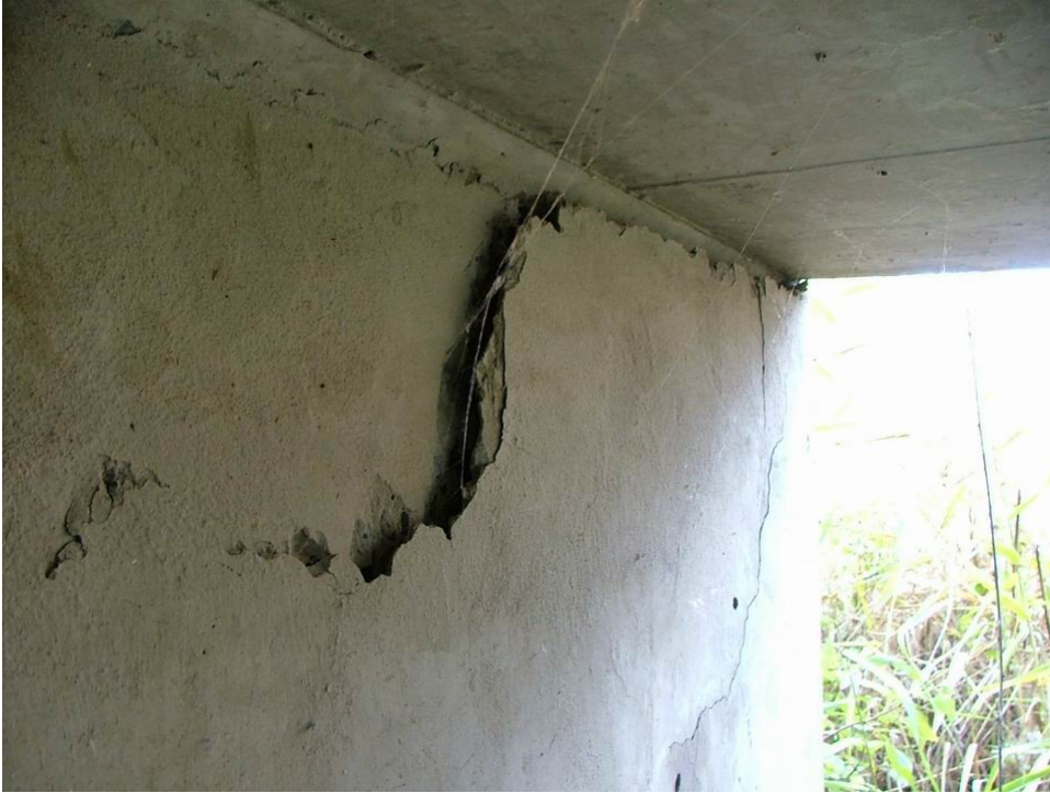
Large delamination of cell wall at inlet end where wingwall is being forced away.
