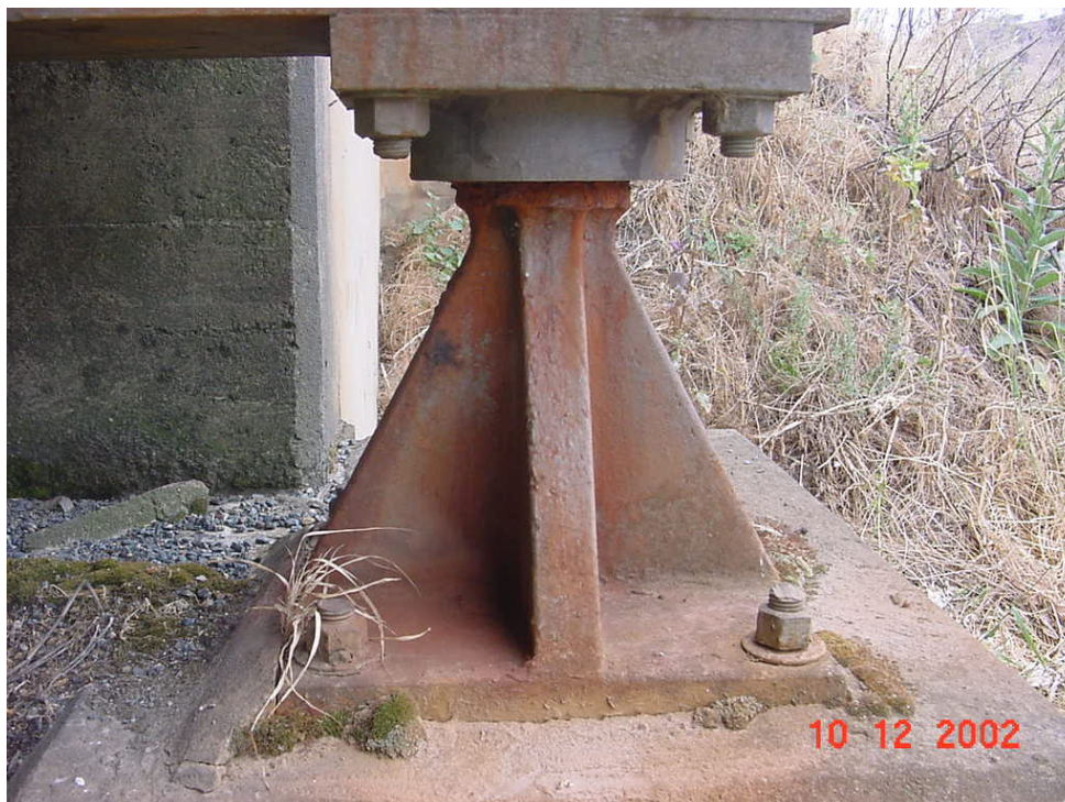
Surface corrosion of the bearing.
