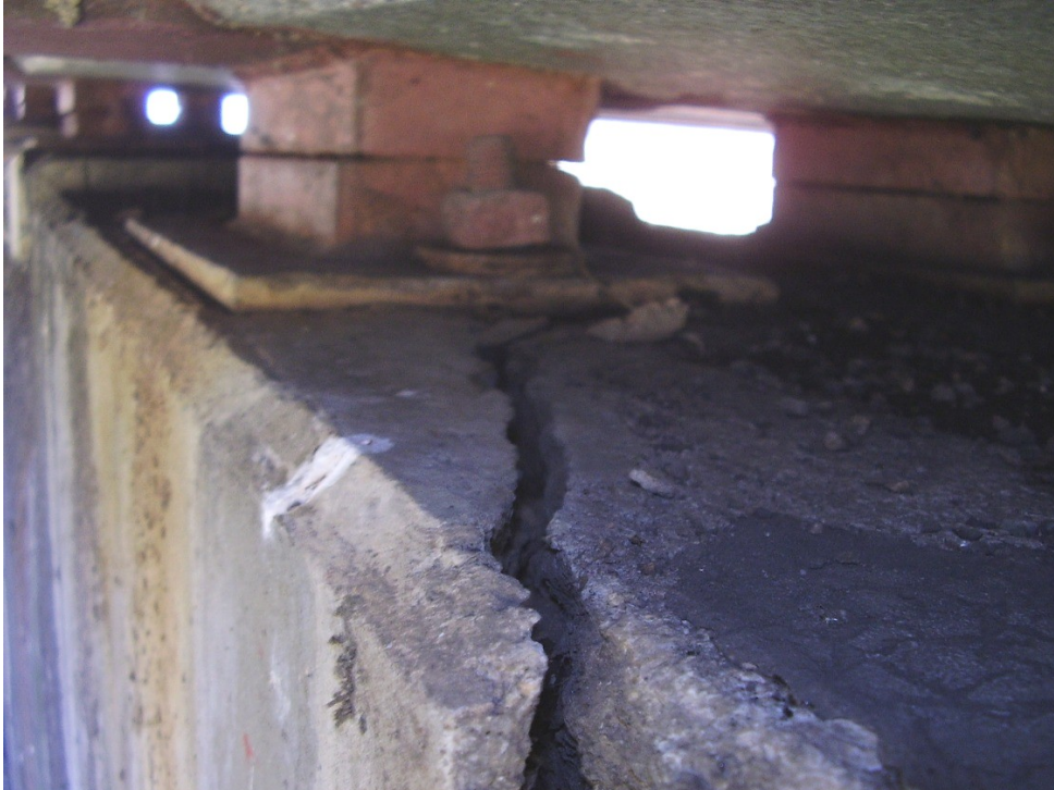
Wide crack splitting the headstock under the bearing
