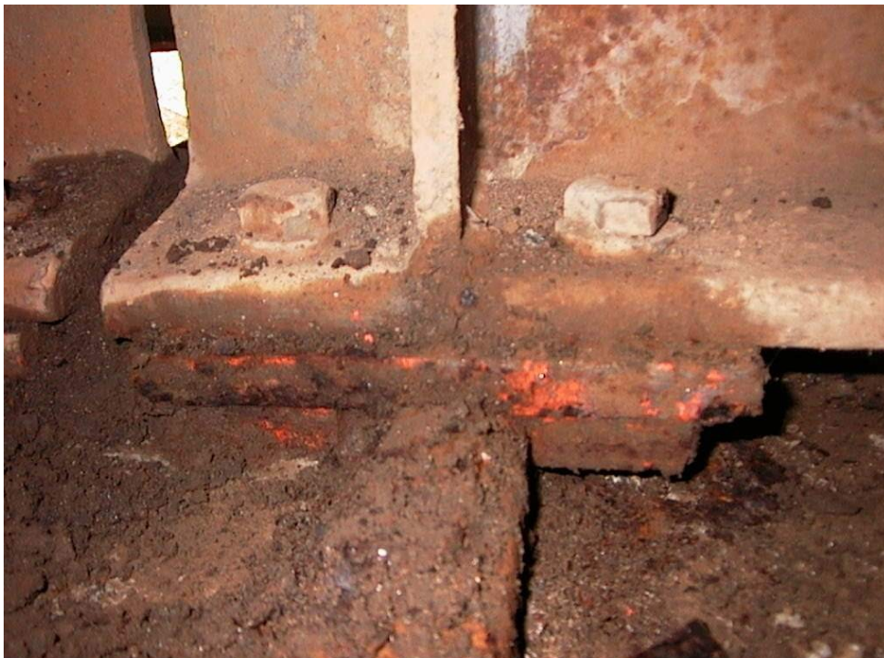
Significant corrosion with pitting.
