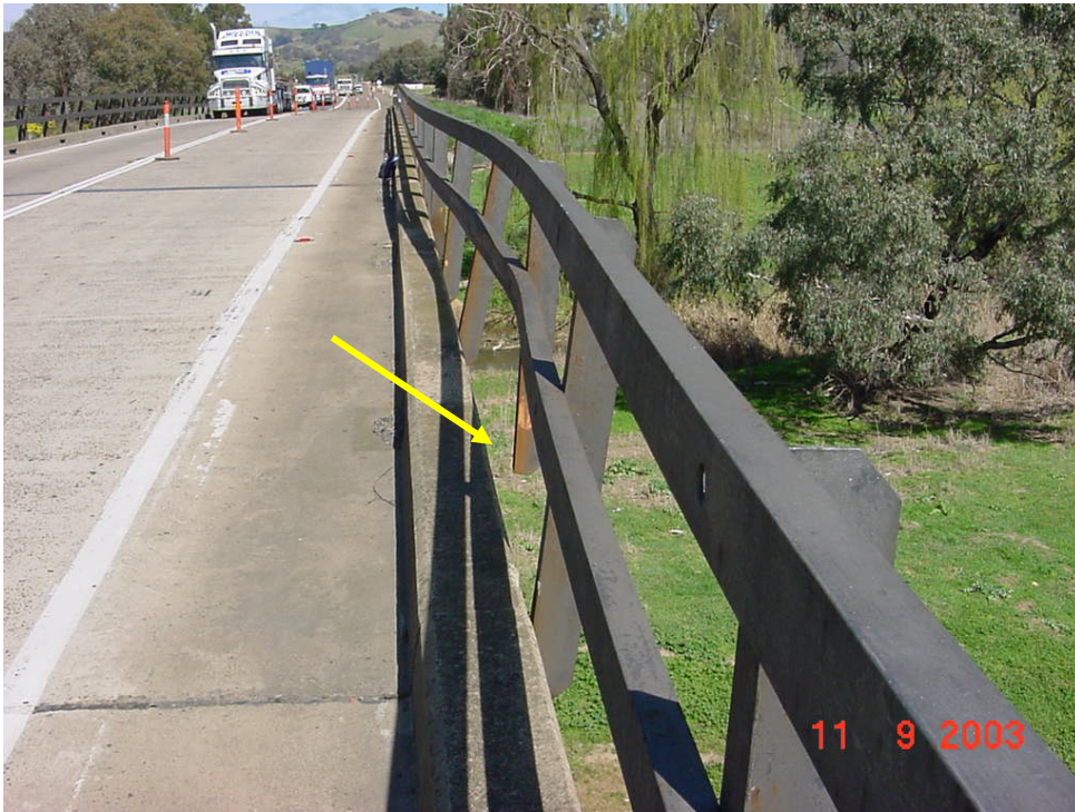
Accident damage with unsupported railing over a short length.
