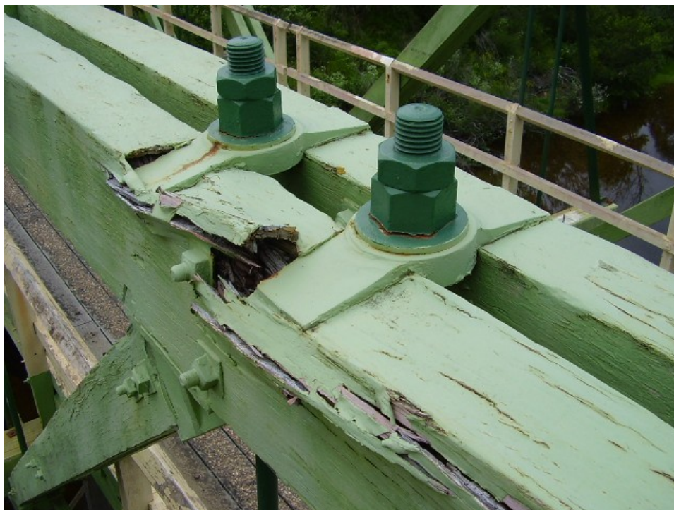
Badly rotten top chord crushing near the support of steel verticals.
