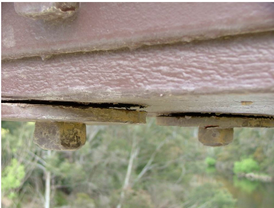
Slightly loose vertical splice bolts at top chord.
