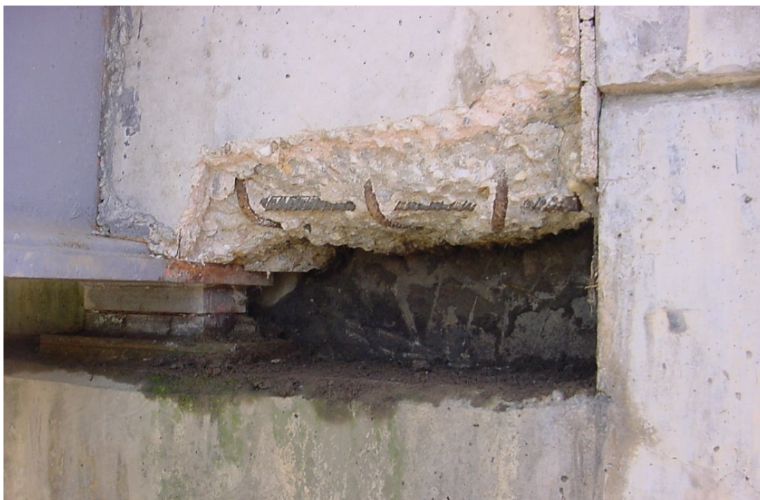
Significant spalling at the bottom of diaphragm. Exposed reinforcement.
