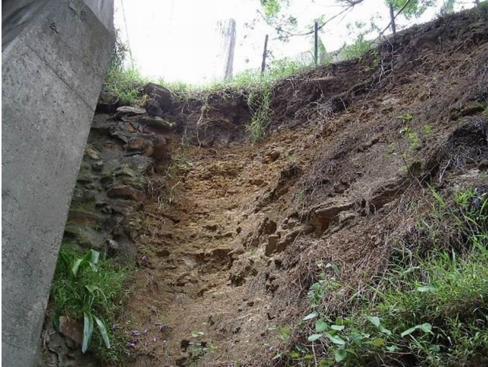
Significant erosion of embankment.
