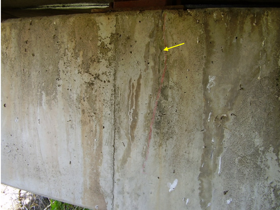
Vertical crack under the bearing
