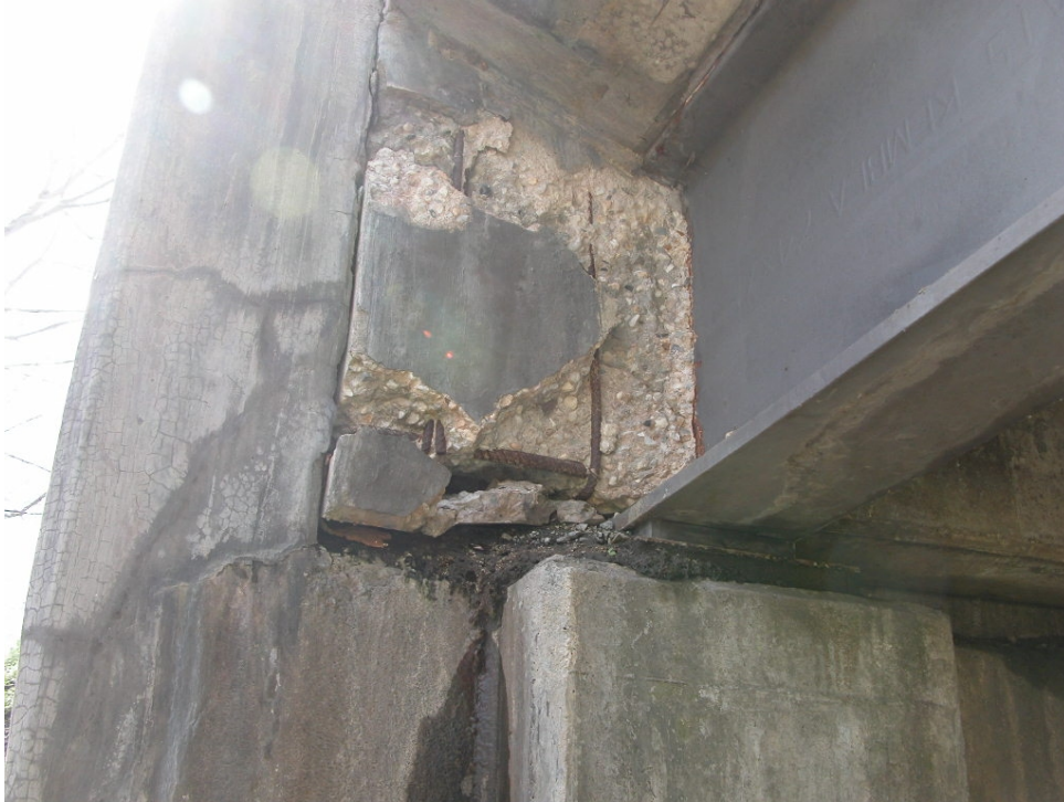
Crushed concrete diaphragm with exposed reo.
