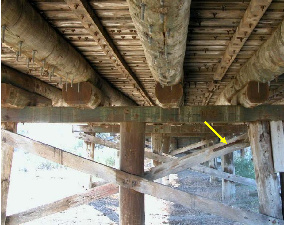
Minor decay of the wale.
