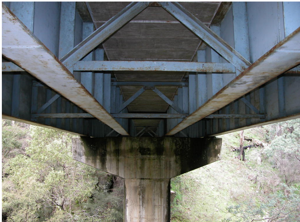
Extensive corrosion at flange edges.
