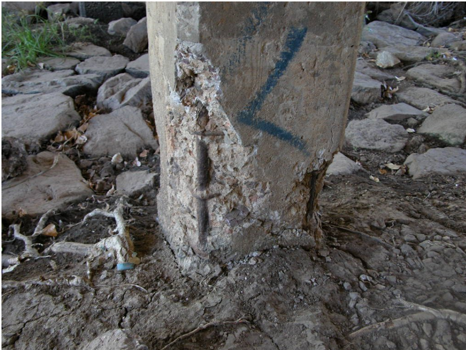
Significant spall with exposed reinforcement.
