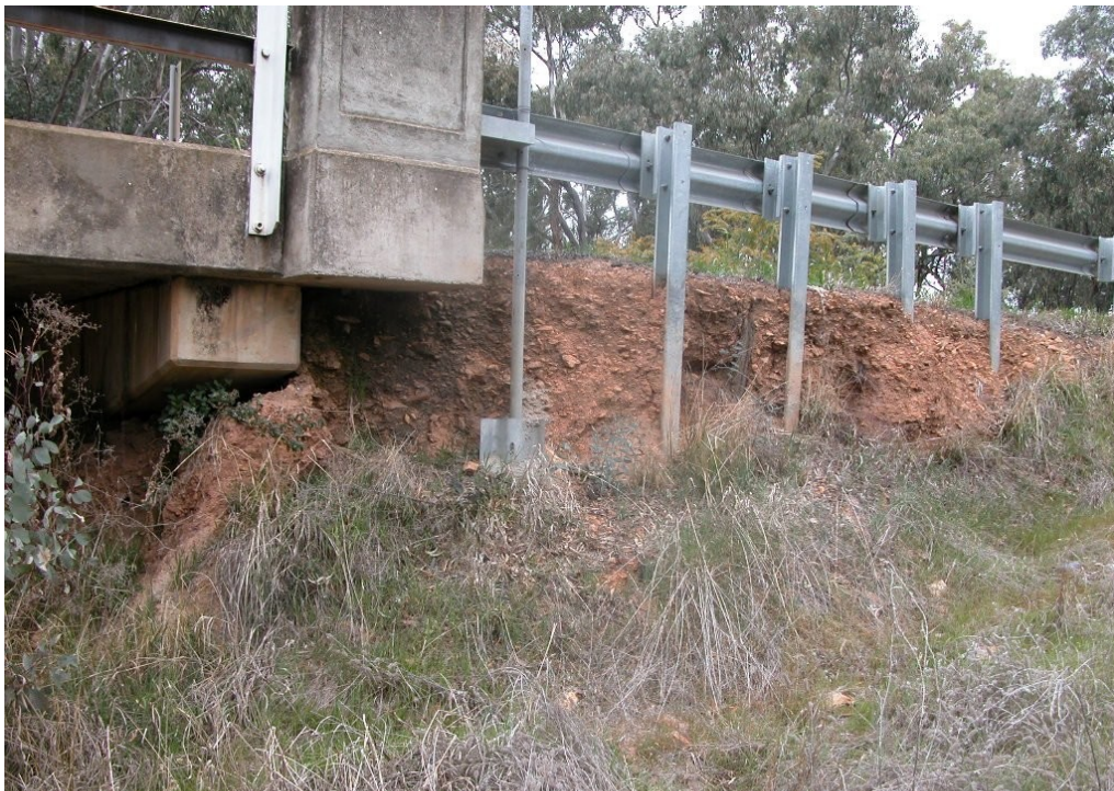
Significant undermining and scour under abutment and approaches.
