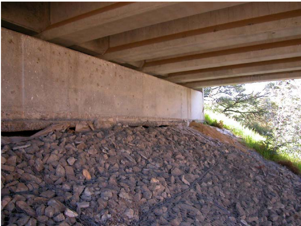
Settlement of the embankment.
