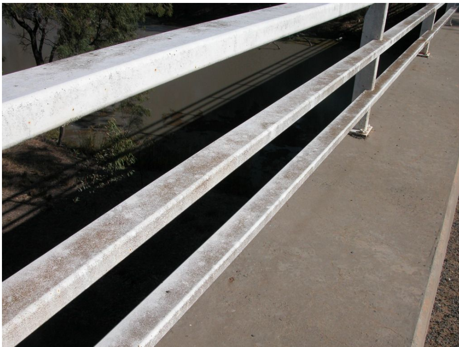
Protective coating showing signs of distress but is still reasonably effective.
