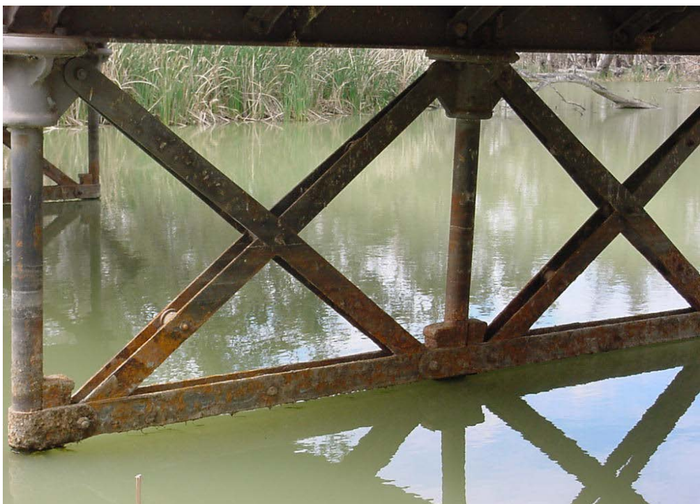
Heavy pitting on steel pier.
