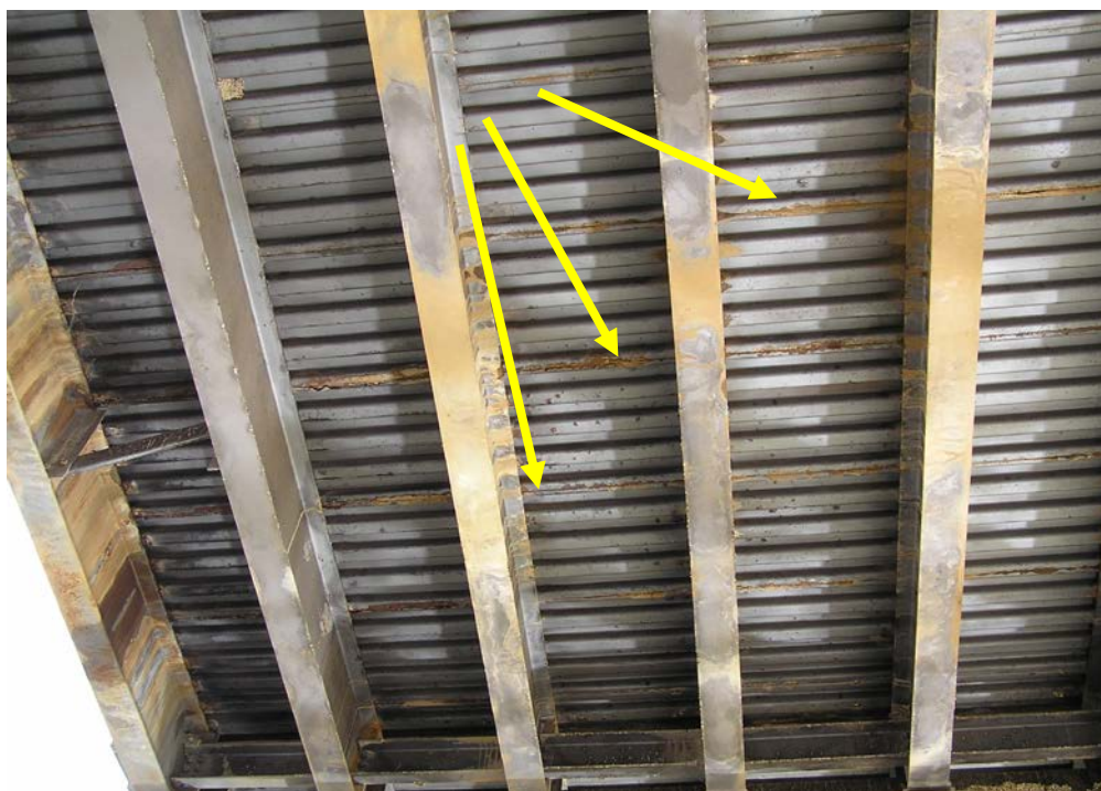
Moderate corrosion at all deck connections.
