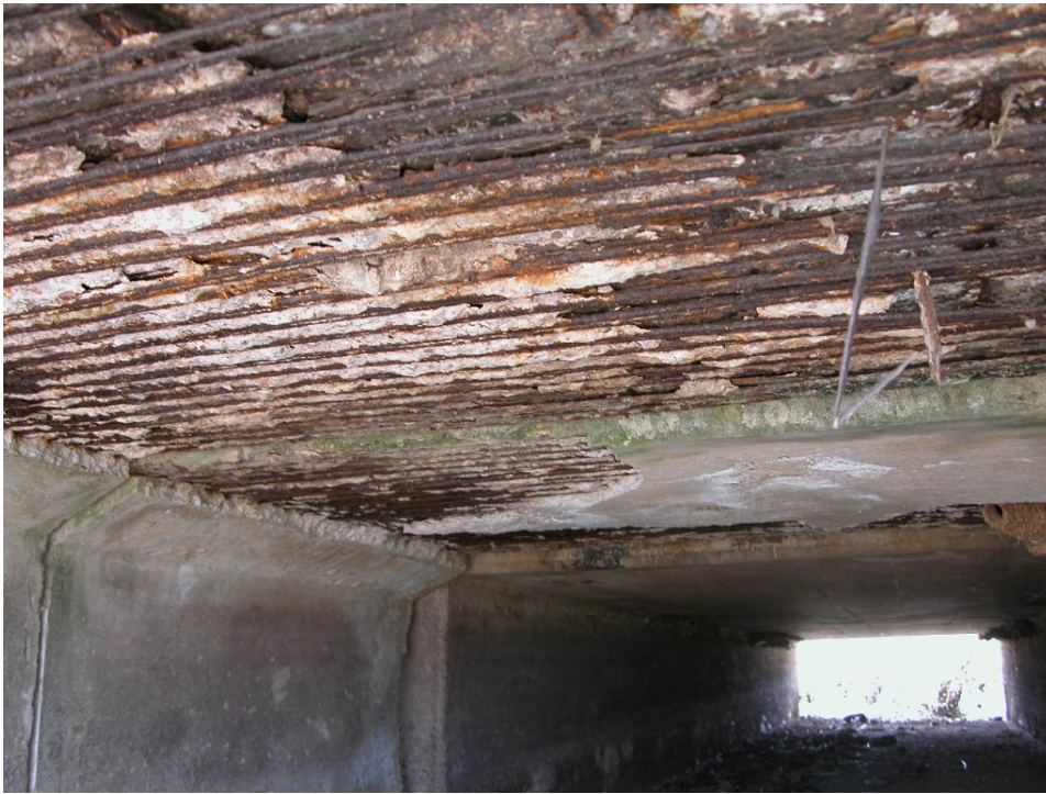
Extreme delamination and corrosion exposed reinforcement of precast units.
