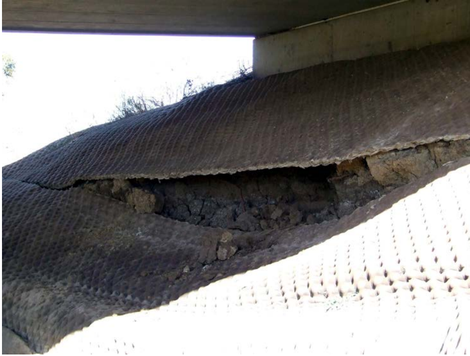
Fabric protection partially collapsed due to settlement.
