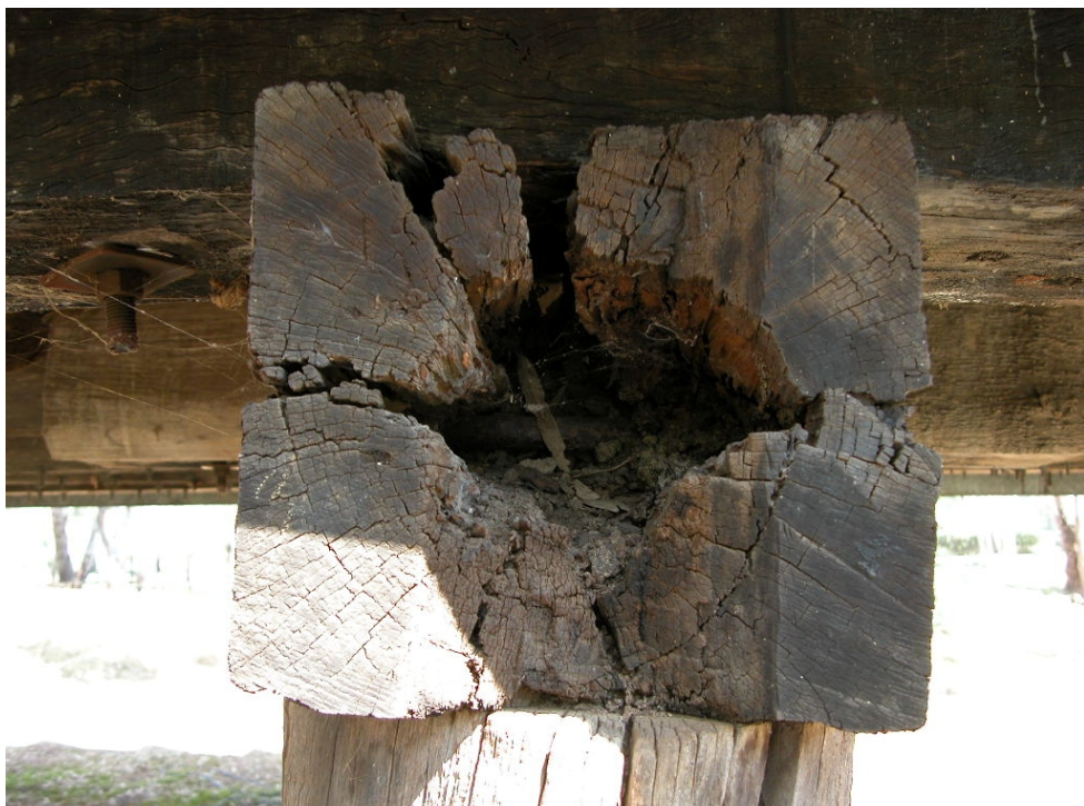
Badly rotten timber headstock.
