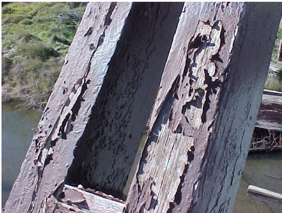
Coating has failed in significant areas.
