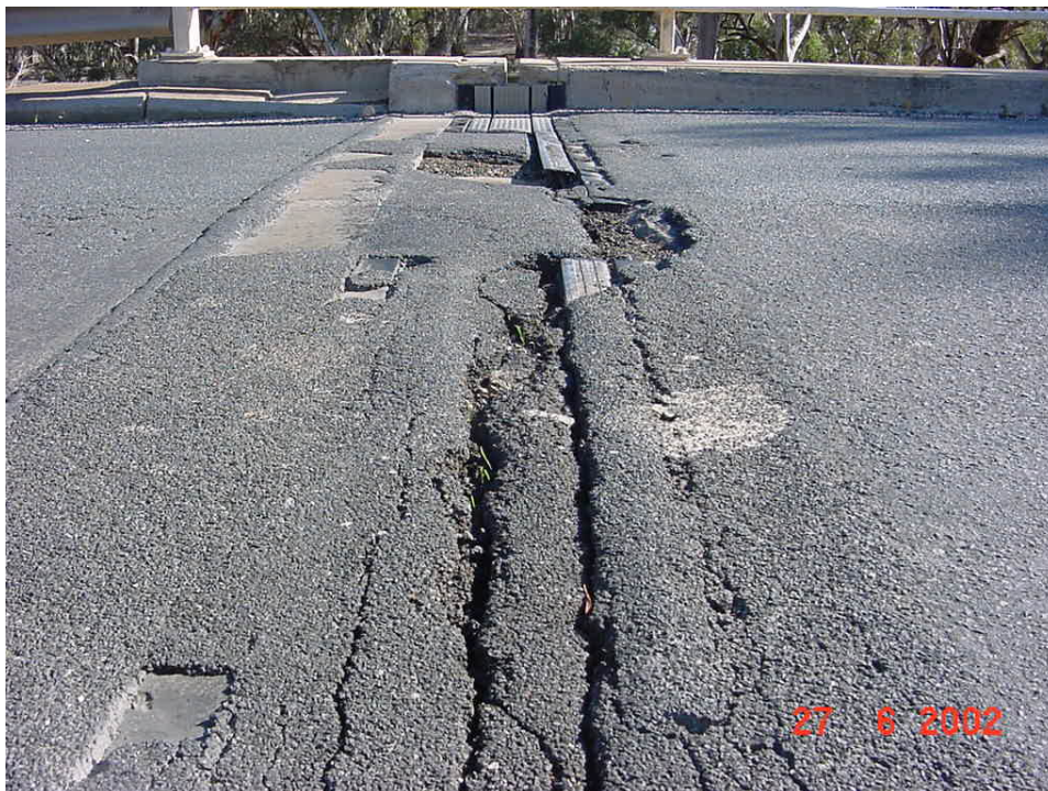
Joint in poor condition.
