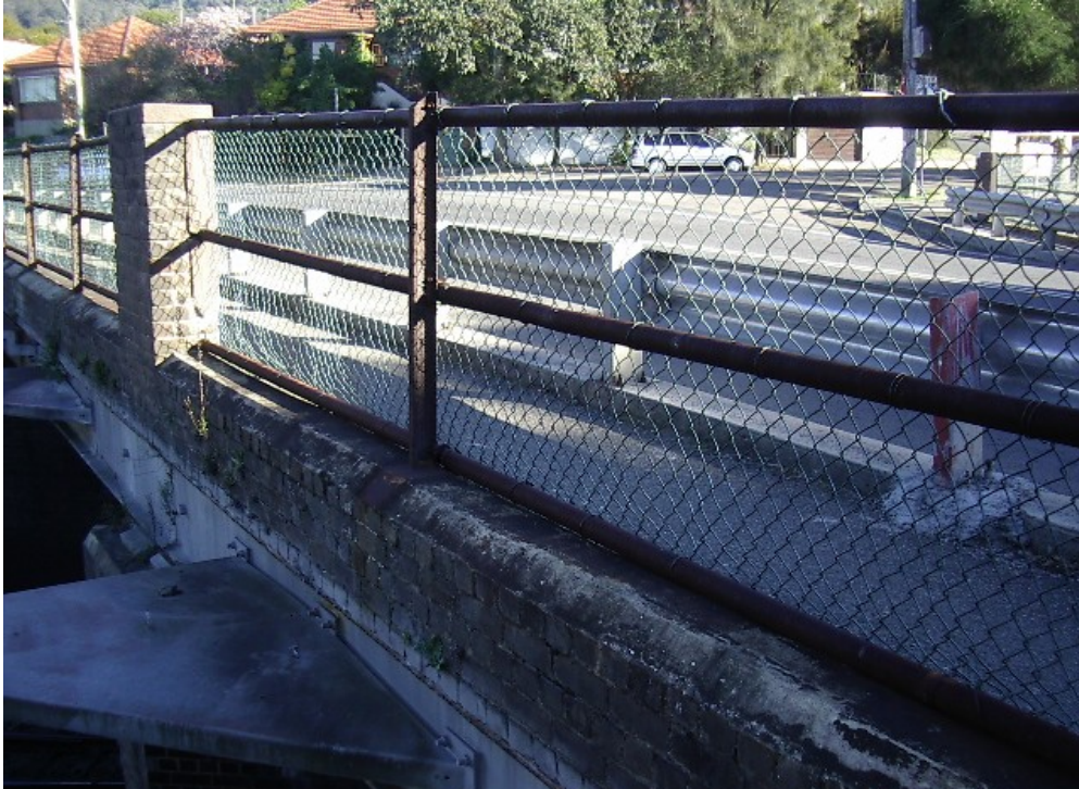
Corrosion of metal components.
