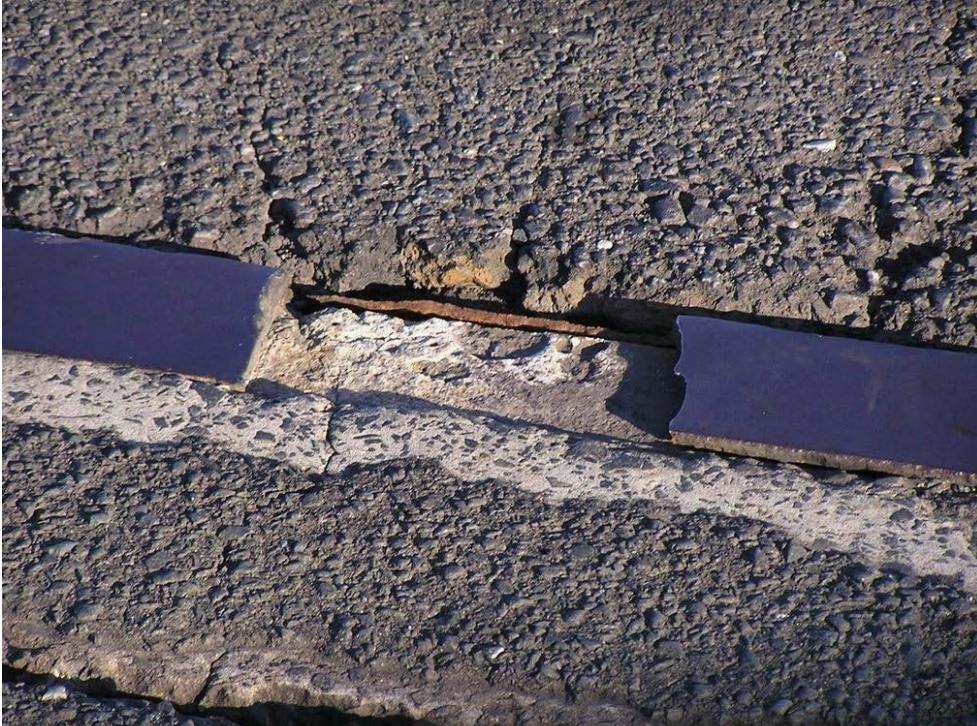
Loose and broken protection angle.
