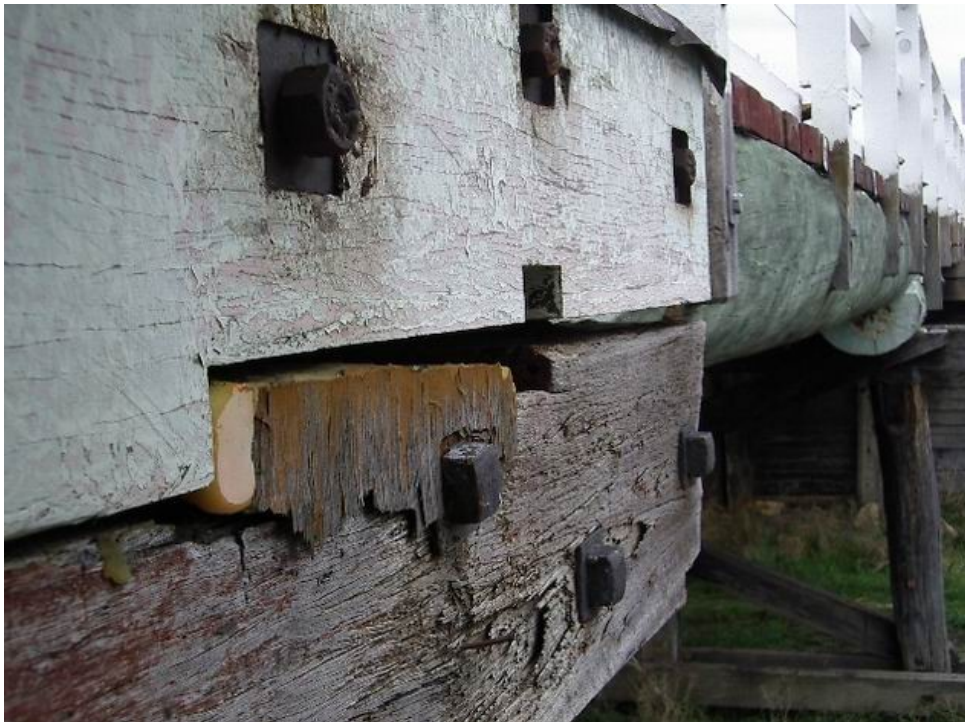
Integrity of the shear key is doubtful with significant separation of the butting block members.
