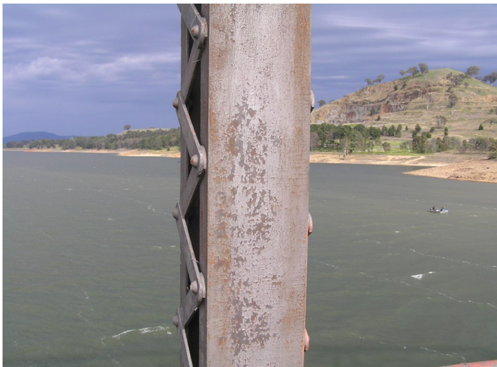
Large areas of topcoat deterioration with primer exposed.
