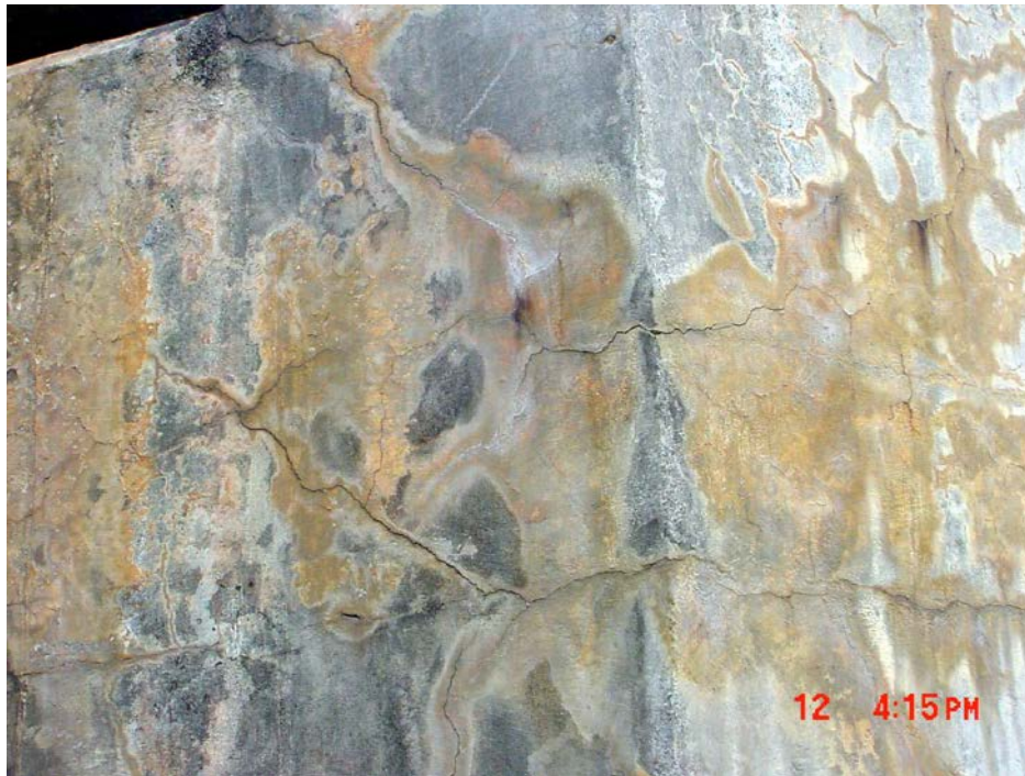
Severe AAR cracking on a headstock
