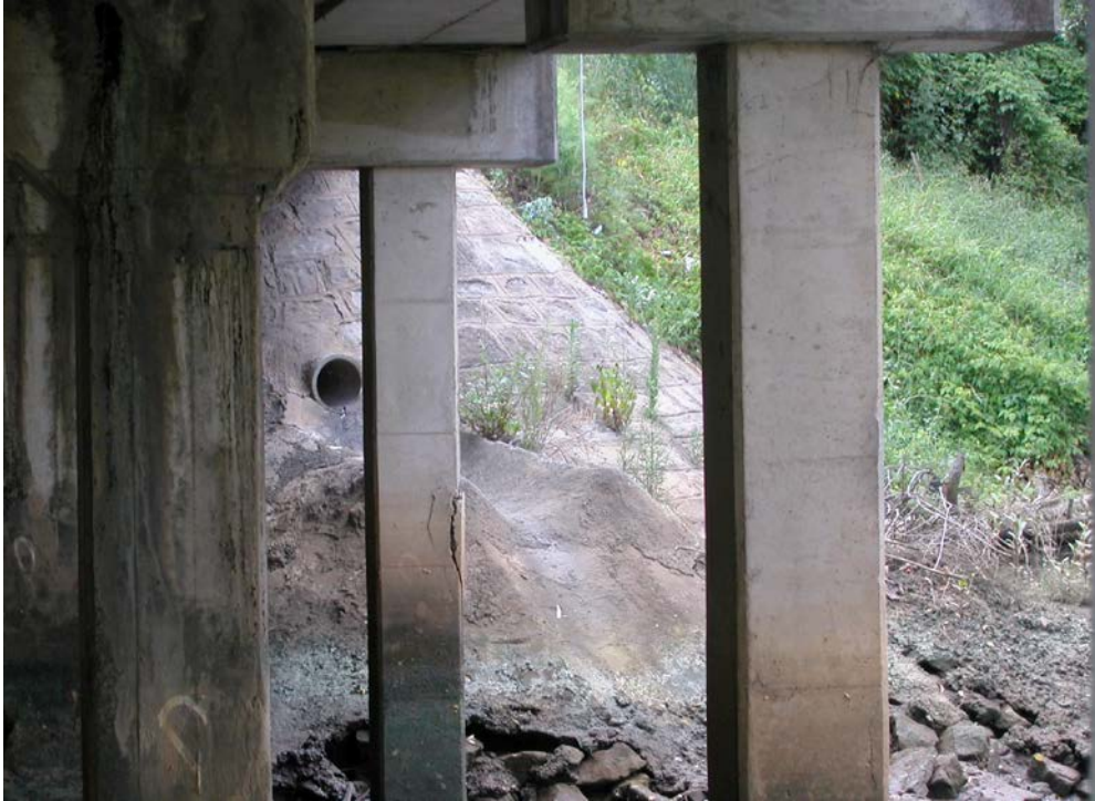
Some delamination of a corner of a pile ready to spall.
