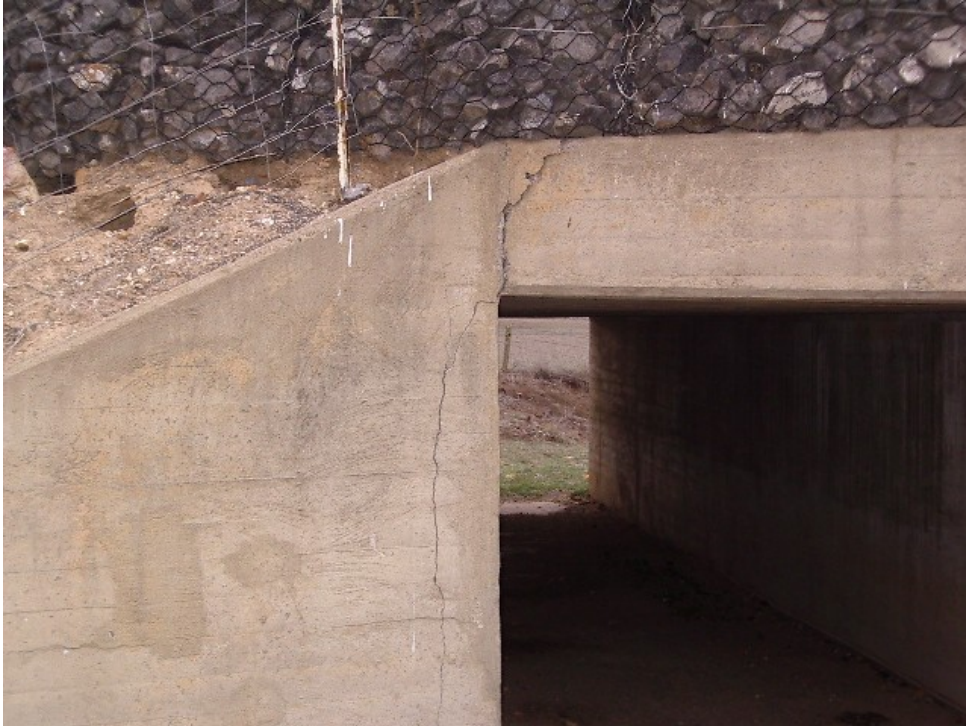
Vertical cracking on the wingwall culvert cell
