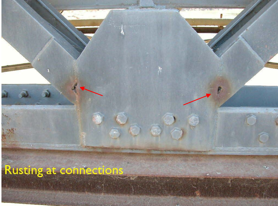
Corrosion and section loss at gusset plate welded connections.
