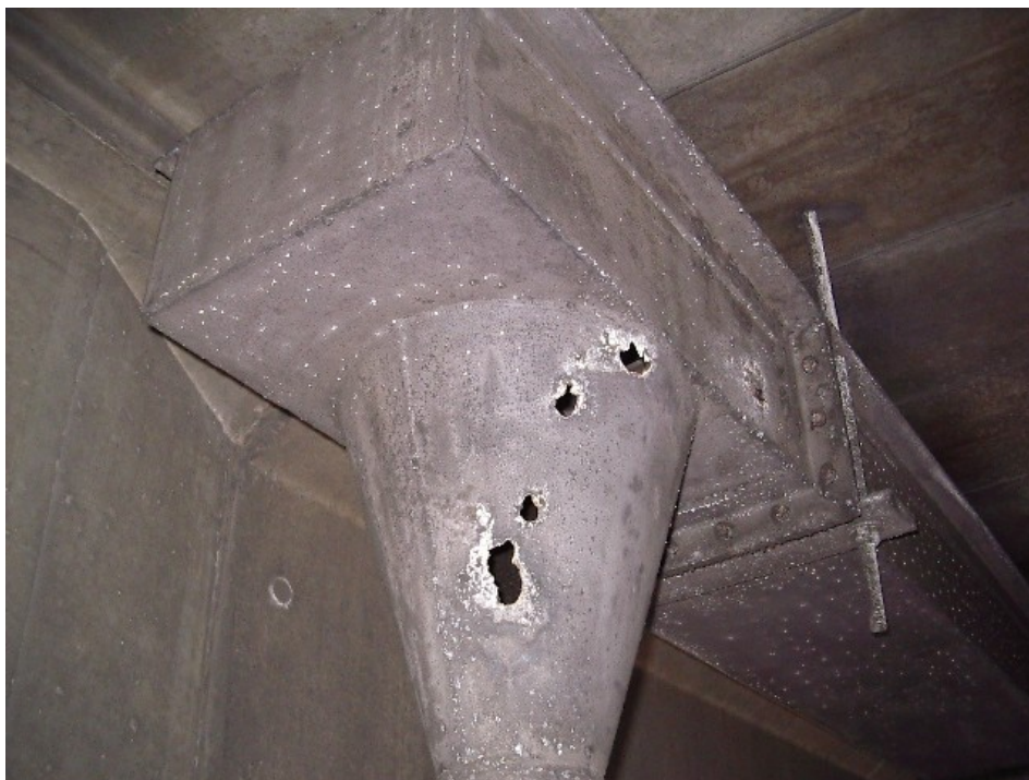
Drainage downpipe with holes.
