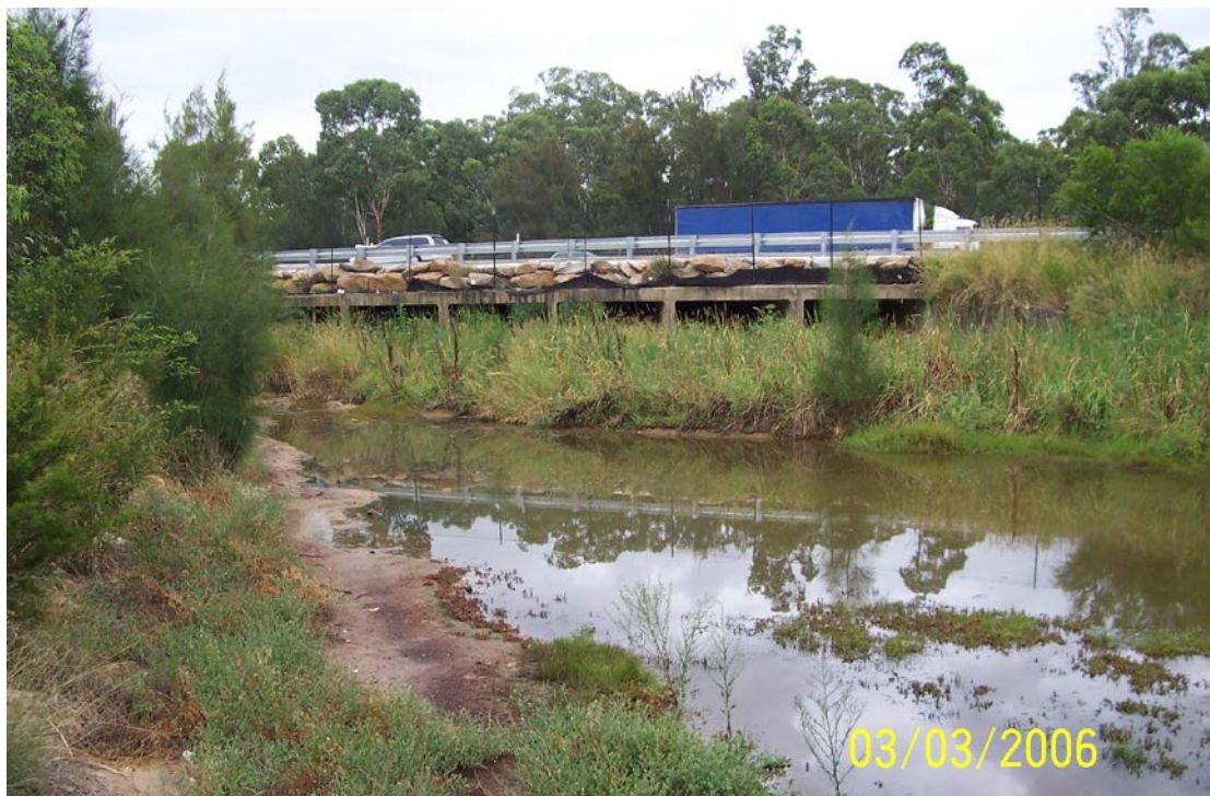
Waterway showing about 20% siltation with ponding water.
