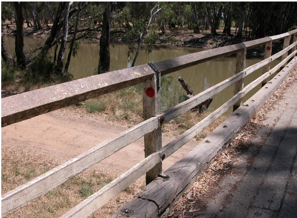
Timber railing in good condition with failed paint coating.
