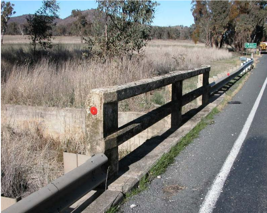
Concrete railing with minor spall.
