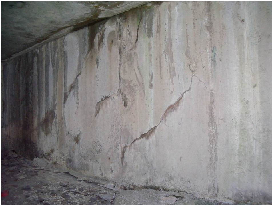
Significant diagonal cracking.
