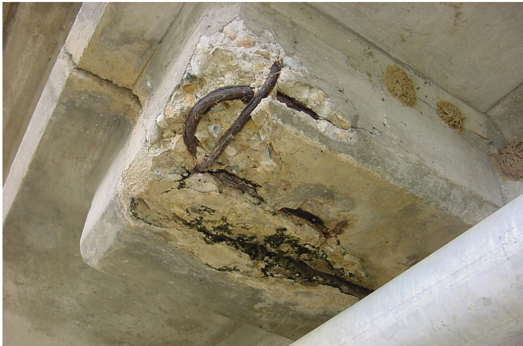
Spalled concrete with exposed reinforcement.
