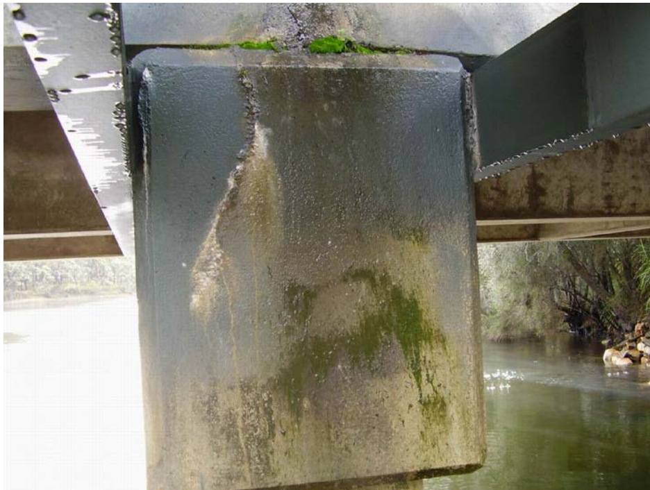
Crack with leaching on the end of headstock
