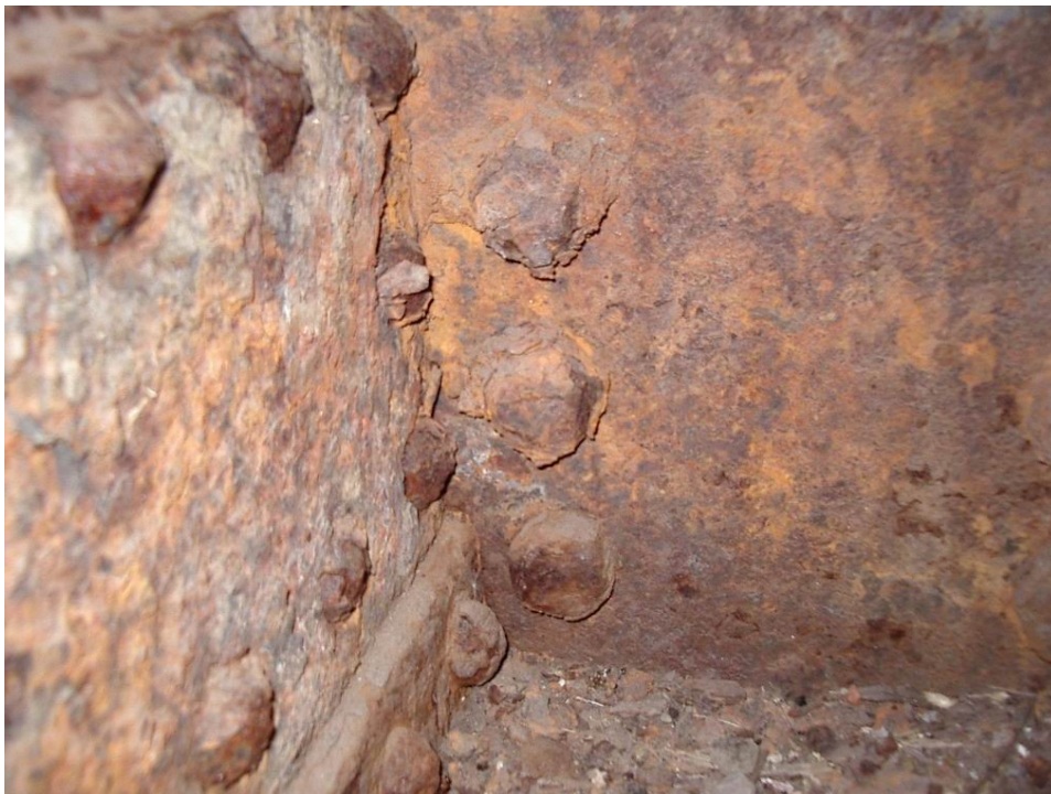
Heavy pitting and the bolt heads corroding away.
