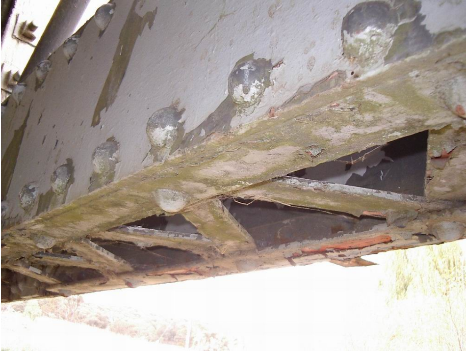
Surface rust and minor pitting at the bottom.
