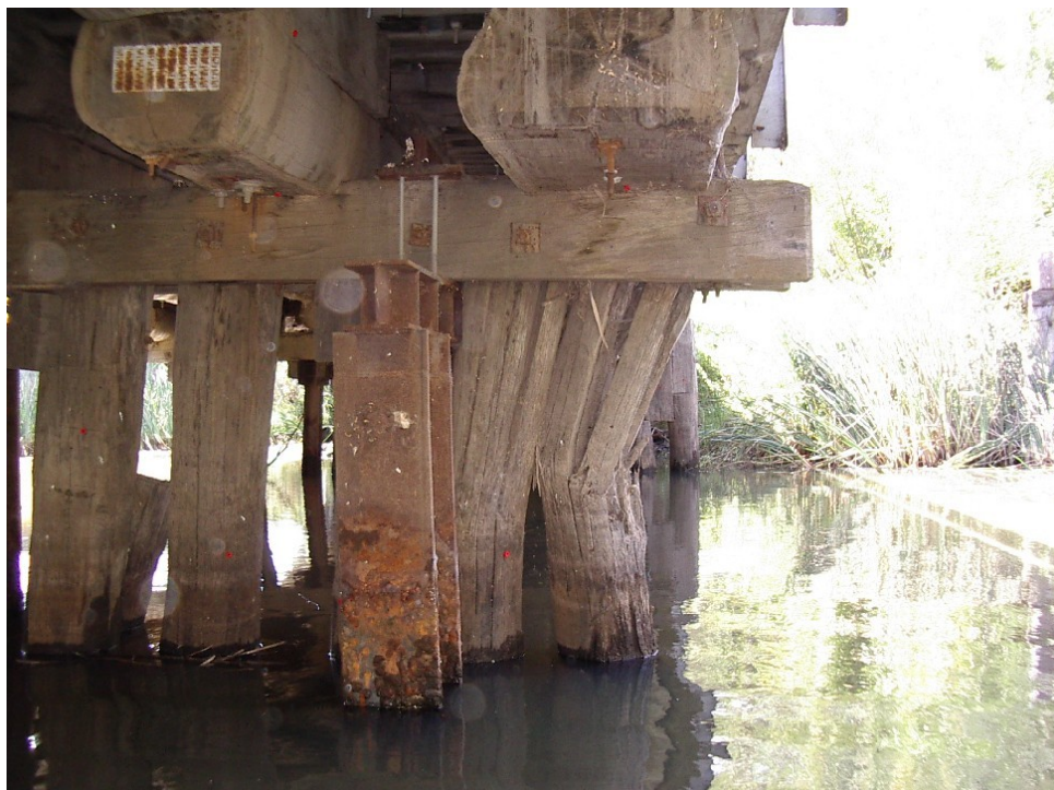
Failed timber piles.
