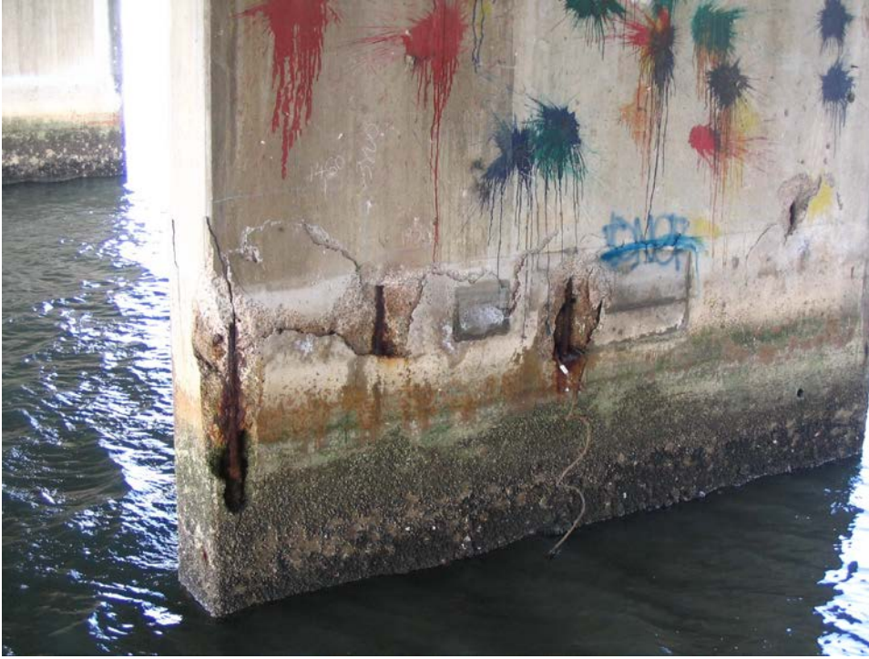
Significant loss of section of reinforcement.
