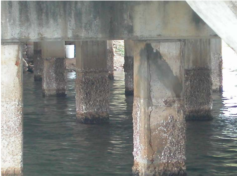
Repaired piles cracking again.
