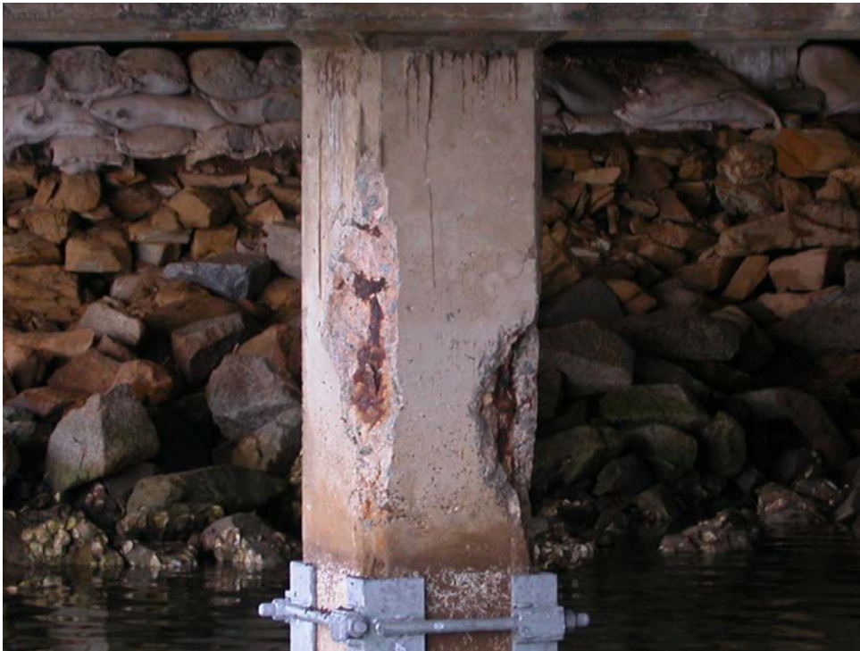
Advanced deterioration. Significant loss of section. Significant vertical cracks on all faces where the pile is braced in the steel frame.
