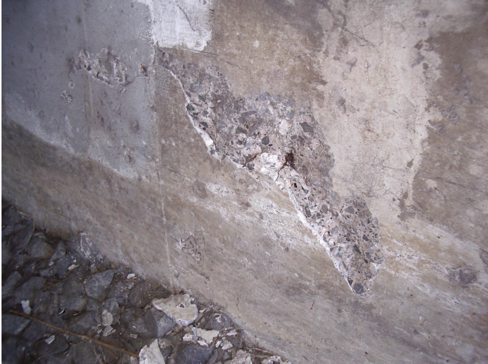
Spalled area at base of abutment.
