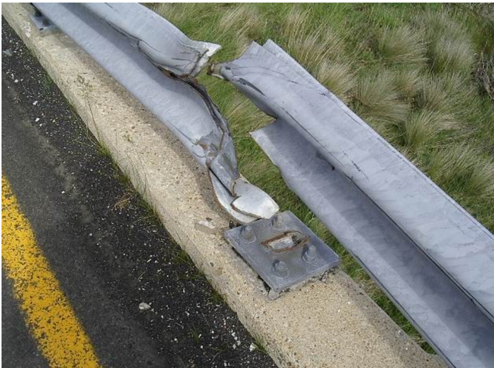
Badly damaged metal railing with missing post and torn guard fence rail.
