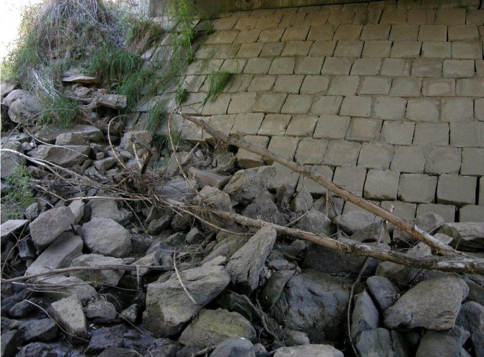
Batter protection undermined by scour at the base.
