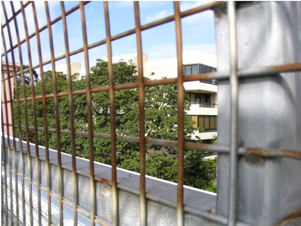
Rust forming on the screen.
