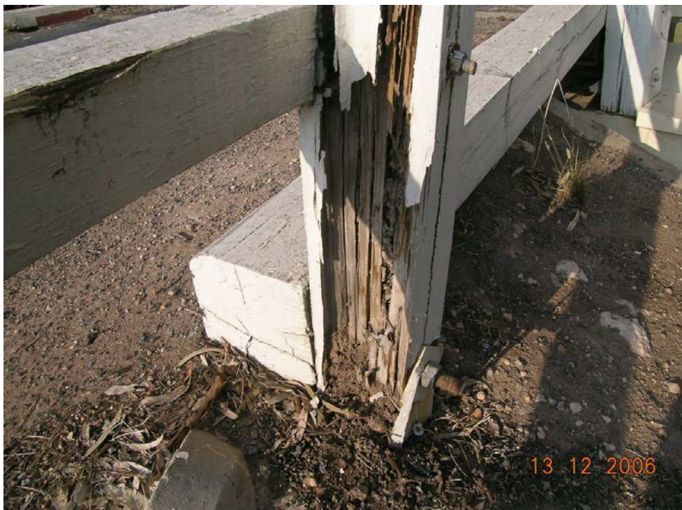
Badly deteriorated timber rail post.
