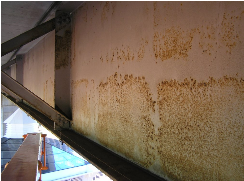
Surface rusting on web of girder.
