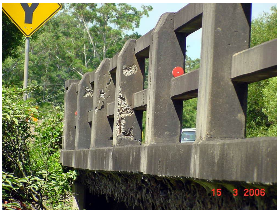
Spalls and exposed reinforcement.
