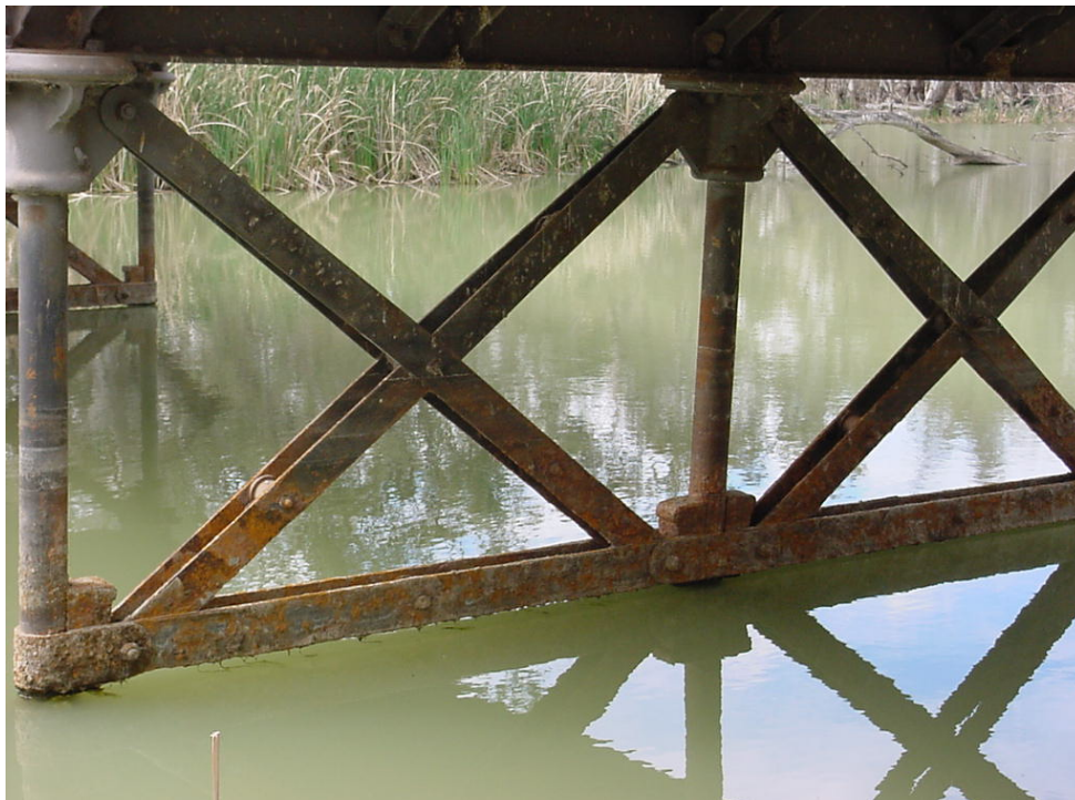
Failed coating and significant corrosion of pier bracing.
