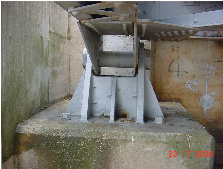
Signs of surface corrosion.
