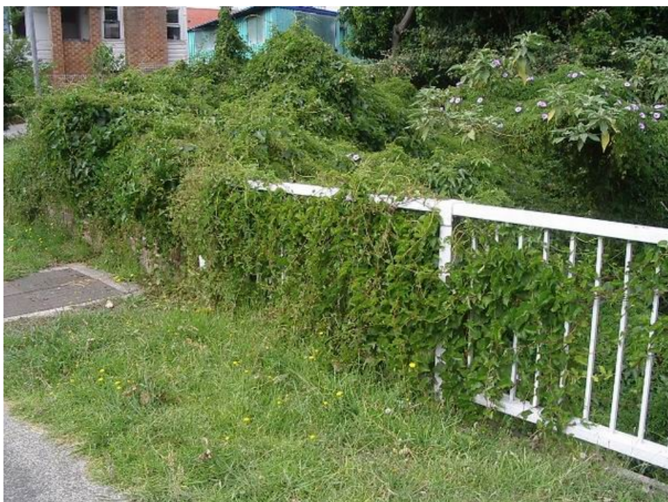
Overgrowth of vegetation covering bridge railing and any delineator sign on the end post.
