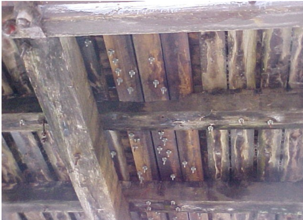
Medium decay of cross decking.
