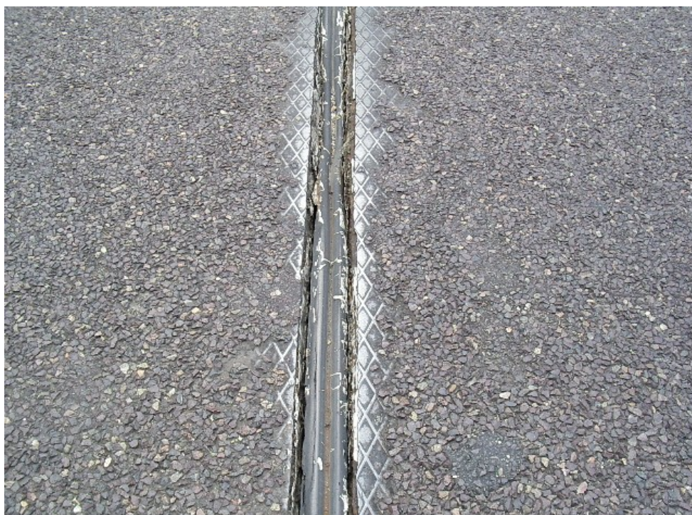
Moderate loss of adhesion on either side of the compression seal.
