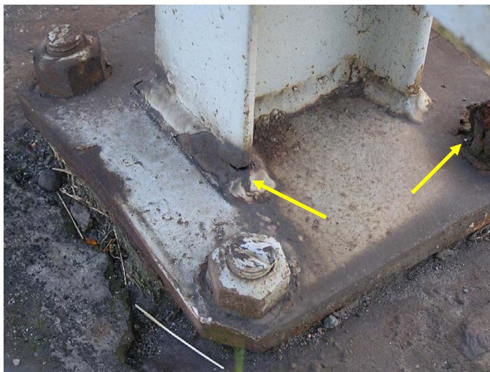
Weld crack at the base and corrosion of nut.
