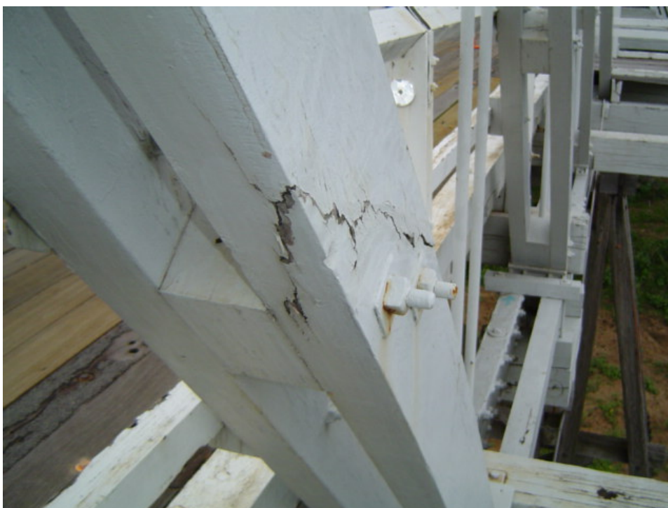
Failed diagonal strut flitch.
