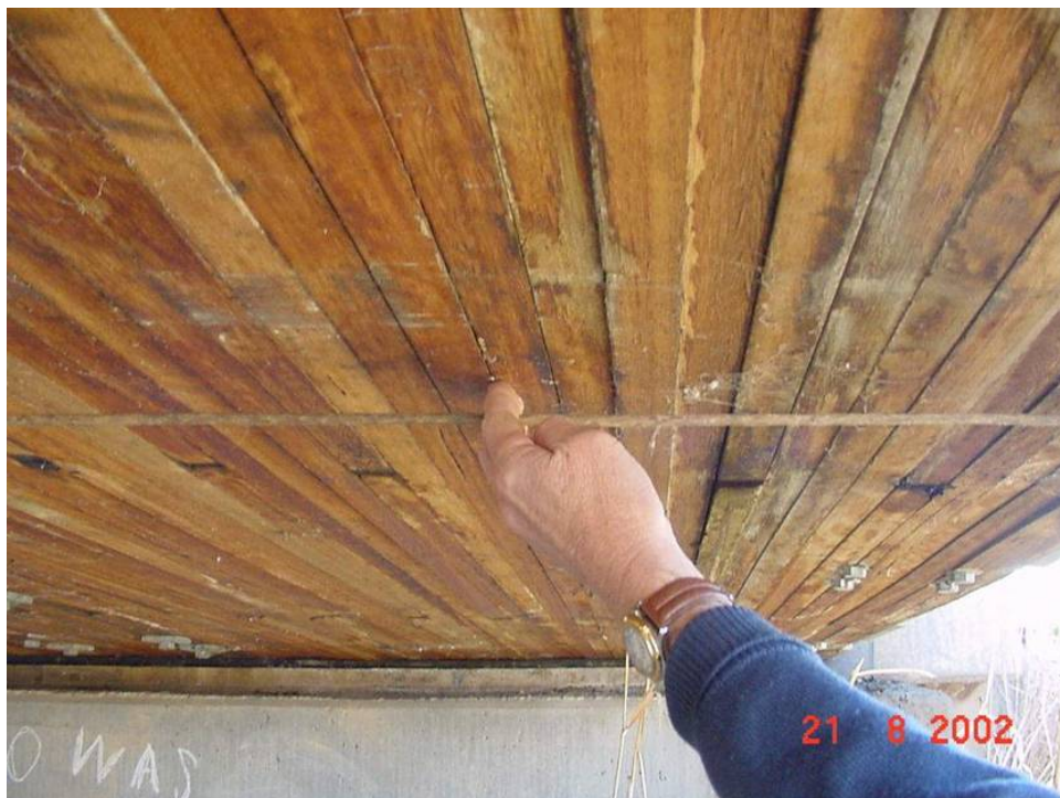
Water seeping through laminates.
