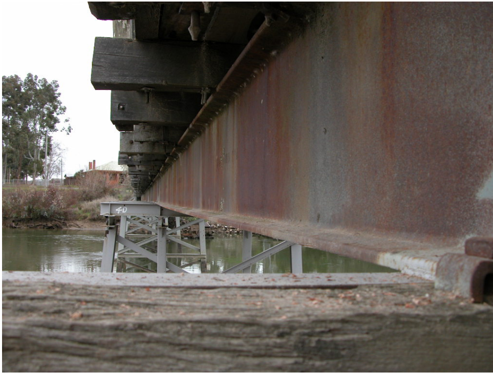
Coating no longer present.
