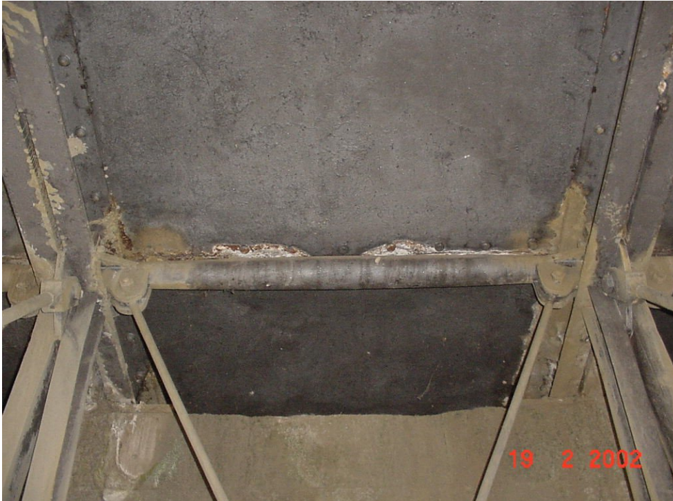
Buckle plate deck with minor leakage and corrosion at the edges.
