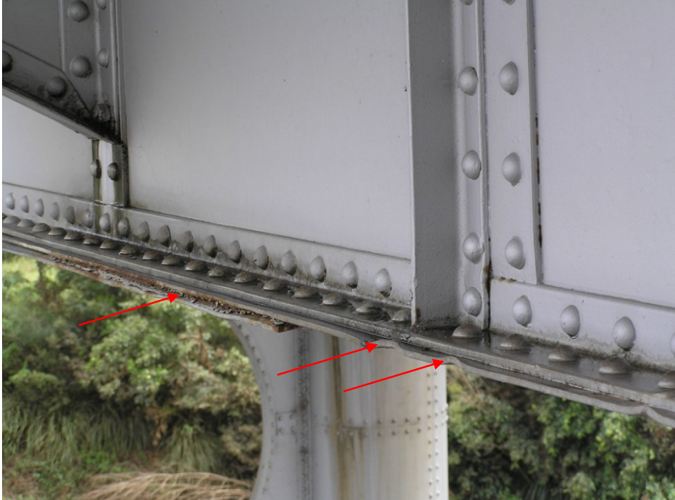
Crevice corrosion at splice plate on underside of girder. Some minor mechanical impact damage also evident.
