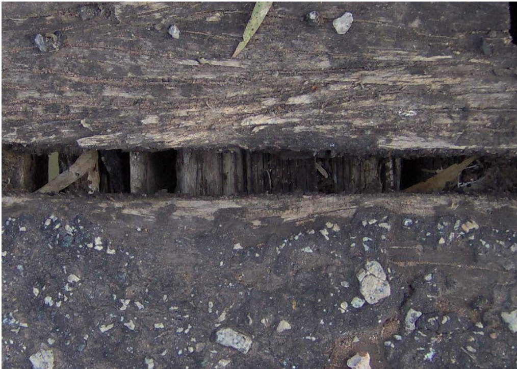
Advanced deterioration of transverse decking.
