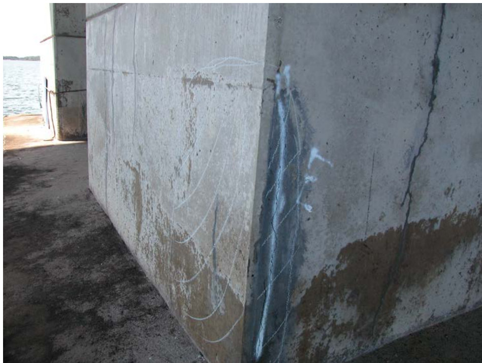
Patched up crack reopening
