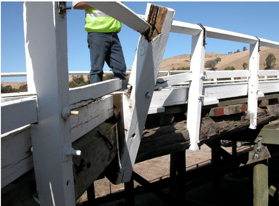
Timber railing requiring immediate repair.
