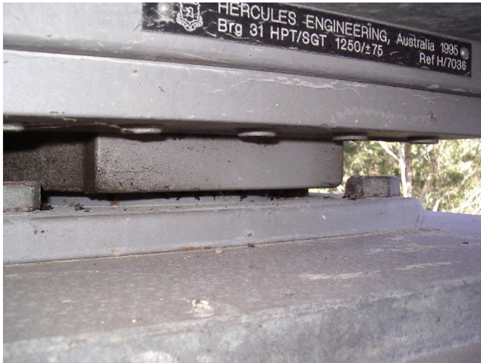
Minor leakage of rubber.
