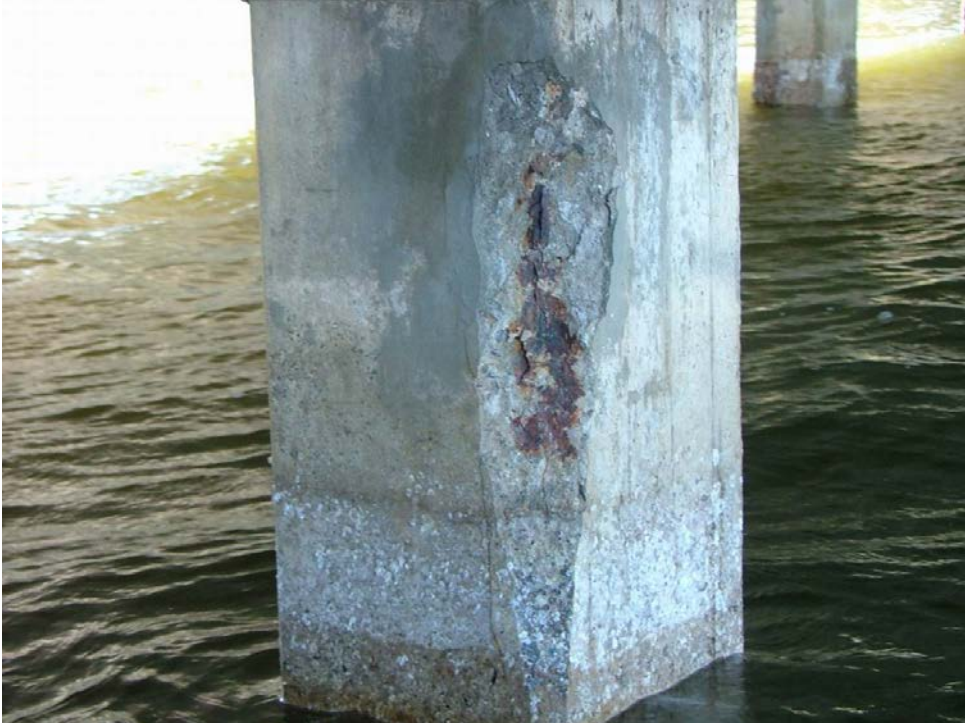
Significant spall with corroding reinforcement.
