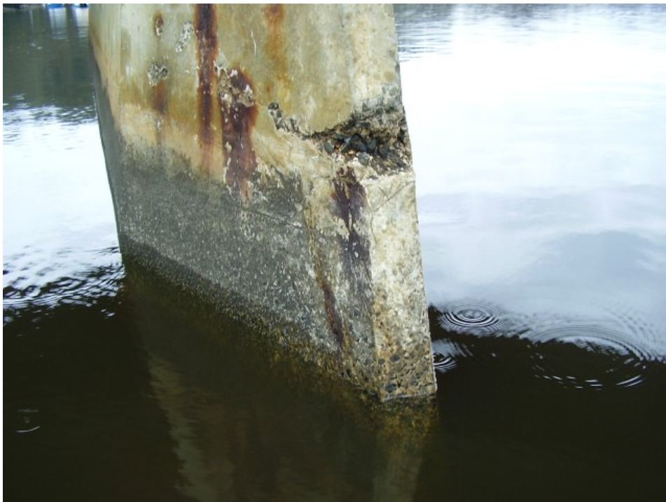
Some spalls and signs of corrosion of reinforcement.
