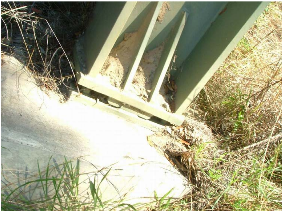
Dirt accumulation inside structural element.
