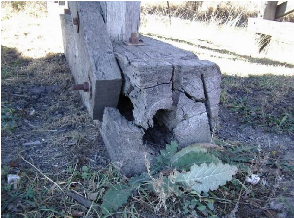
Badly rotten sill beam.
