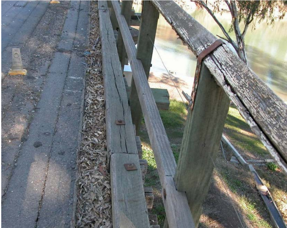
Timber railing and kerb with significant splits.
