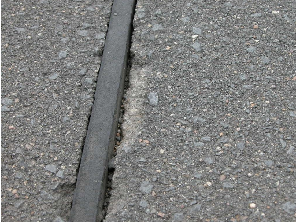
Joint with minor spalls not showing any major leakage under the bridge.
