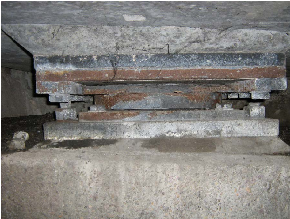
Enclosed bearing with surface corrosion.
