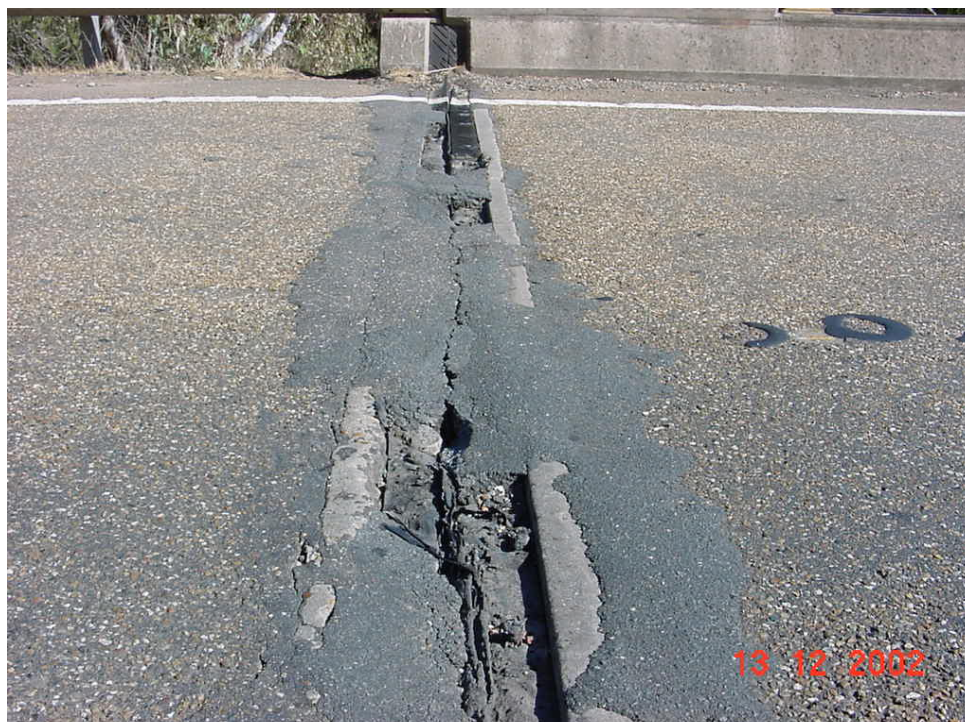
Joint in poor condition.
