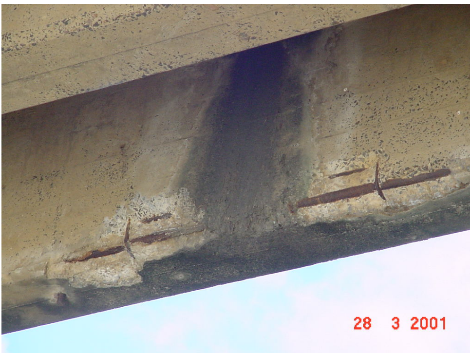
Bottom edge spalled. Exposed and corroding reinforcement with no significant loss of section.
