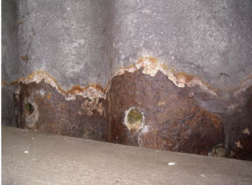
Significant corrosion with missing bolts.
