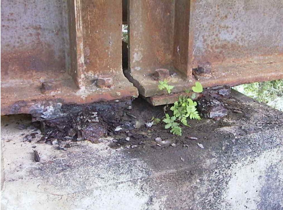
Advanced corrosion of the base plate.
