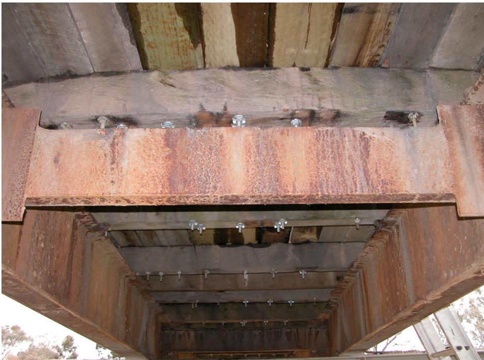
Coating no longer present.
