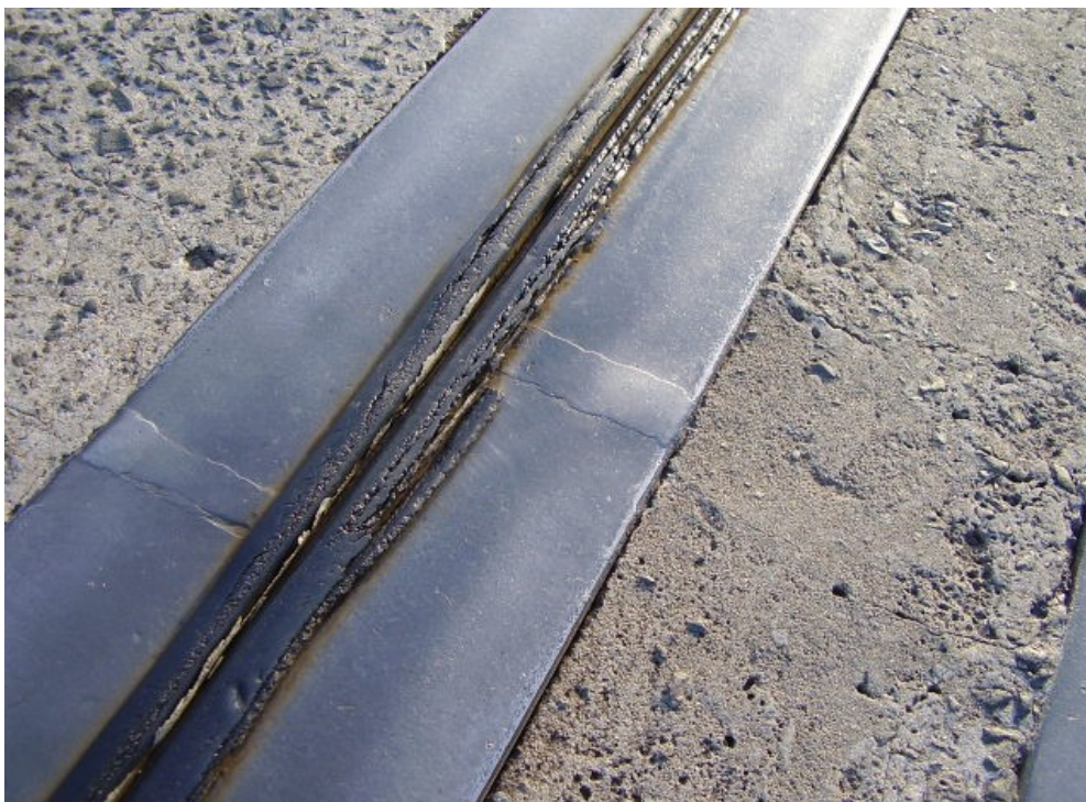
Moderate deterioration of the seal.
