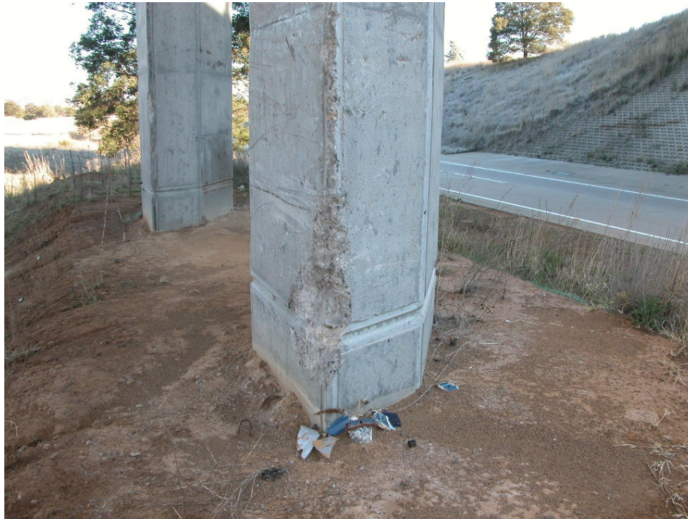
Accident damage - Concrete chipped off the pier column
