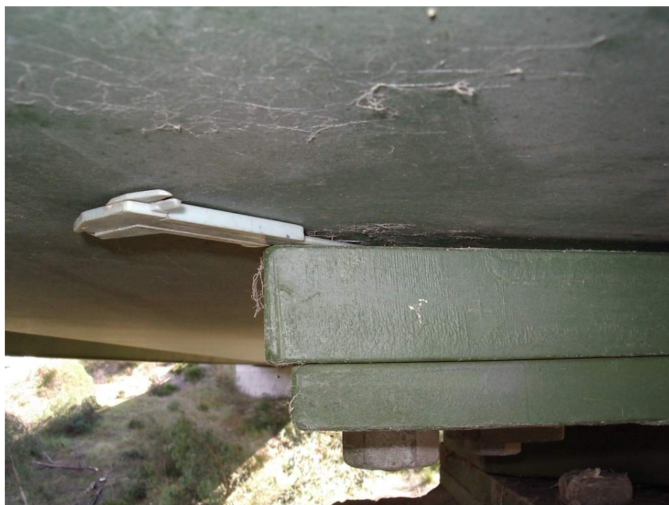
Excessive gap at the concrete bearing interface indicating rotational limits of the bearings may have been reached.
