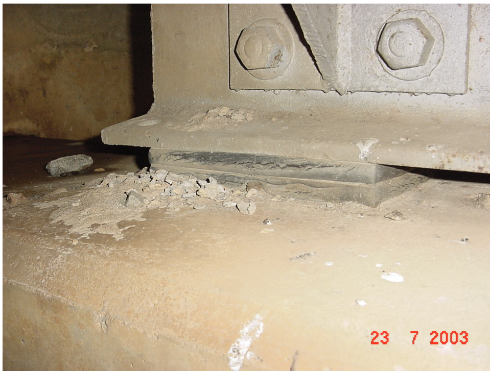
Significant splitting and bulging of bearing pads.
