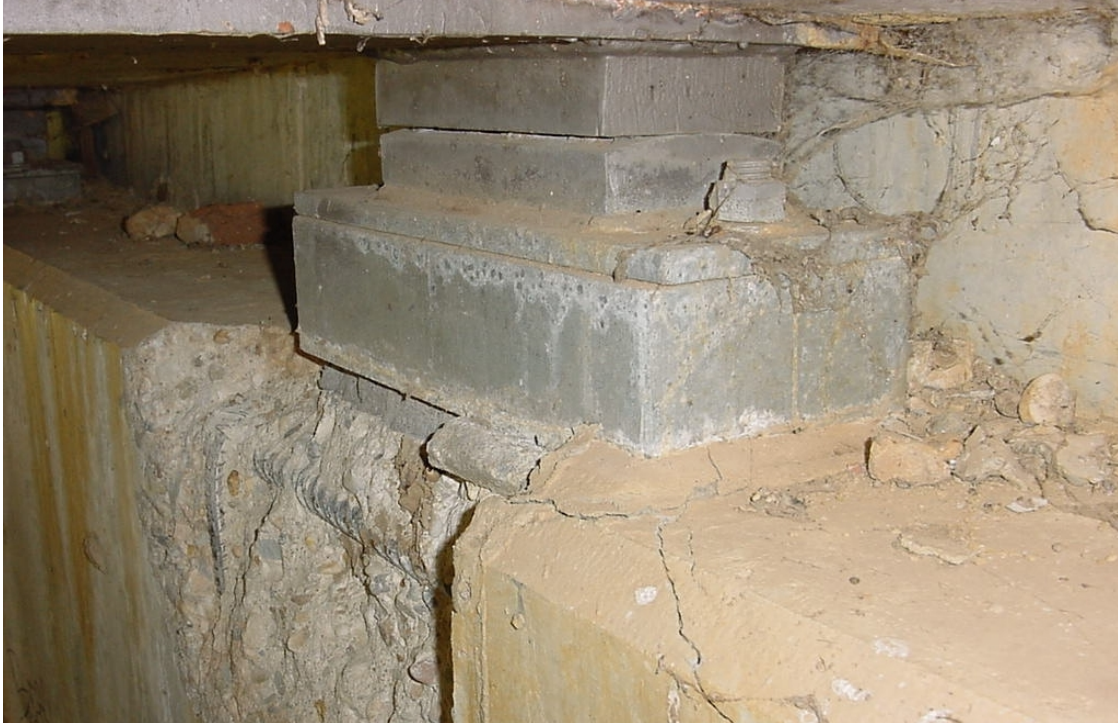
Major spall near the bearing with exposed reinforcement.
