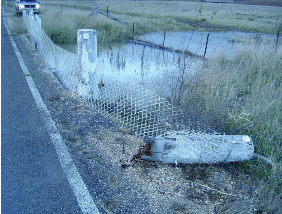
Miscellaneous railing with broken timber post,
