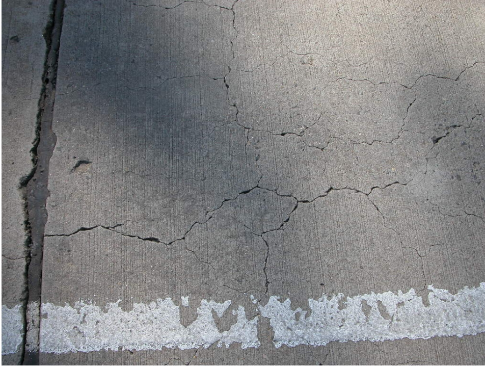
Cracked deck slab.
