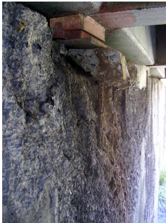
Local failure of the headstock under the bearing threatening support of the beam. Reinforcement and holding bolt exposed
