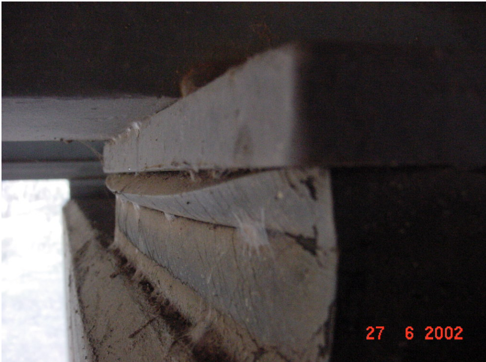
Significant bulging of bearing pad.
