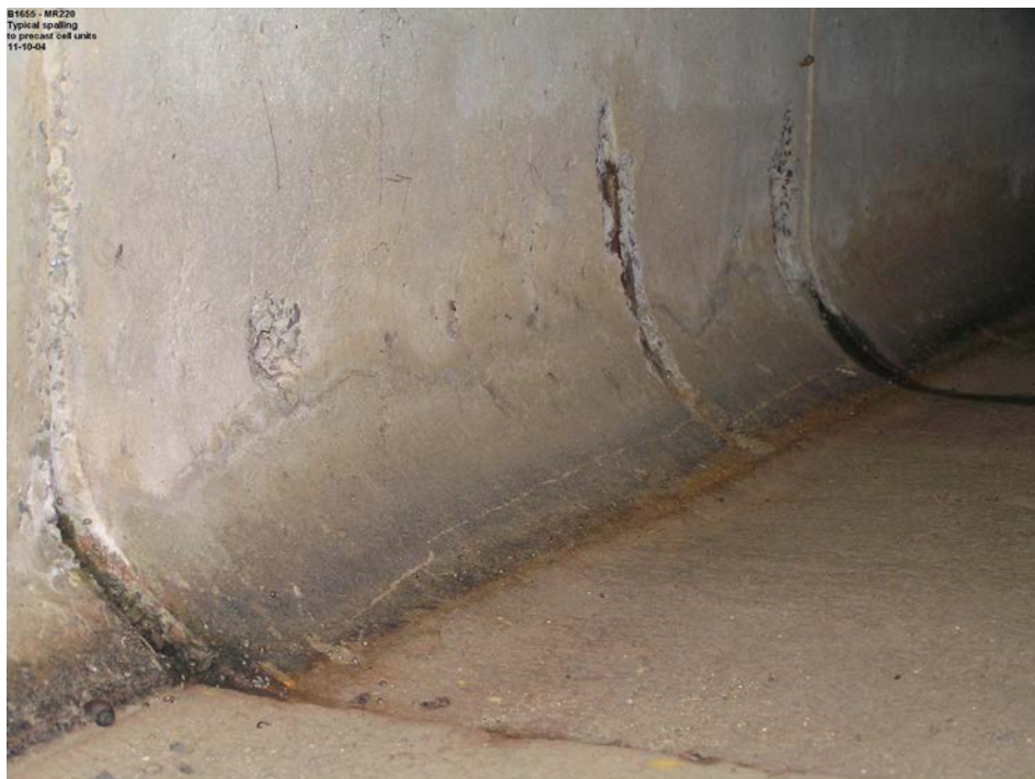
Spalls on the wall.
