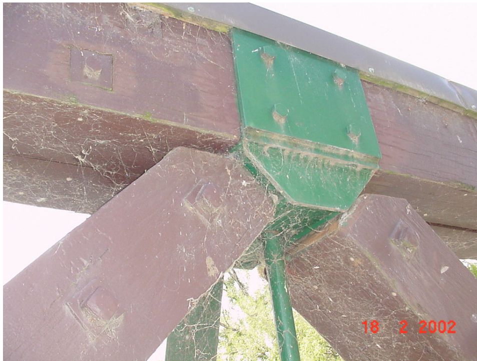
Timber strut in good condition has partially slipped off the joint. The movement is significant to affect the serviceability of truss.
