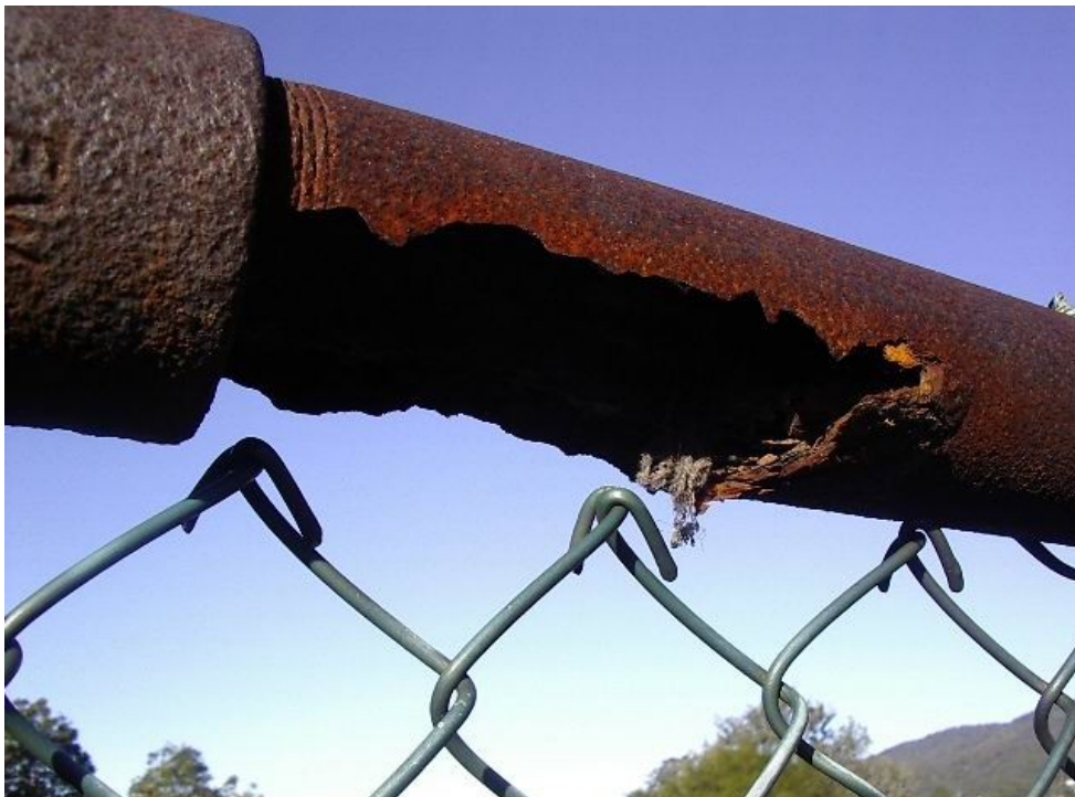
Badly corroded steel tube rail.
