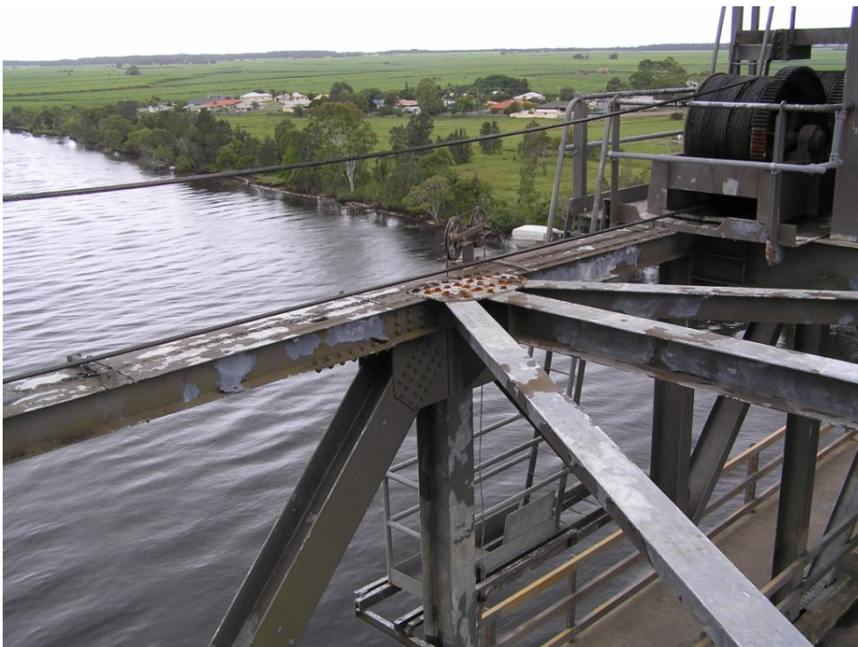
Surface rusting on rivets.
