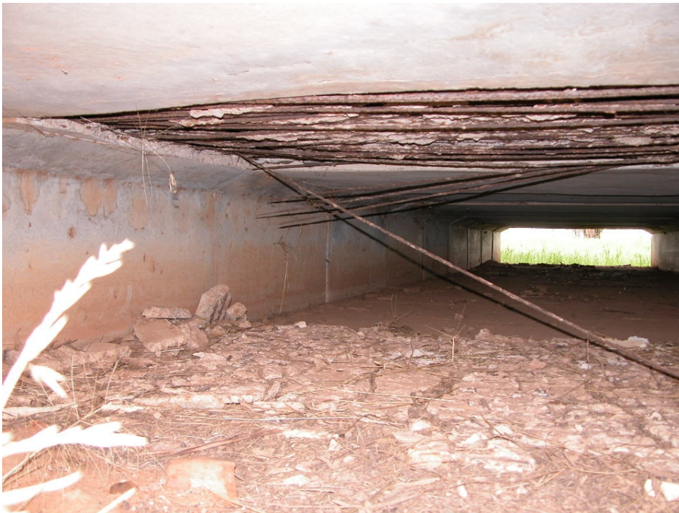
Extreme delamination and with falling off roof reinforcements of precast units.
