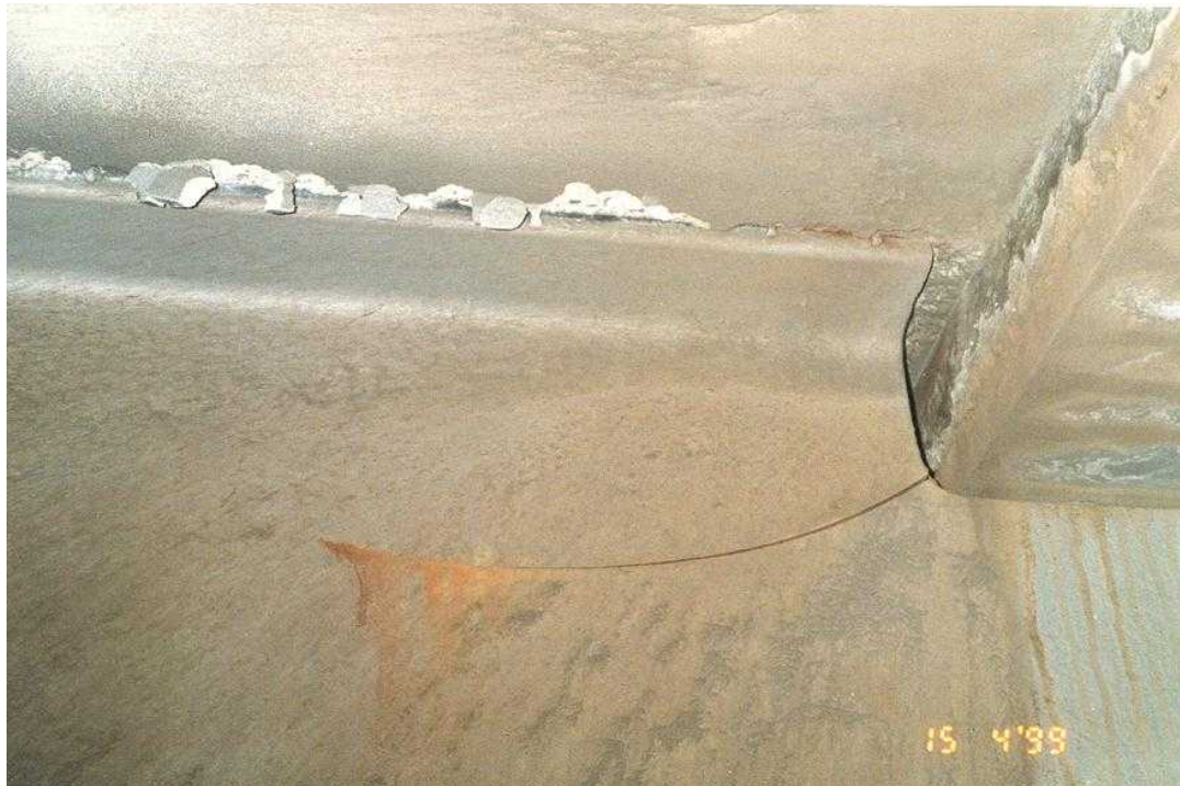
Fatigue crack in stringer.
