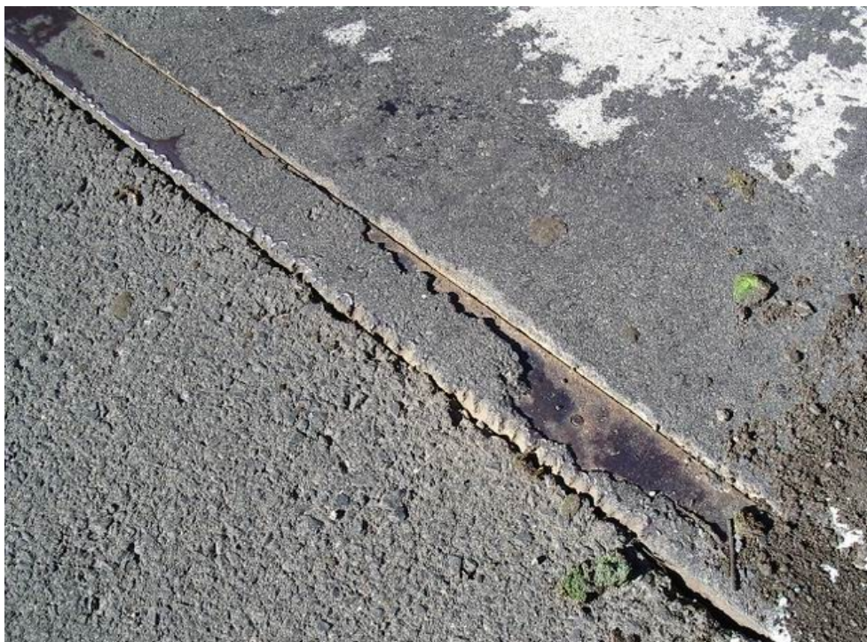
Protection angle is loose and noisy.
