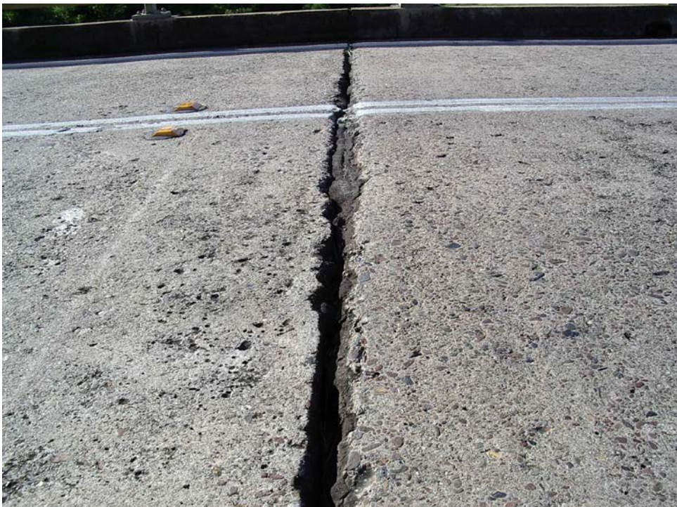
Seal has failed leading to extensive water leakage through the joint.
