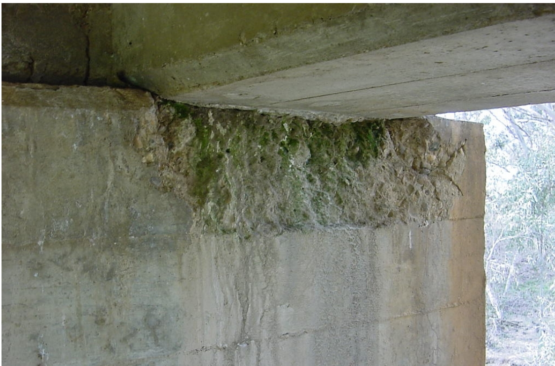
Significant spall under the beam on the headstock.
