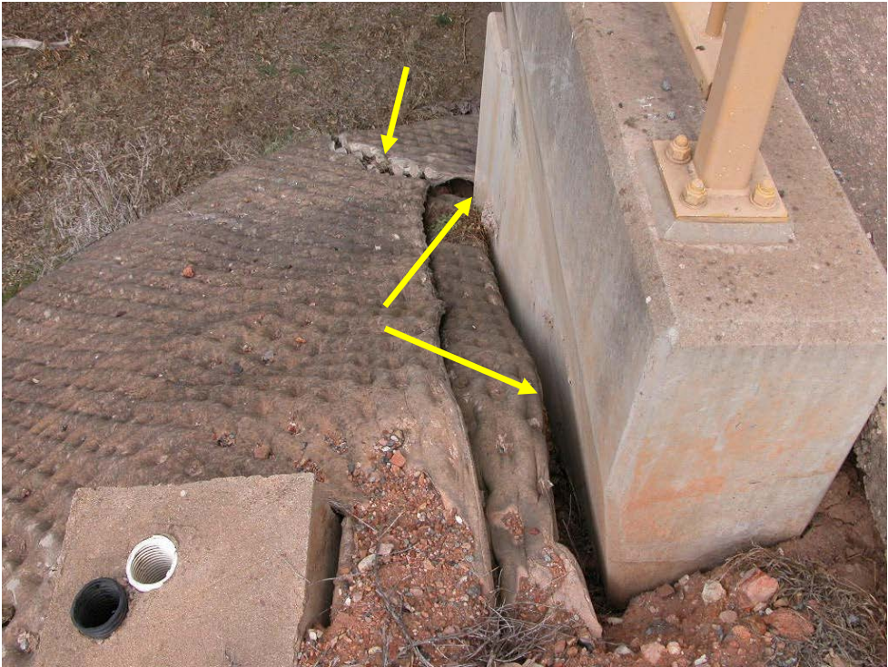
Cracked fabric protection and gaps allowing water to run under and erode the base
