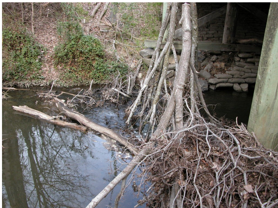
Waterway with some scour and debris buildup.
