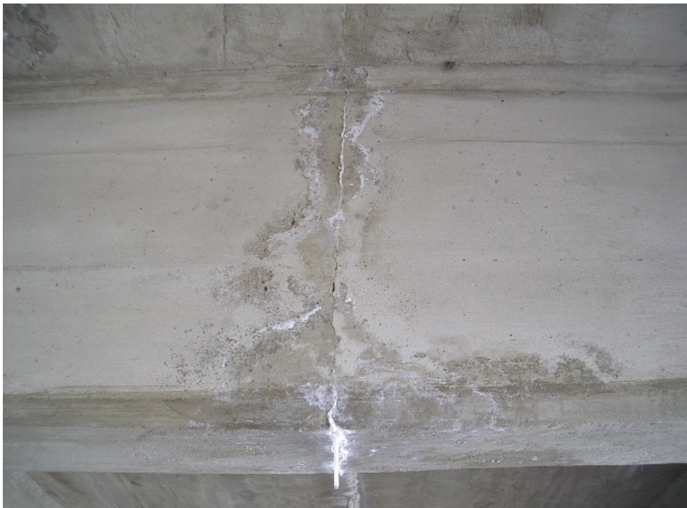
Significant moisture ingress and leaching at the construction joint of the cross girder. No evidence of corrosion.
