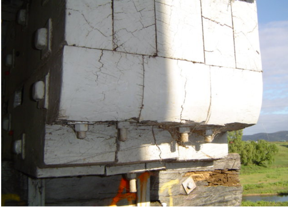
Minor splits on the members of the butting block.
