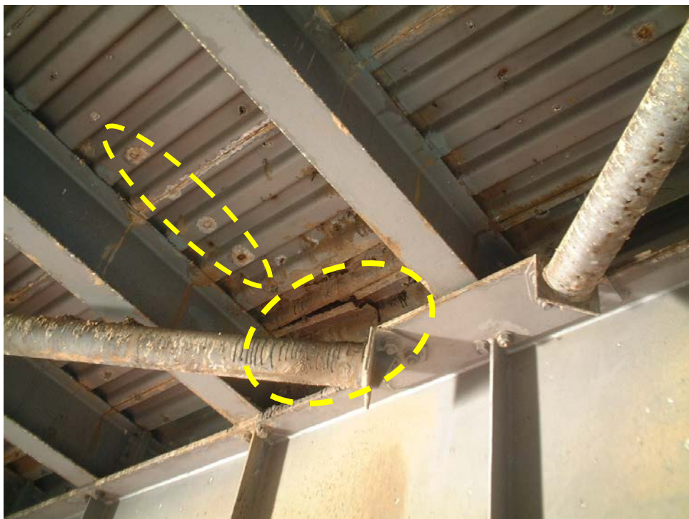
Failed connectors and localised failure of decking.
