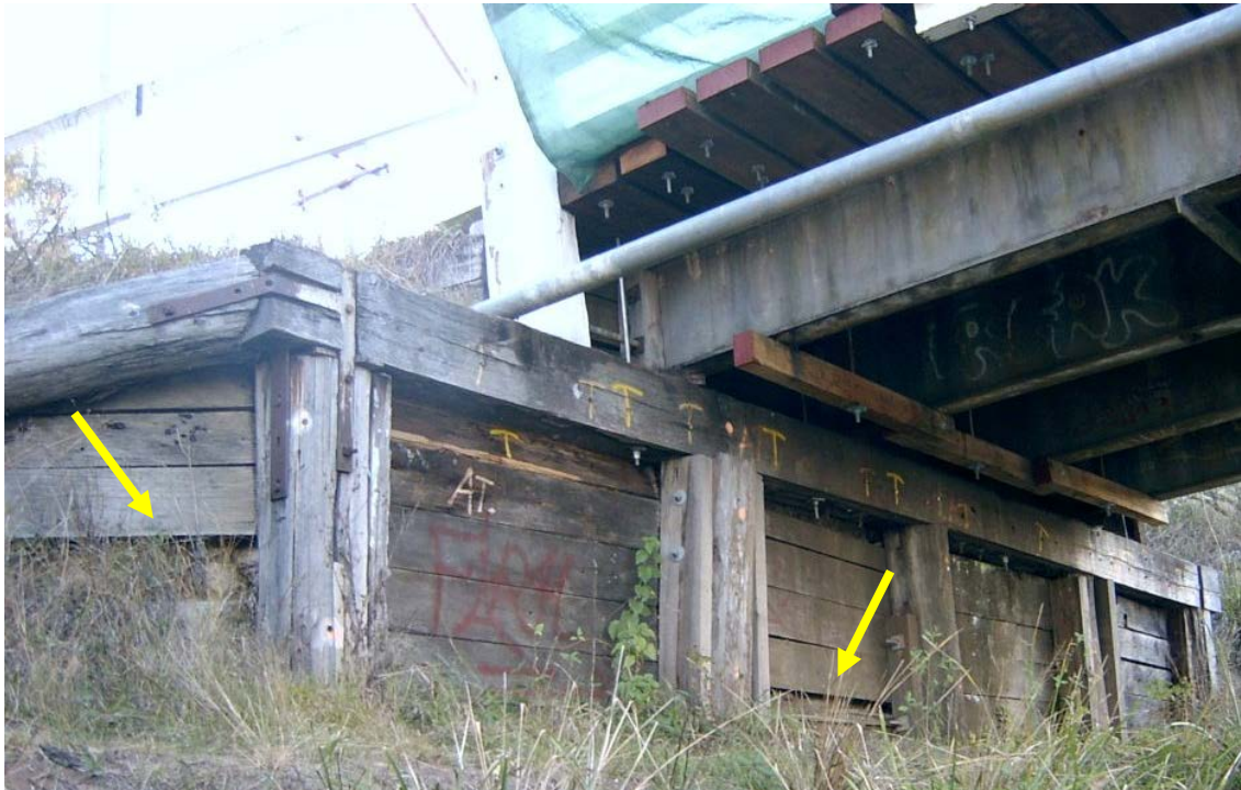
Abutment sheeting with termite infestation and some rotten boards.
