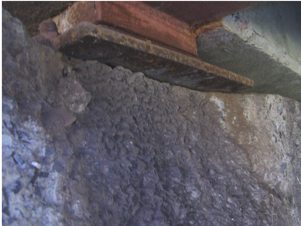
Significant spall under the bearing on the headstock. No exposed reinforcement in the headstock.
