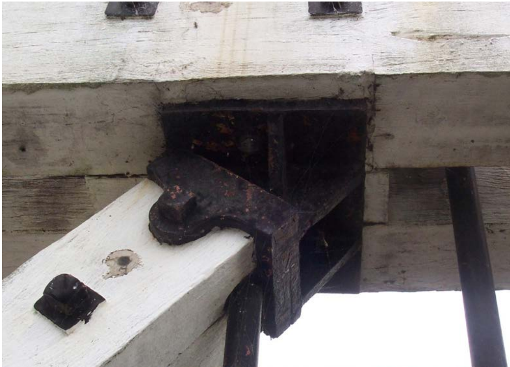
Shoe showing surface rust and minor pitting.
