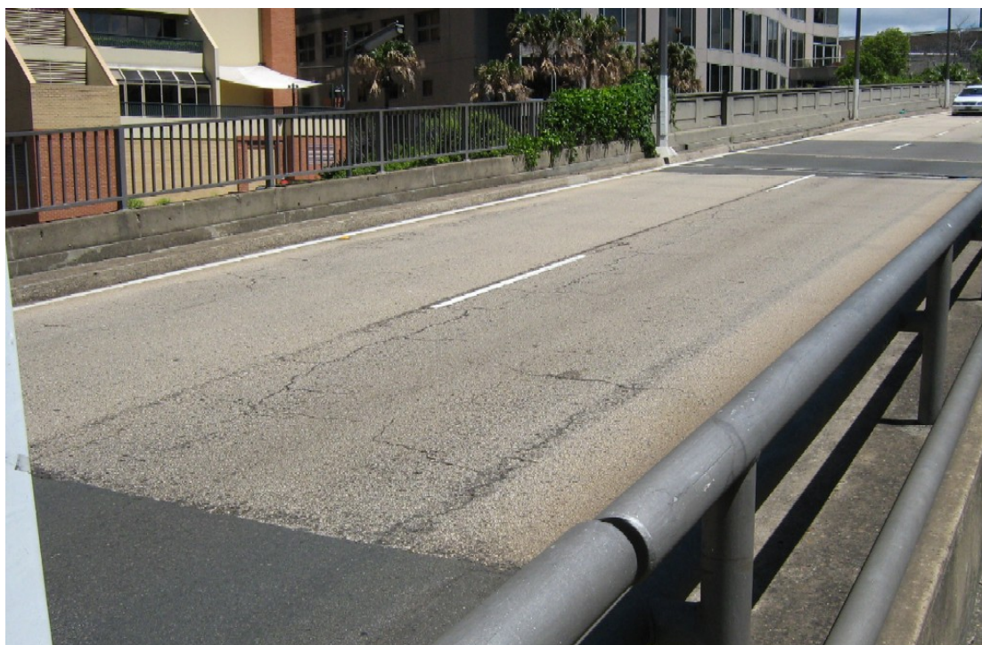
Cracking of large areas of the wearing surface on the bridge.
