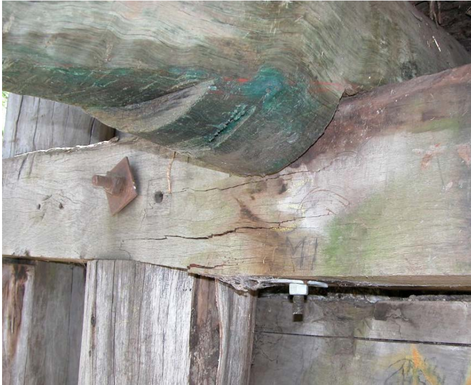
Timber headstock with significant crack under the girder.
