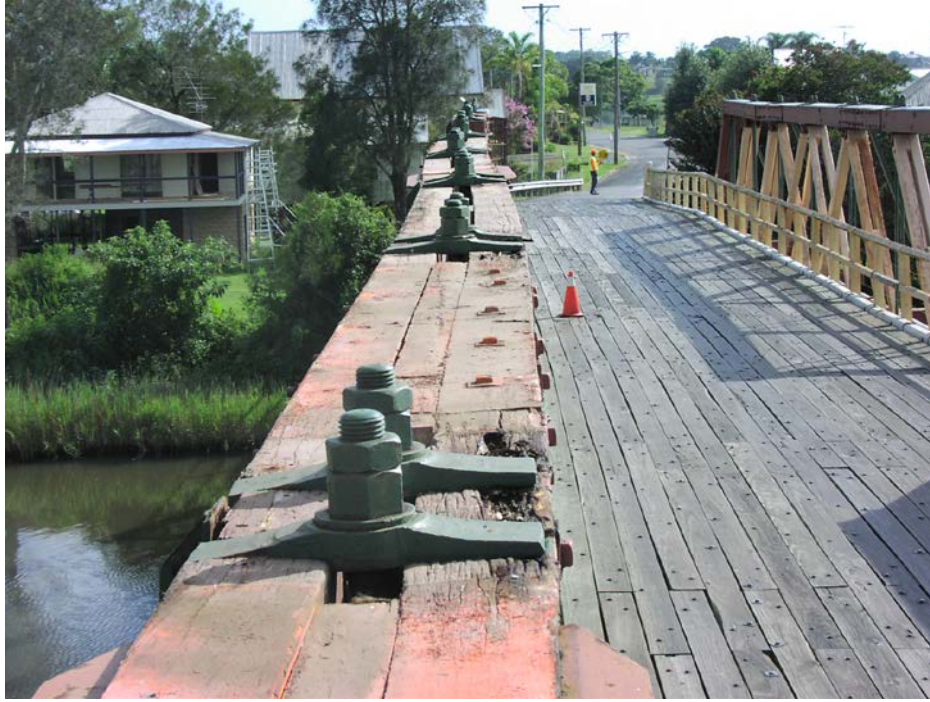
Significant out of alignment of the top chord with major decay.
