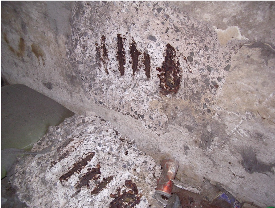
Major delamination - corrosion of reinforcement.
