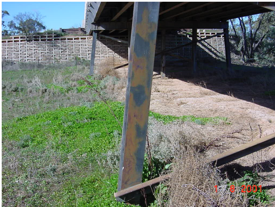
Uniform surface rusting on pile.
