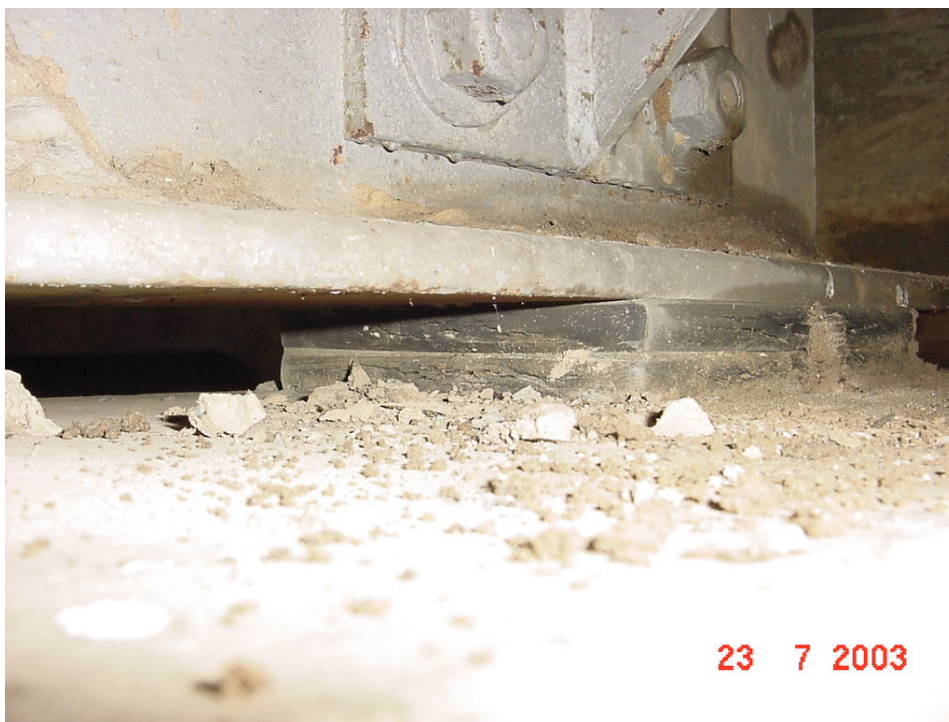
Significant splitting and bulging of bearing pads.
