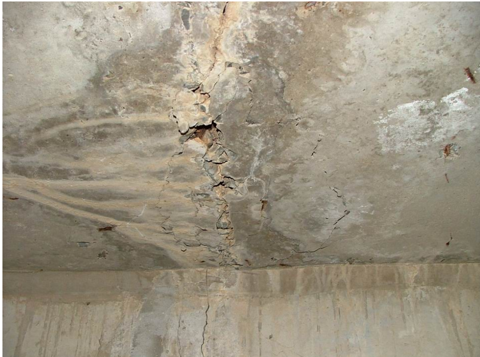
Cracking, leaching and spalling around an area of poor concrete in the roof.
