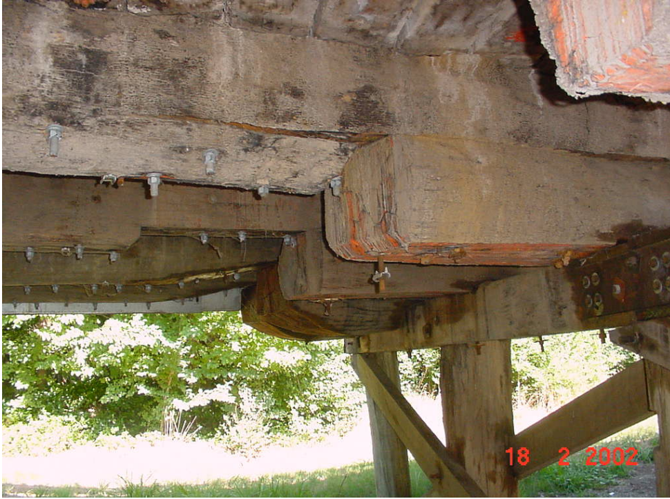
Minor split on the girder.
