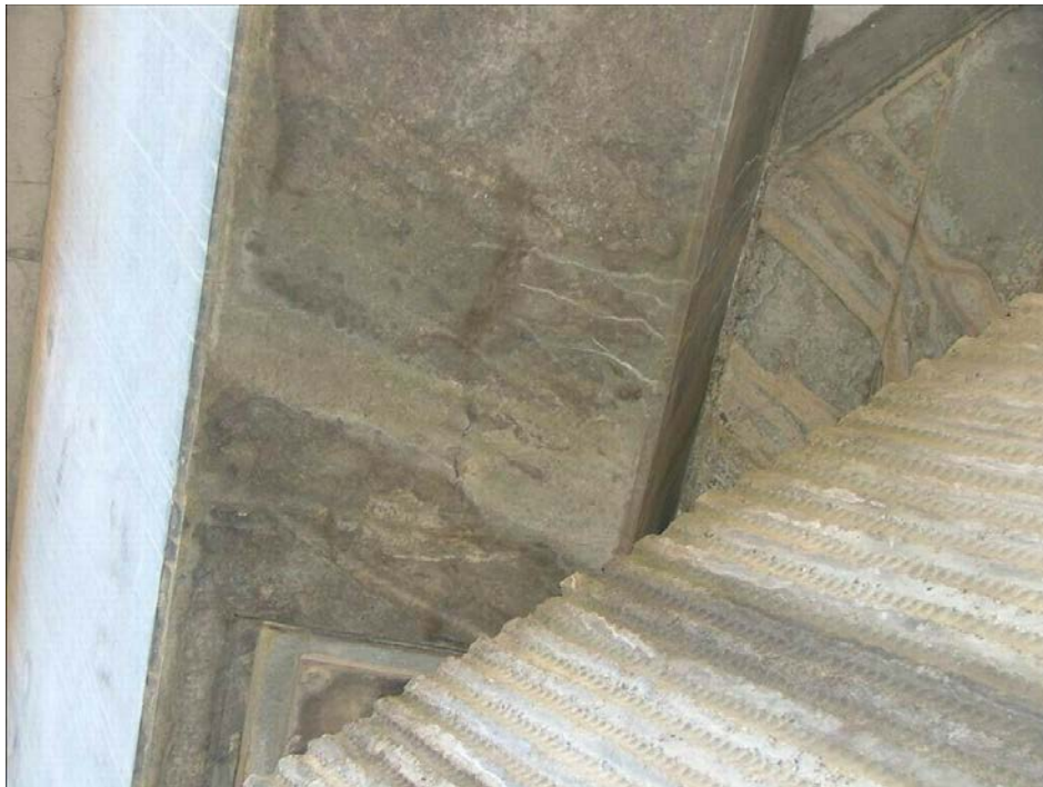
Short cracks and leaching on the soffit of prestressed trough girder
