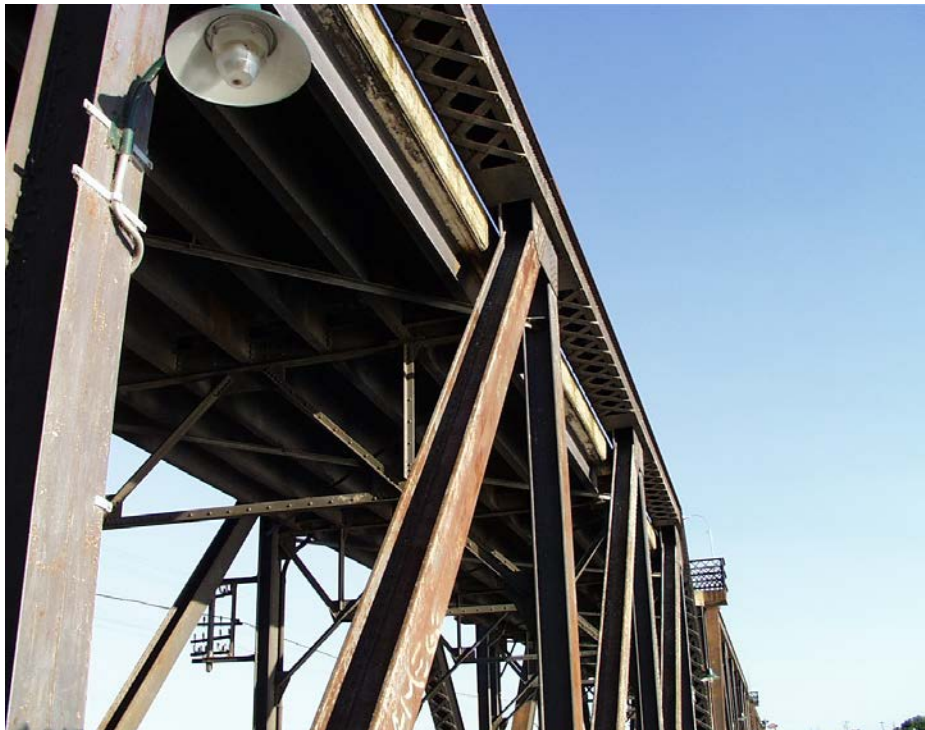
Uniform surface rust on diagonal.
