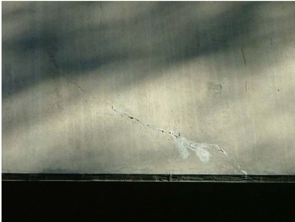
Diagonal cracking near pier 1, crack extending to the soffit.
