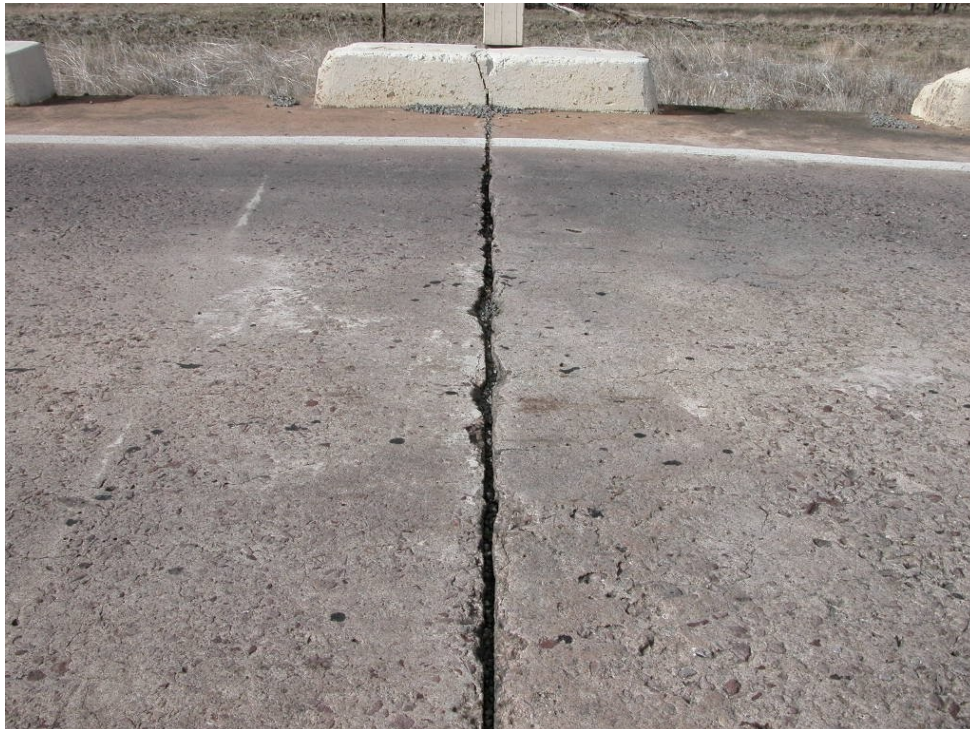
Joint blocked with debris. Minor spalls at joint edges.
