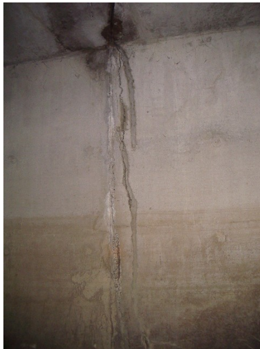
Vertical crack near the construction joint on the wall. noticeable leaching.
