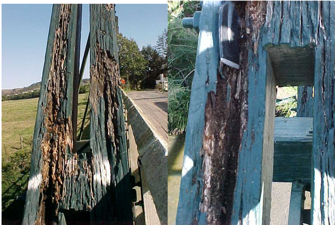
Advanced decay of principals
