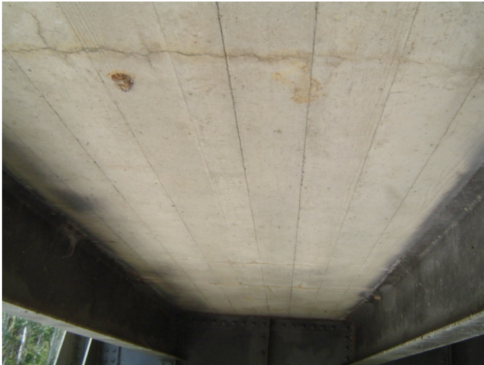
Transverse cracking of deck slab with minor leaching.
