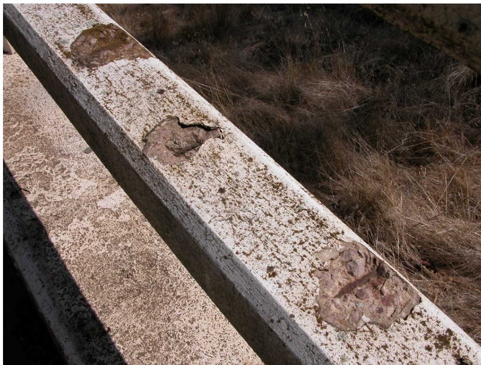
Spalls and exposed reinforcements.
