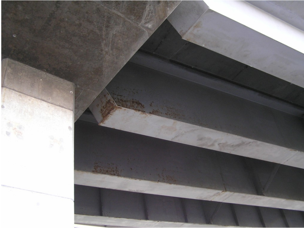
Localised breakdown at end of girder.
