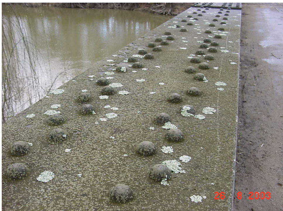
Deterioration of entire topcoat.
