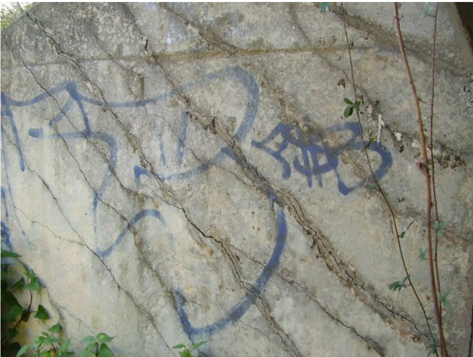
Heavy diagonal cracking of inlet wingwall.
