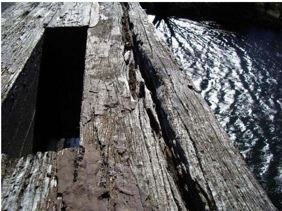
Badly split and rotting top chord.
