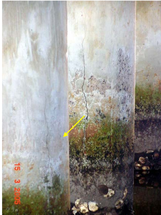
Wide vertical cracks with some signs of corrosion.
