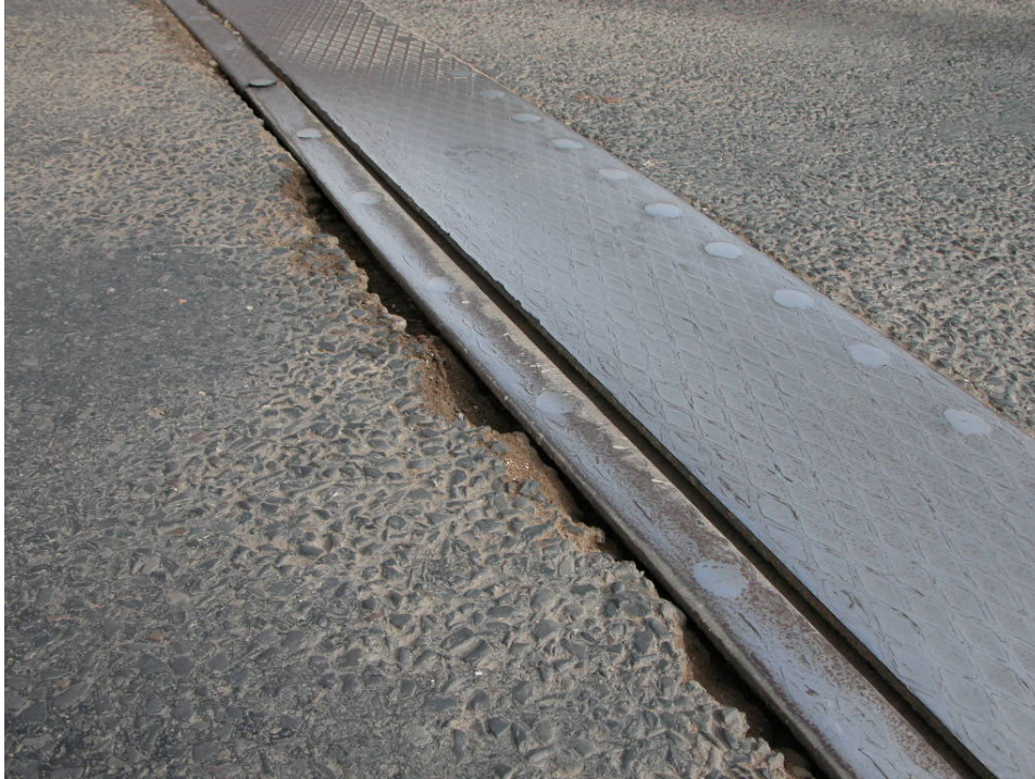
Significant spalling of concrete adjacent to the joint.
