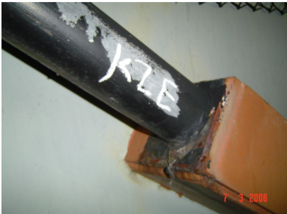
Minor surface corrosion on cable anchorage block in a pedestrian bridge.
