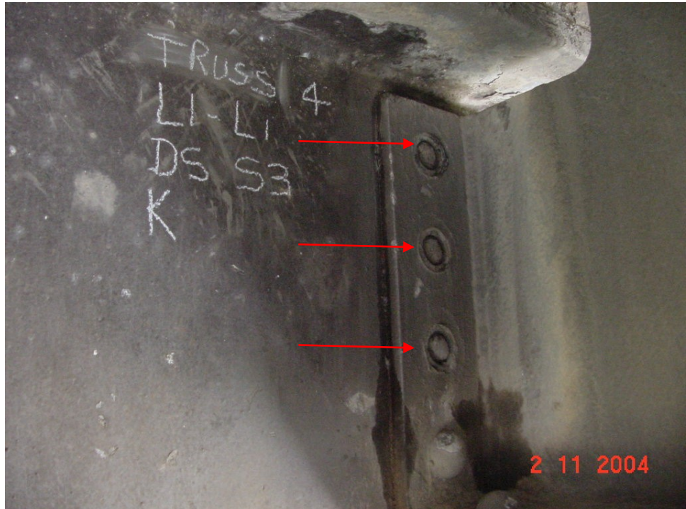
Failed rivets at connection with cross girder.
