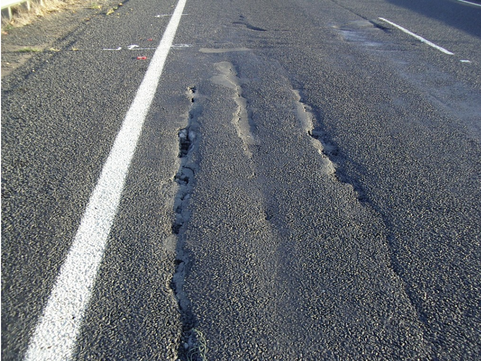
Wearing surface with extensive damage.
