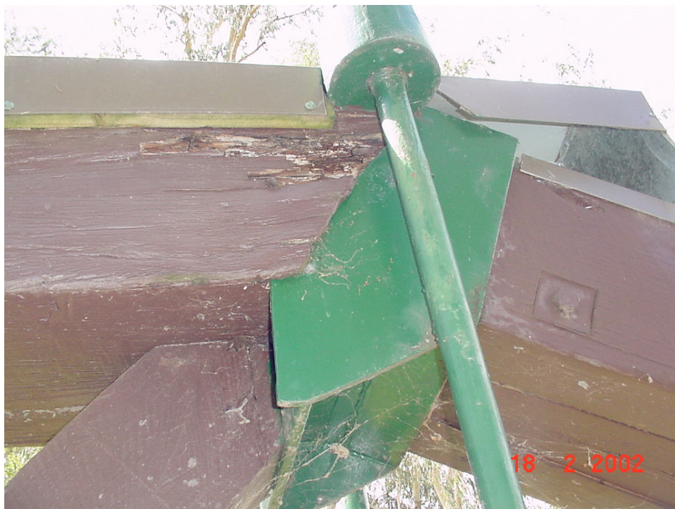
Significant crushing of the top chord.
