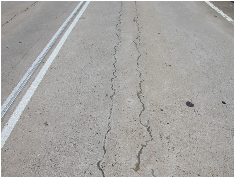
Longitudinal cracks on either side of the road centre line.
