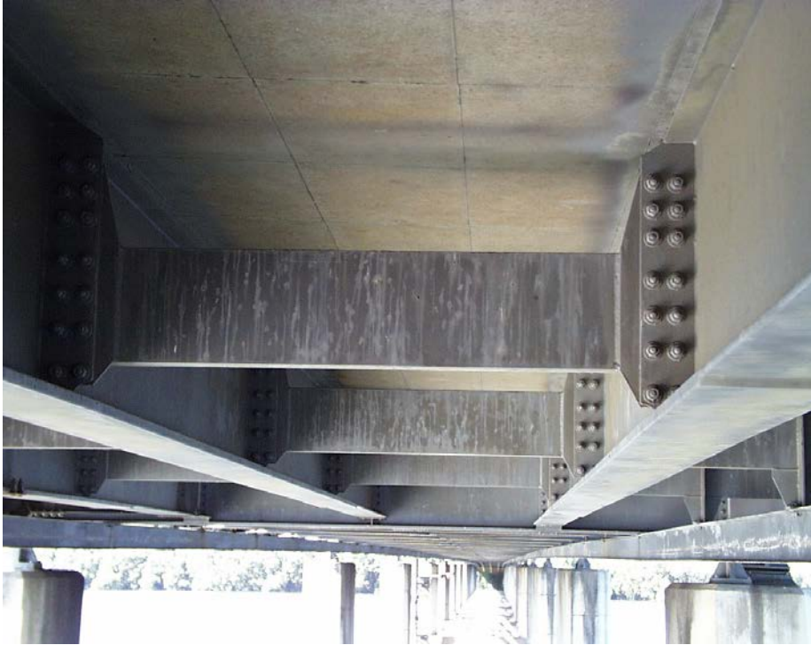
Zinc primer failure on all cross members.
