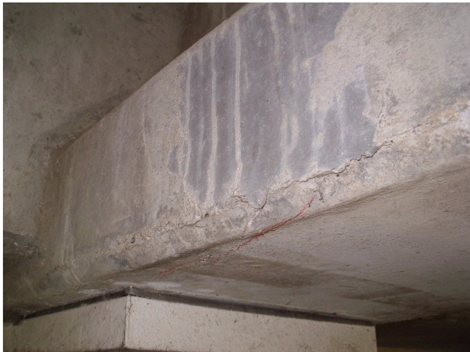
Longitudinal crack along the bottom flange corner near support.
