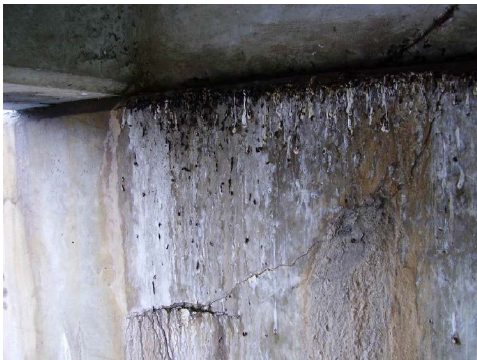
Significant crack with hollow sounding concrete behind the affected area.
