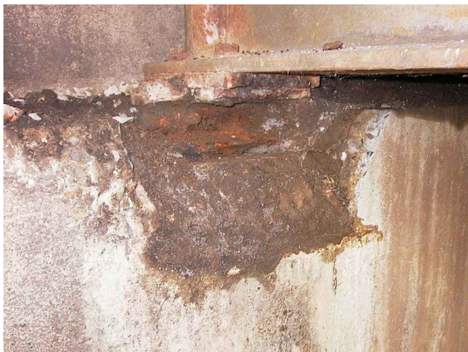
Significant loss of support under the bearing.
