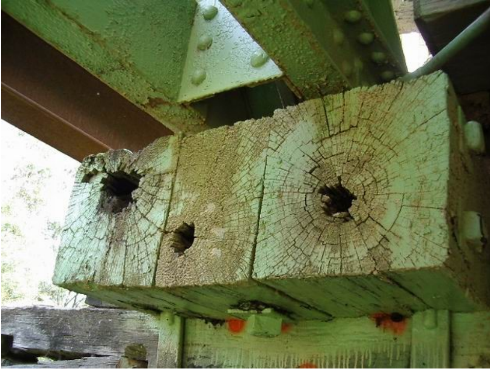
Significant piping in one of the members of the butting block.
