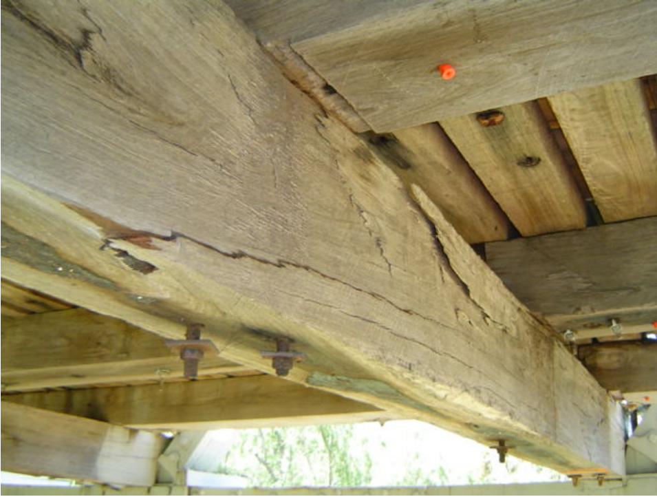
Badly split and cracked cross girder.
