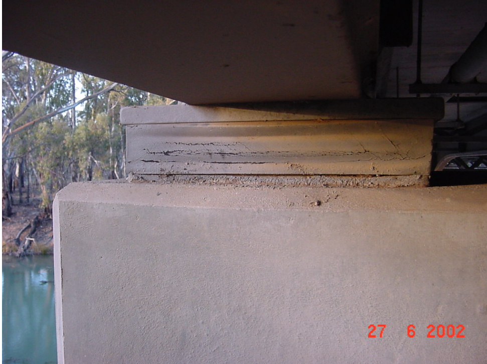
Minor cracking and splitting.
