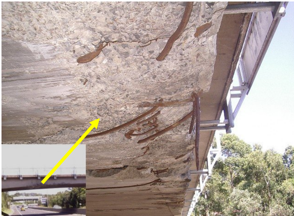
Overheight vehicle impact damage to bottom of prestress girder
