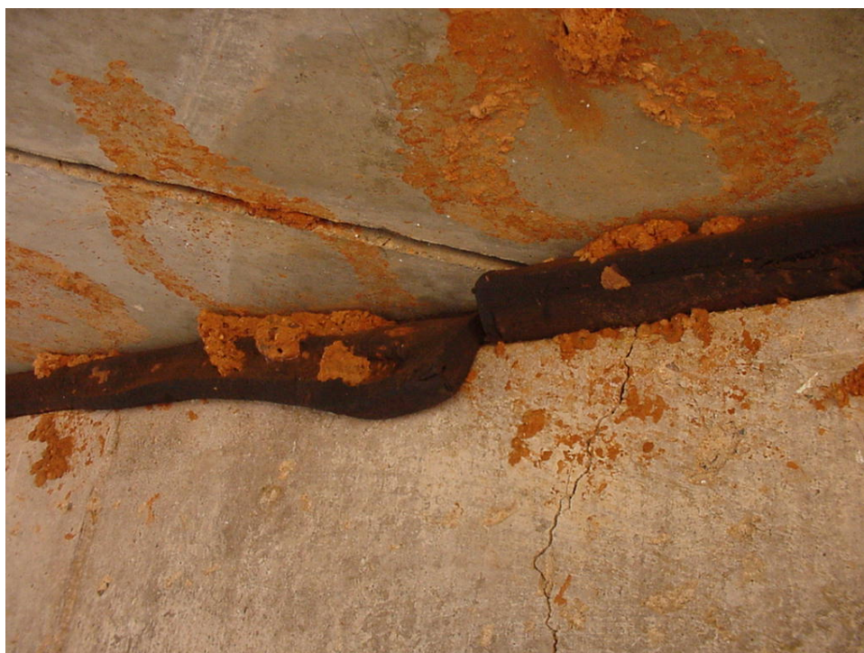
Elastomeric strip bearing slipping out in a skewed PPLNK bridge.
