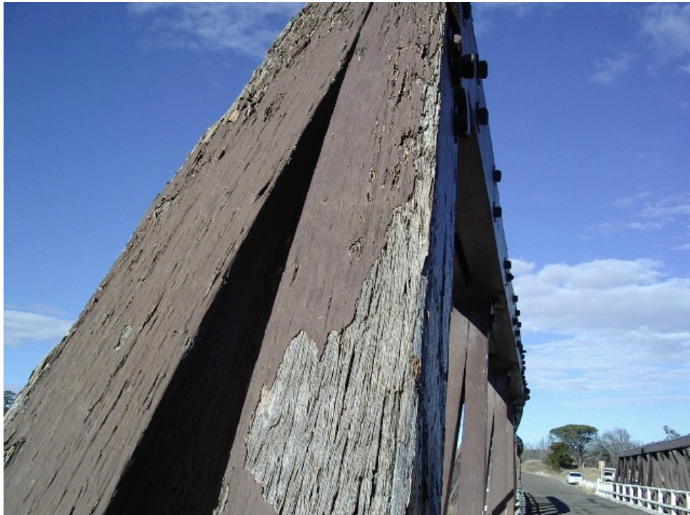
Coating has failed in significant areas.
