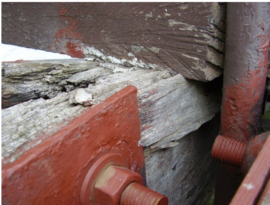
Bottom chord crushing and splitting.
