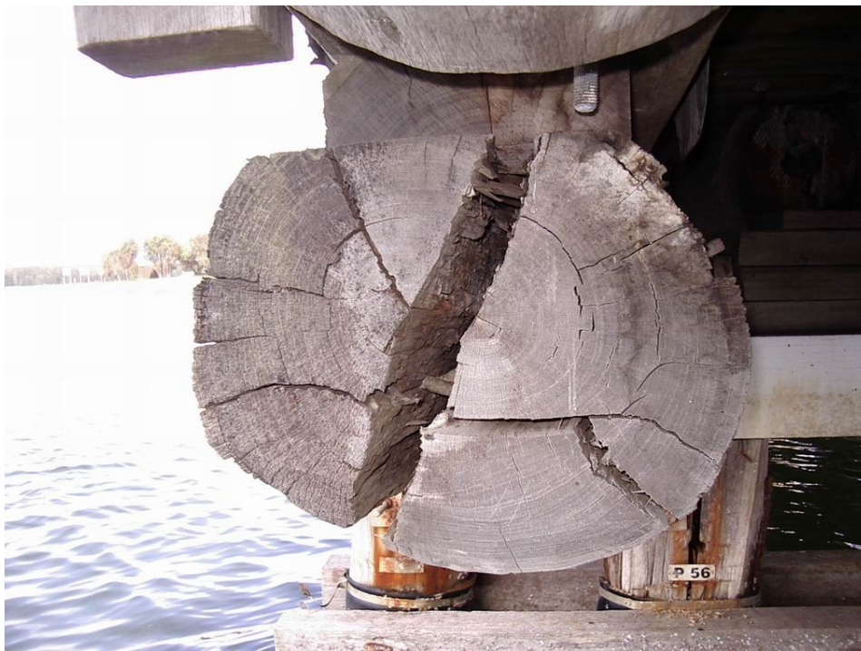
Severely split and splintering corbel
