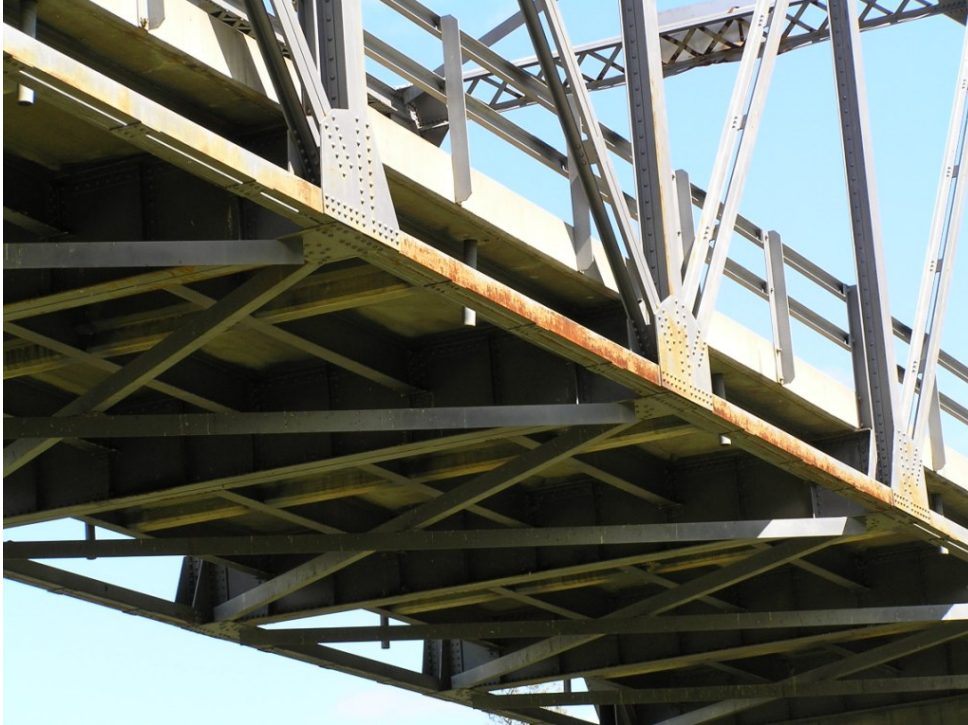
Surface rust on bottom chord.
