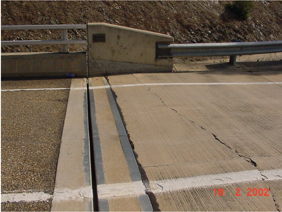
Settlement cracking of approach slab.
