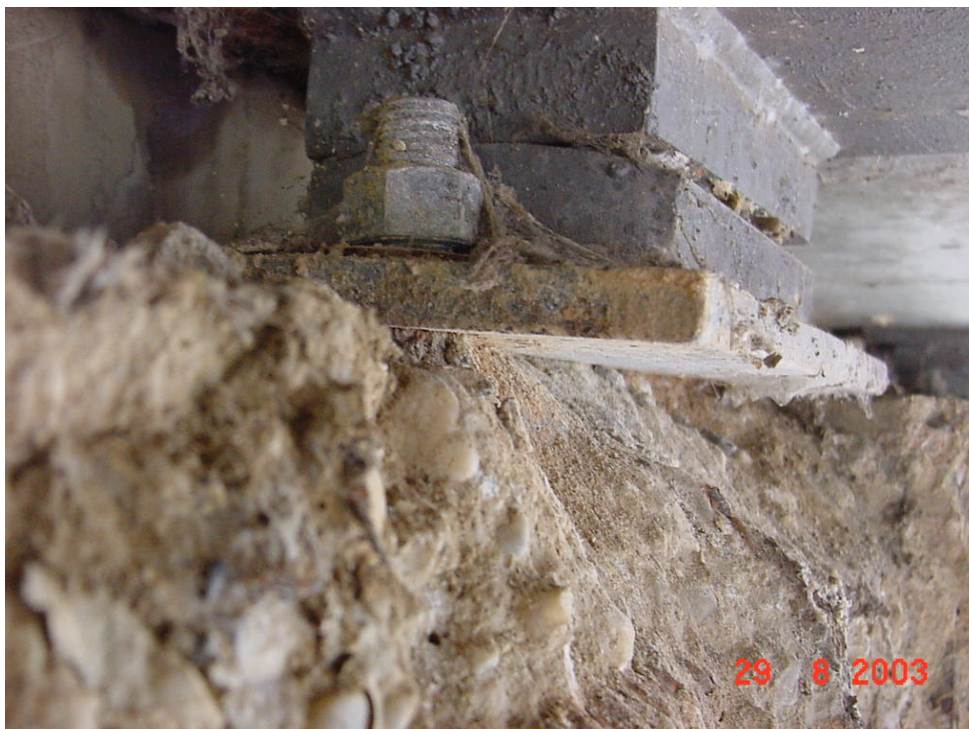
Significant loss of support under the bearing.
