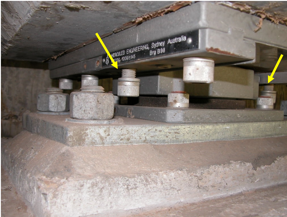
Loose studs on the top plate.
