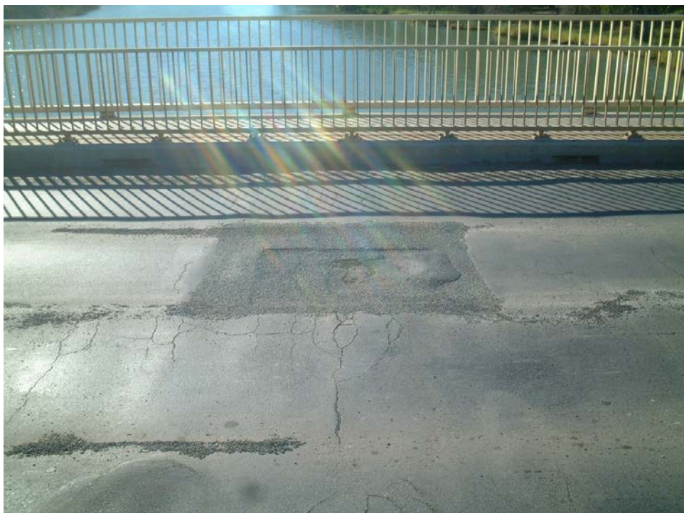
Wearing surface in poor condition.
