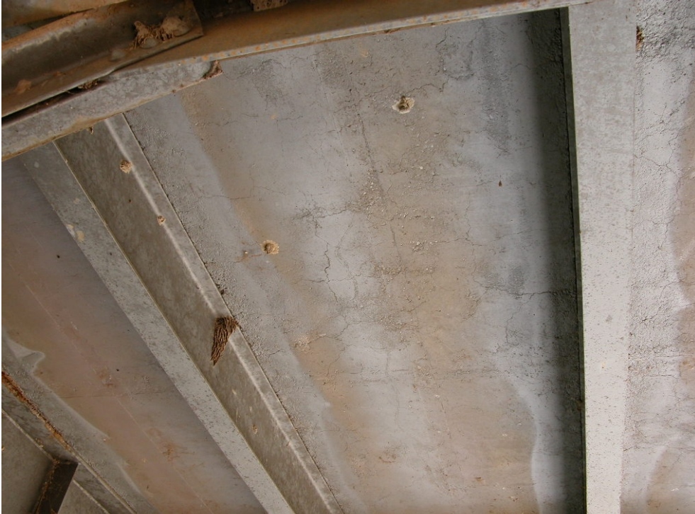
Fine cracks on soffit of deck slab.
