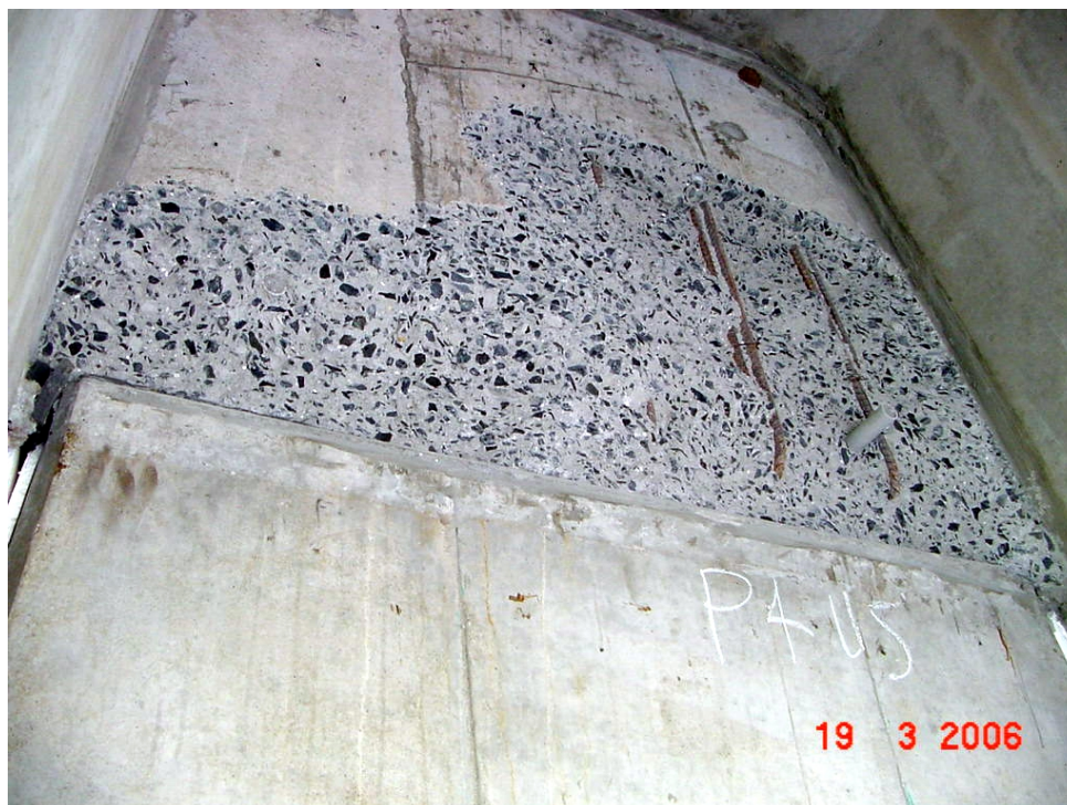
Extensive delamination and exposed reinforcement.
