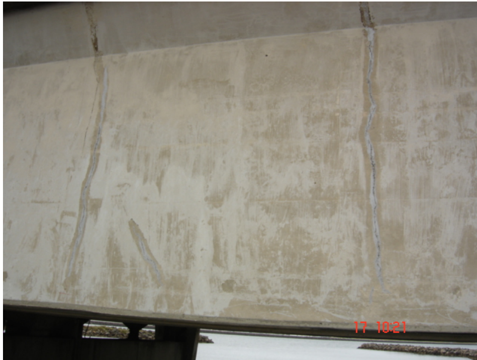
Cracks (previously repaired).
