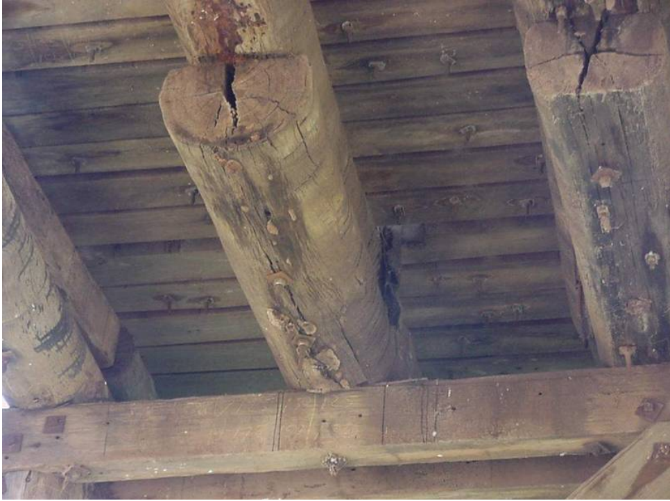
Minor end splits, mainly vertical.
