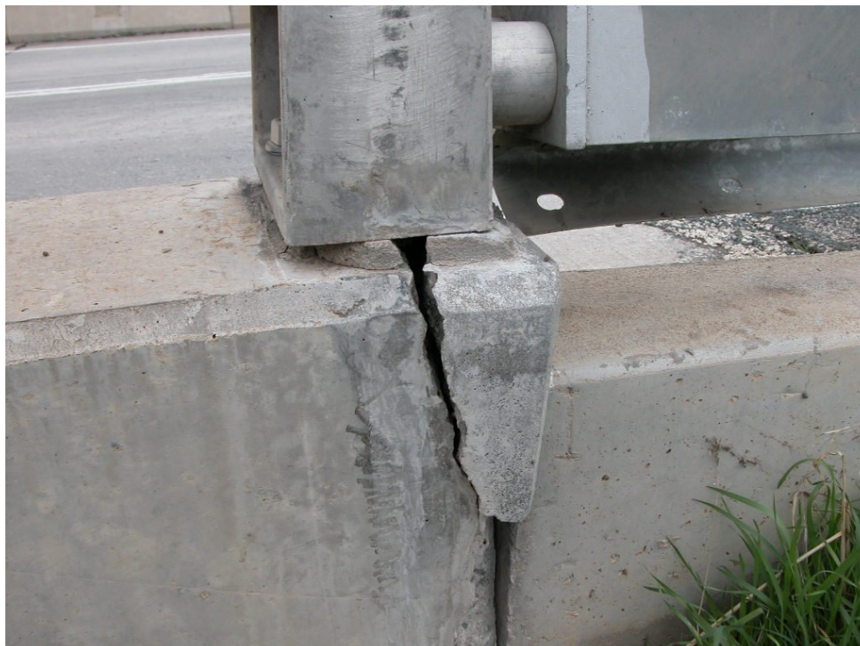
Damage to concrete support requiring repairs.
