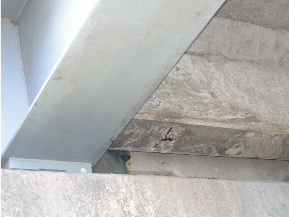
Minor spall with exposed reinforcement in the cross girder
