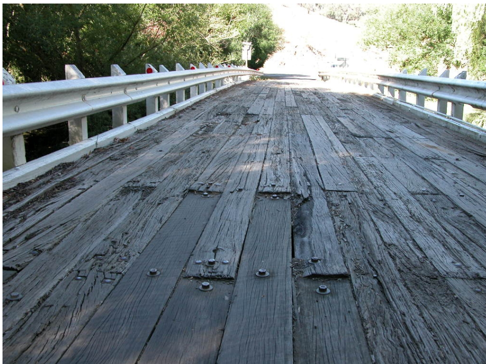
Deck in poor condition with loose bolts and damaged sheetings
