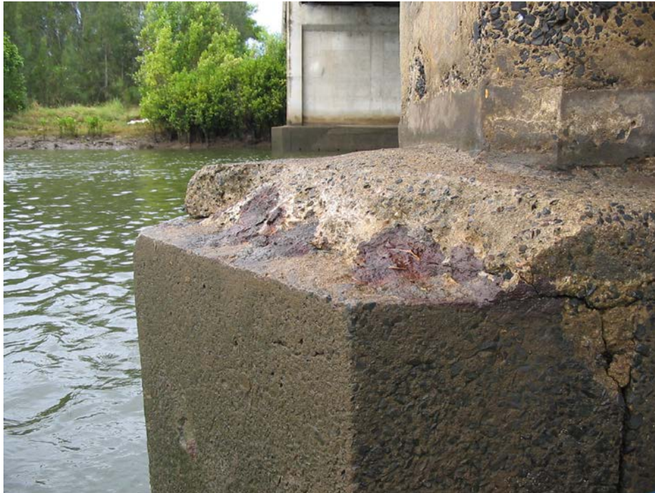
Corroding reinforcement and significant vertical crack on the side.
