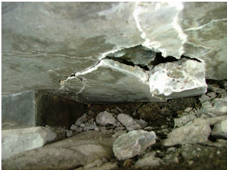
Badly deteriorated end of a prestressed plank girder at an abutment end.
