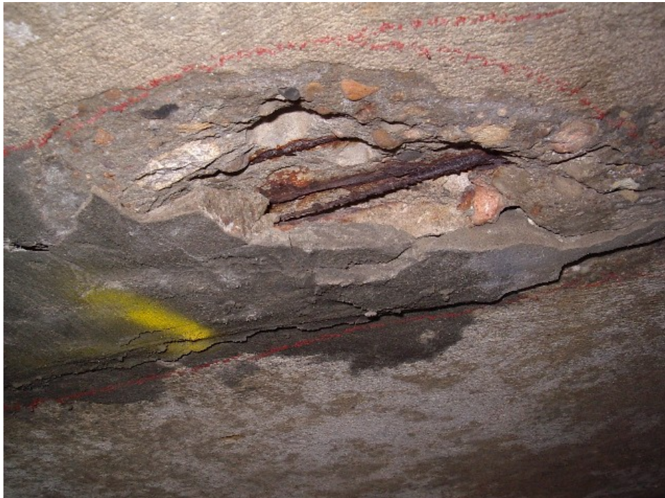
Spalling of a small area of plank soffit with exposed and corroding prestressing strands.
