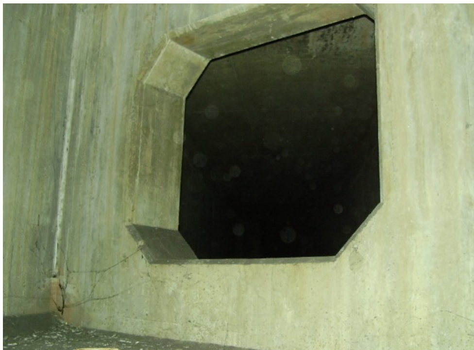
Cracked diaphragm with access hole.
