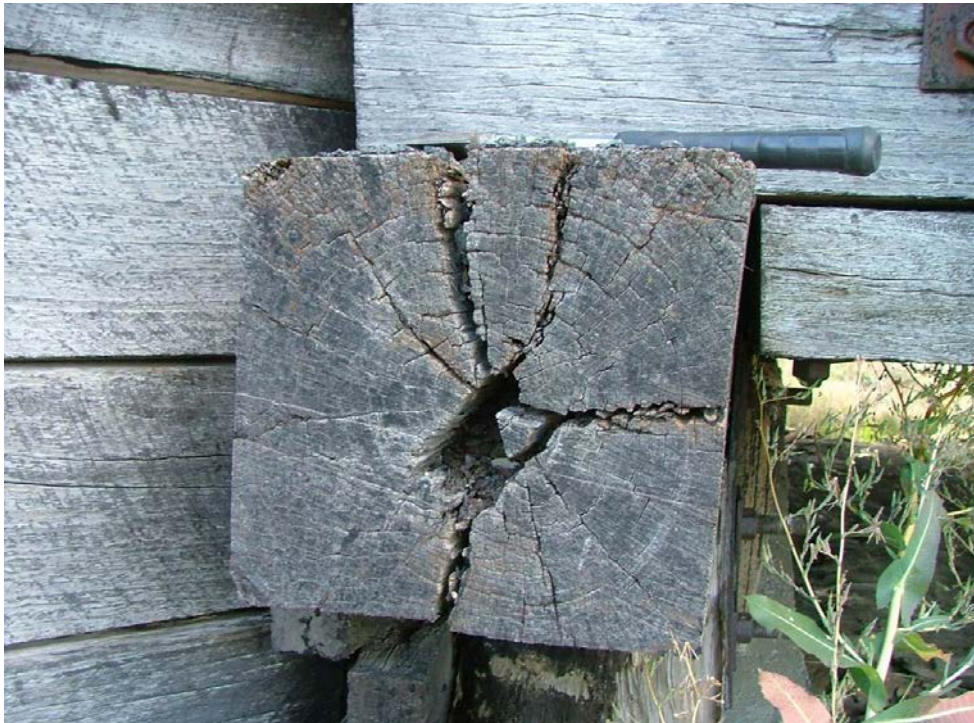
Medium rot and splitting of the headstock.
