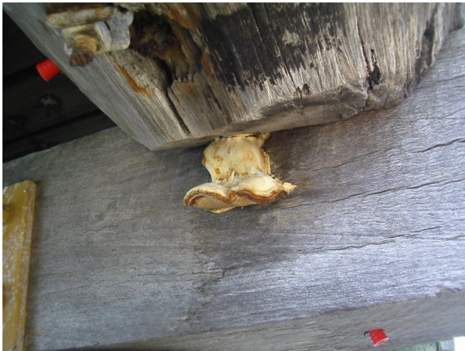
Fungal growth on a corbel.
