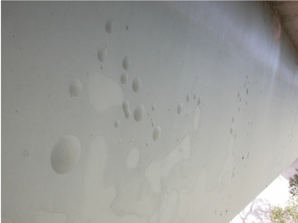
Blistering of topcoat.
