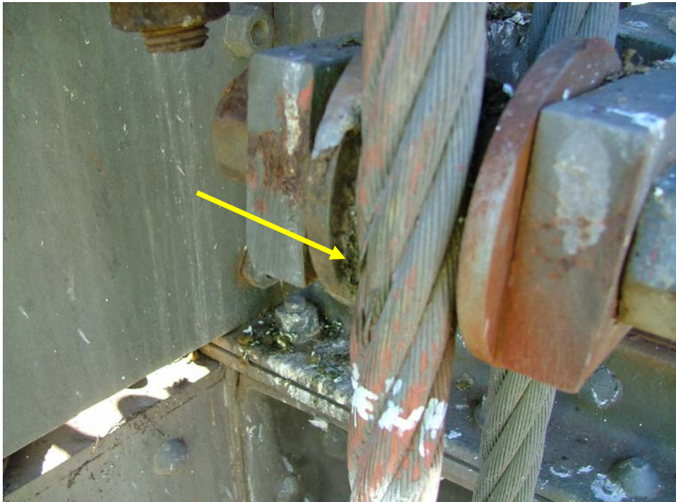
Lift span cable with broken wires.
