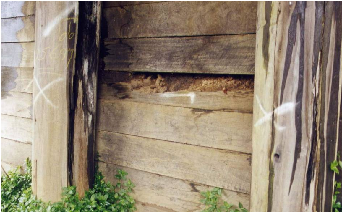
Broken abutment sheeting.
