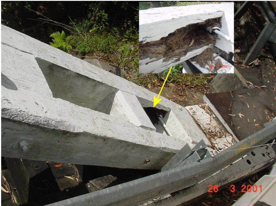
Major rot near the bottom of the principal.
