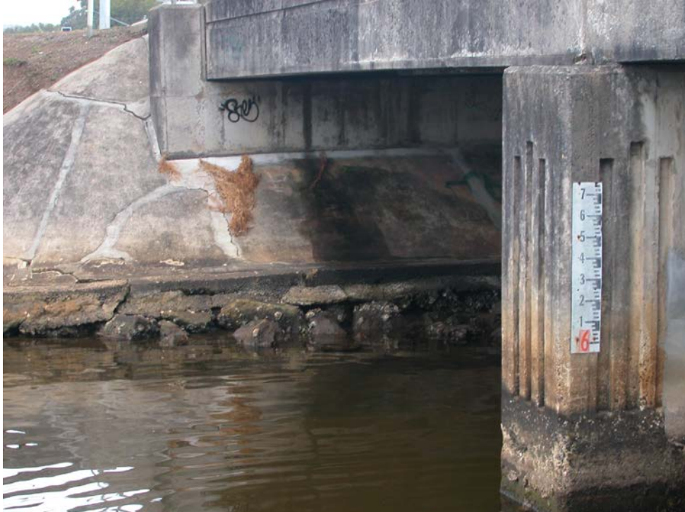
Moderate scour at the base of batter protection.
