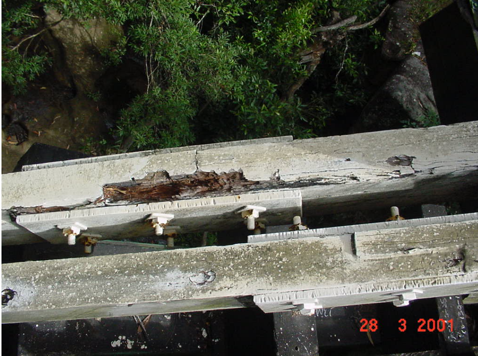
Rotting at the bottom chord flitch at the splice.
