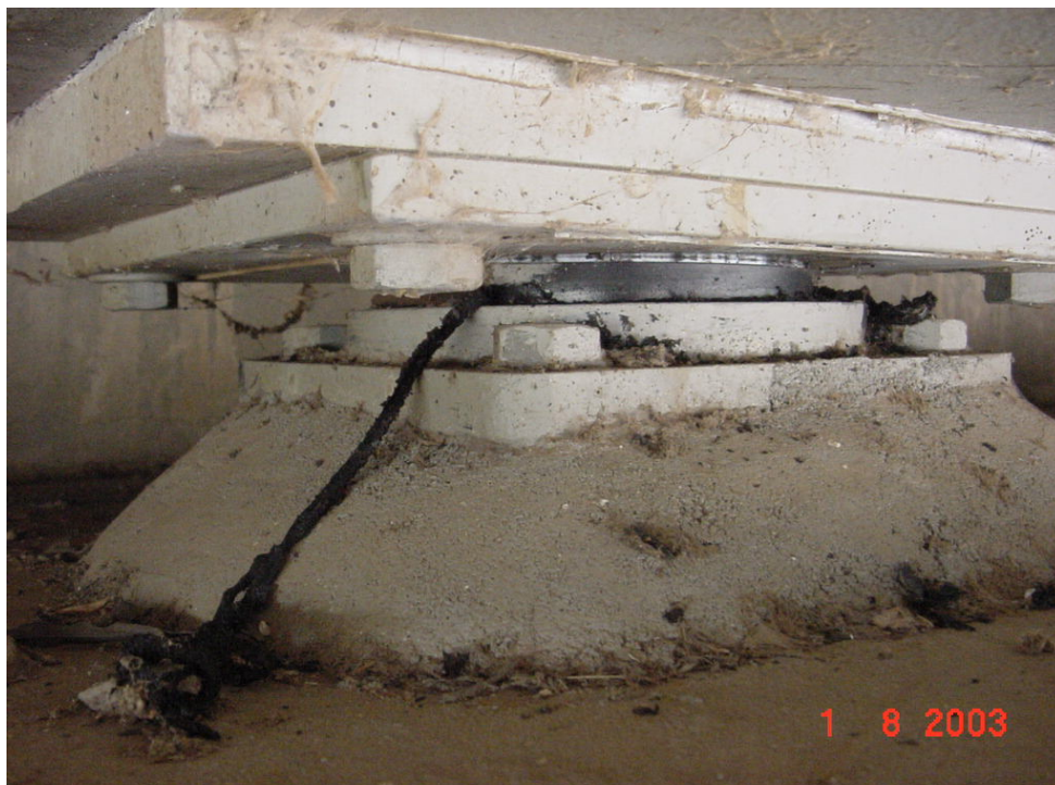
Moderate leakage of rubber.
