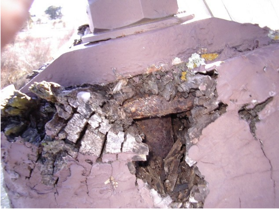
Major rot on end of top chord with crushing of timber and tilting of tension rod bearings.
