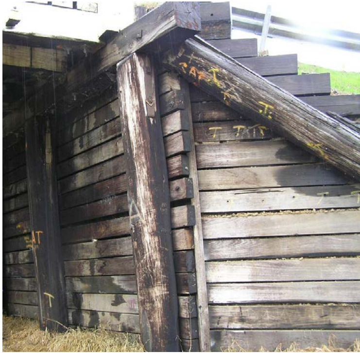
Abutment sheeting with some termite infestation.
