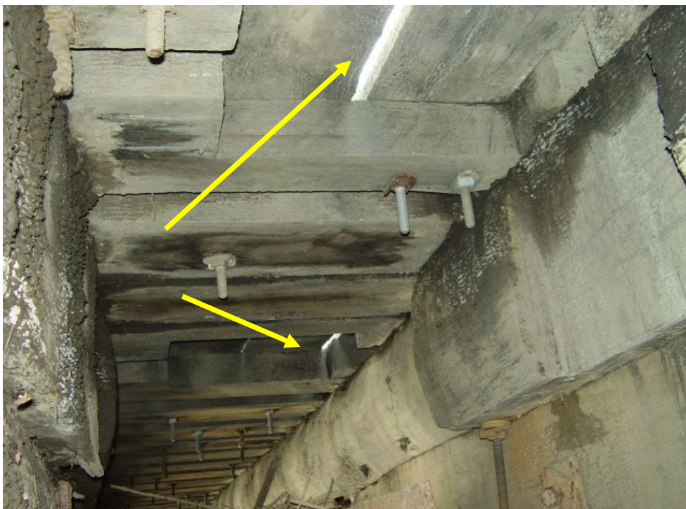
Missing sections of cross decking.
