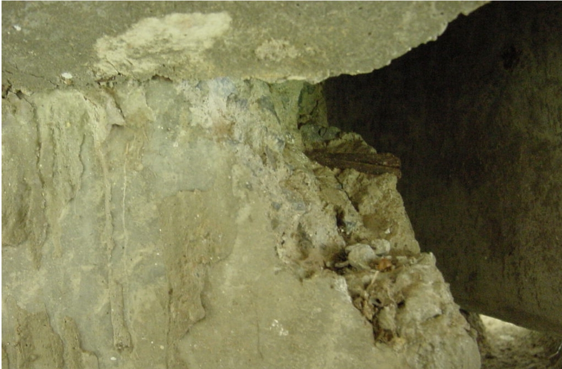
Cracked and spalled end of a 13.7m span pre-tensioned girder with exposed tendon.
