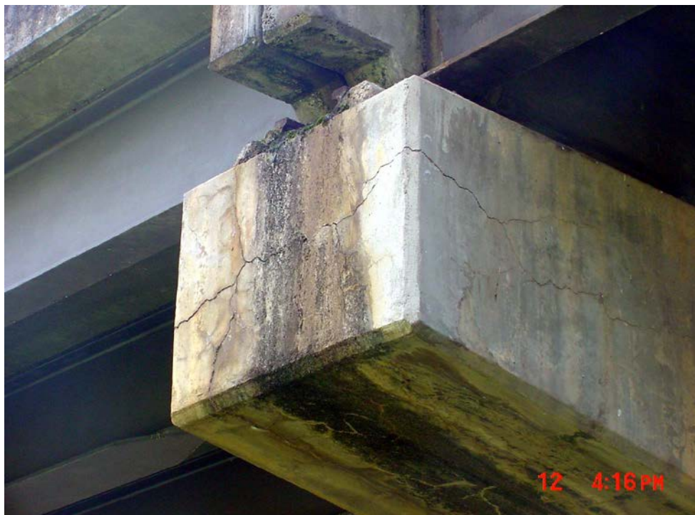
Significant cracking of the headstock in all faces. Pattern is typical of AAR.
