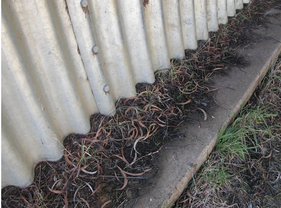
Dirt buildup retaining moisture that can result in corrosion at the base.
