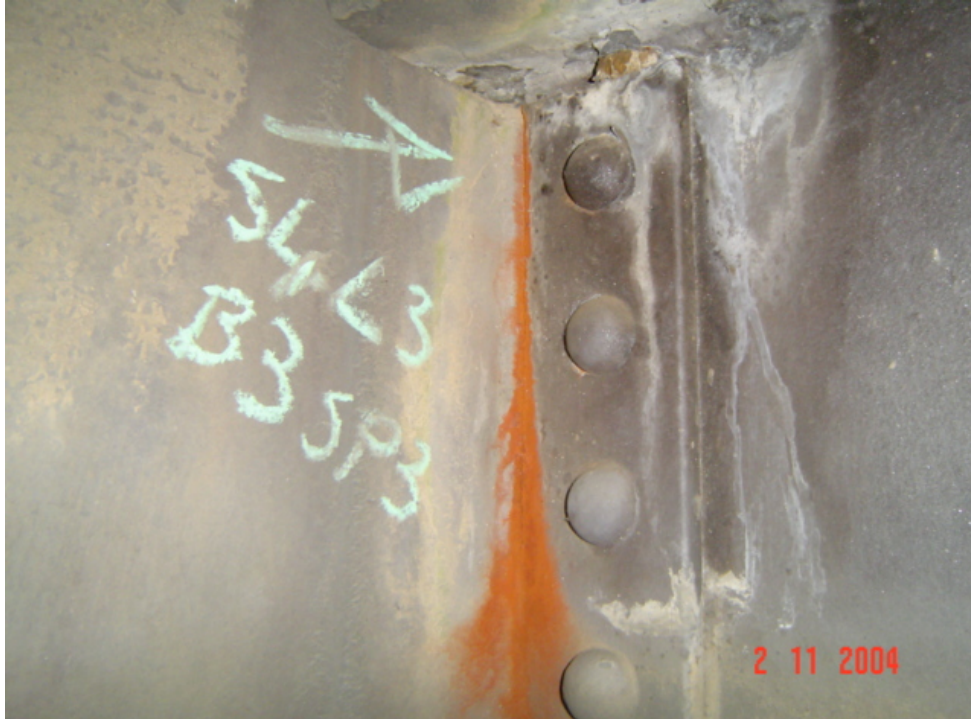
Crack in weld at connection with cross girder.
