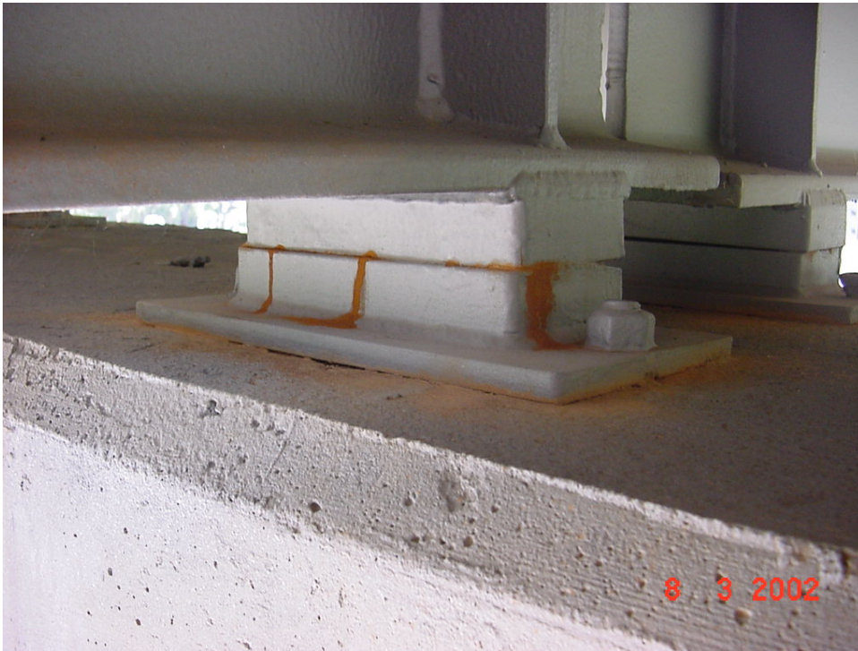
Signs of corrosion at the edges of interface.
