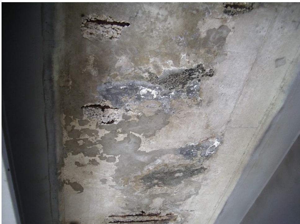
Concrete deck soffit with spalling, leaching and corroding reinforcement.
