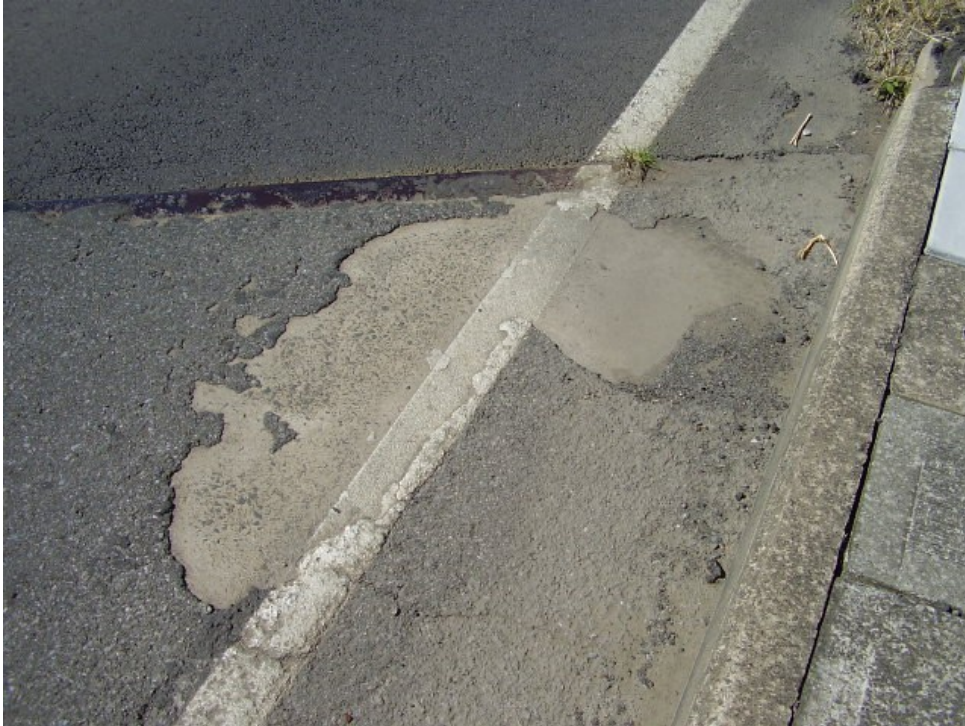
Stripping of wearing surface in small area.
