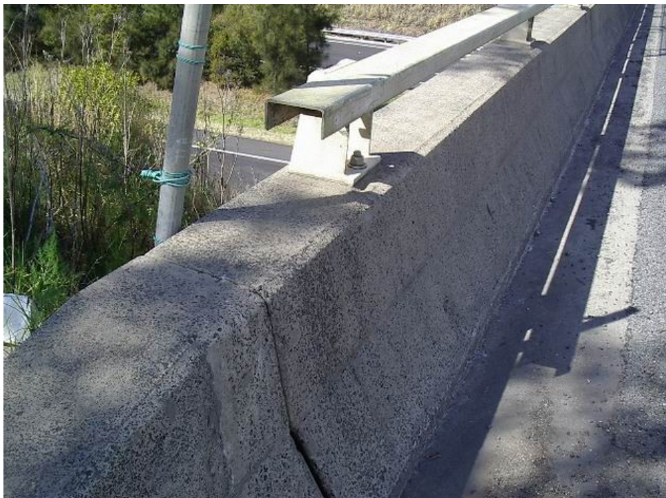
Metal railing without suitable end piece with significant risk to the safety of road users.
