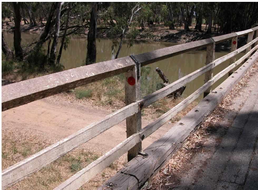
Failed paintwork on a timber railing.
