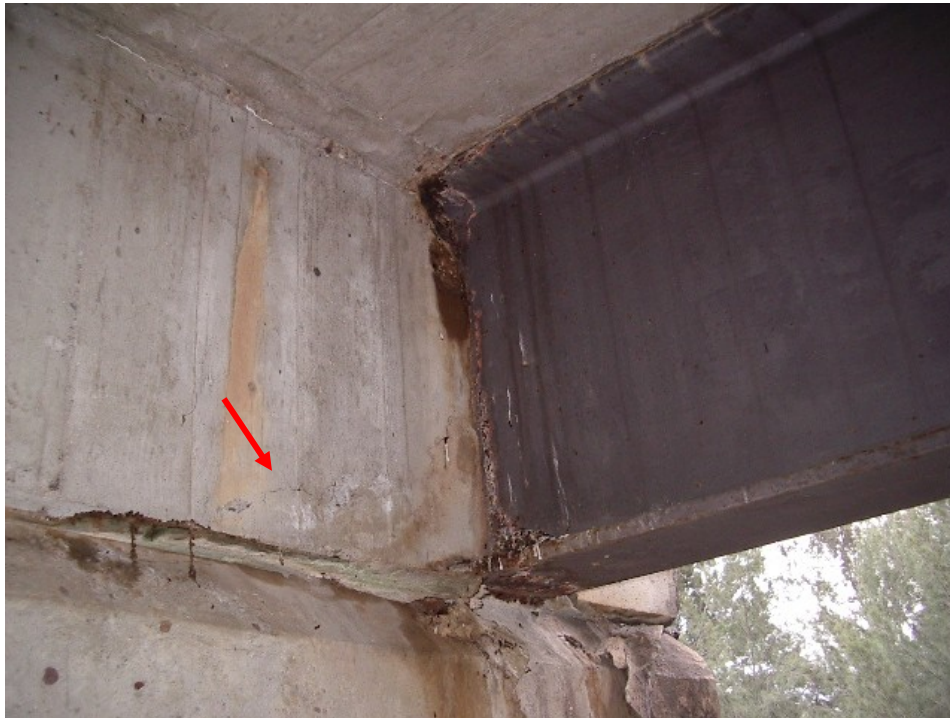
Cracked cross girder.
