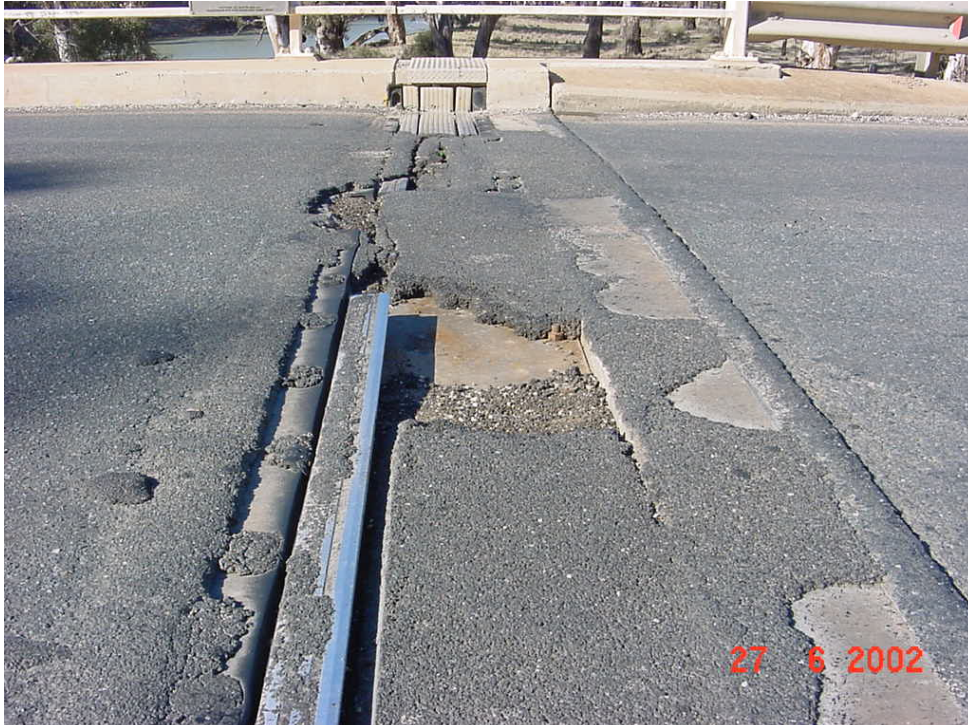
Joint in poor condition.
