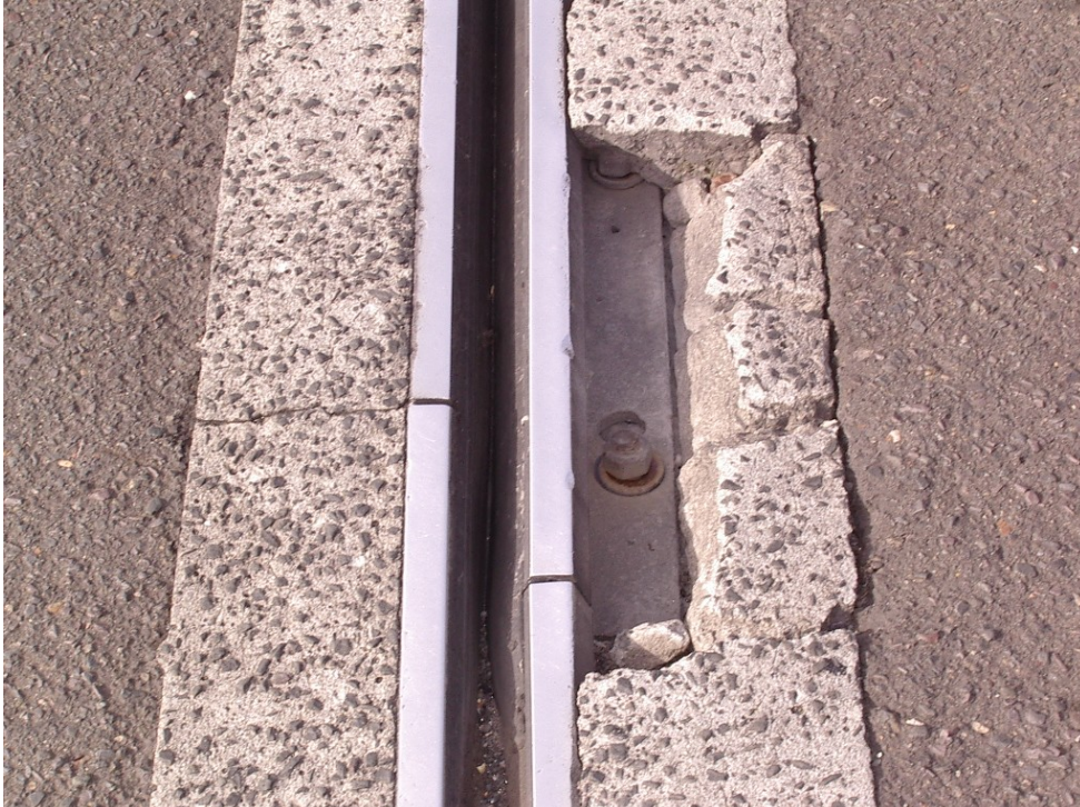
Significant spall and loose nut.
