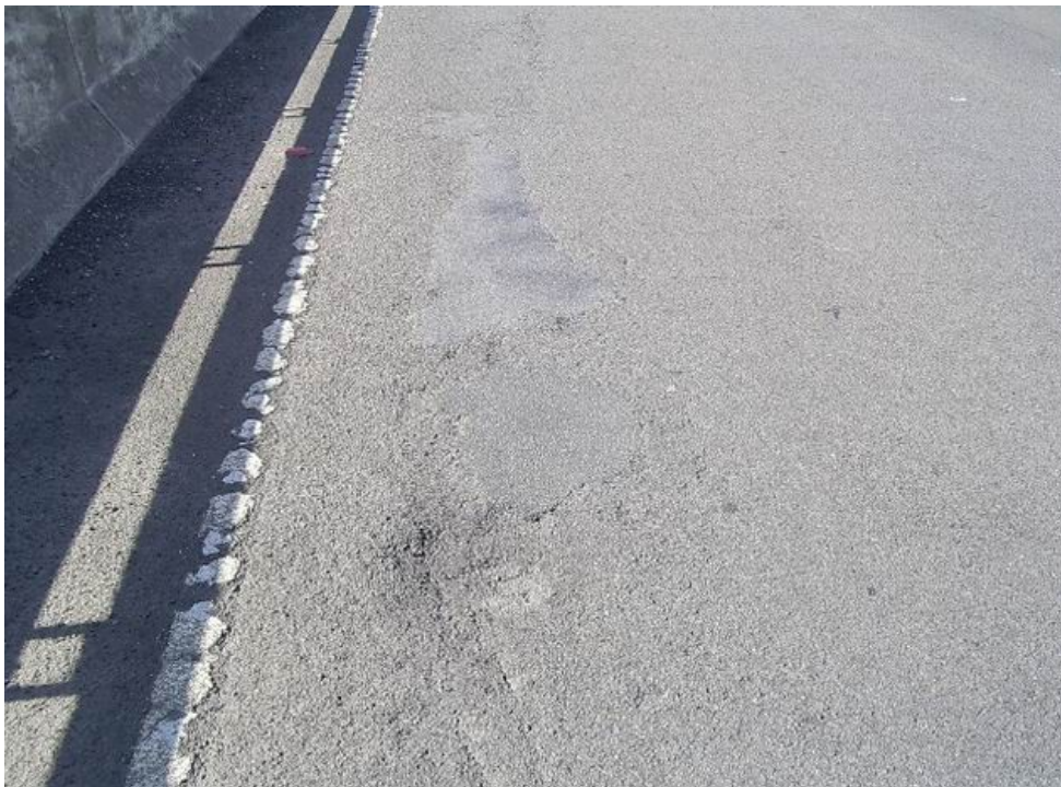
Wearing surface breaking up near some repaired areas.
