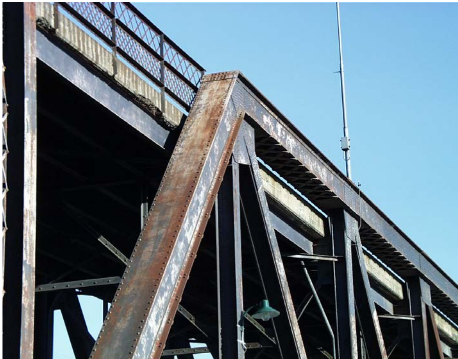
Uniform surface rust on principal. Rusting heavier on the edges and near rivets.
