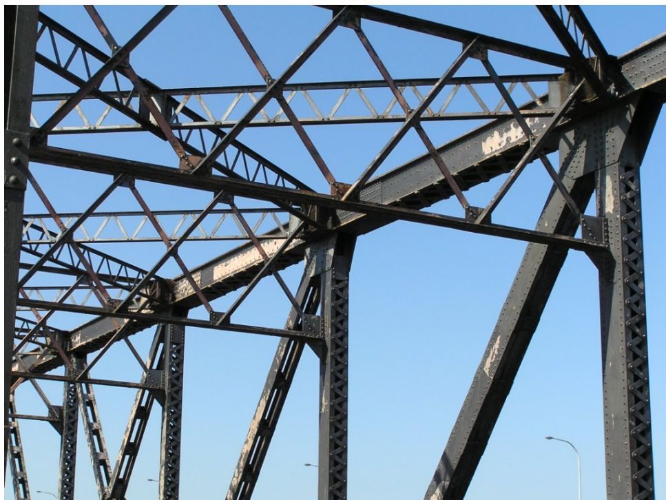
Breakdown of top coat with primer exposed over large areas.
