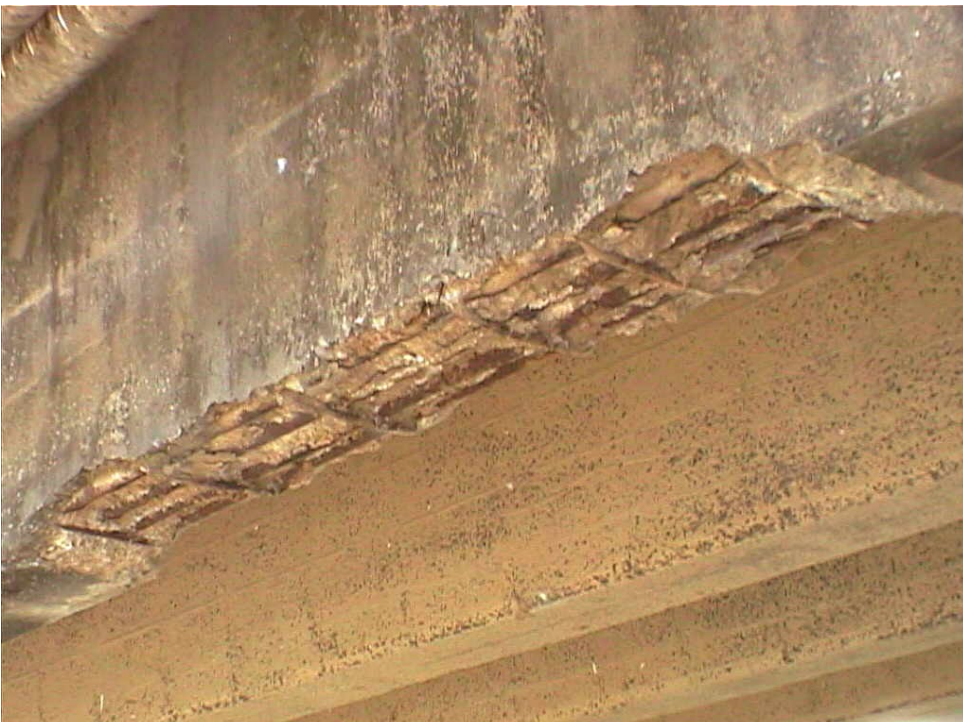
Severe spalling and delamination. Exposed and corroding reinforcement.
