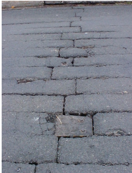
Damaged ends of longitudinal sheeting on rotten cross decking.
