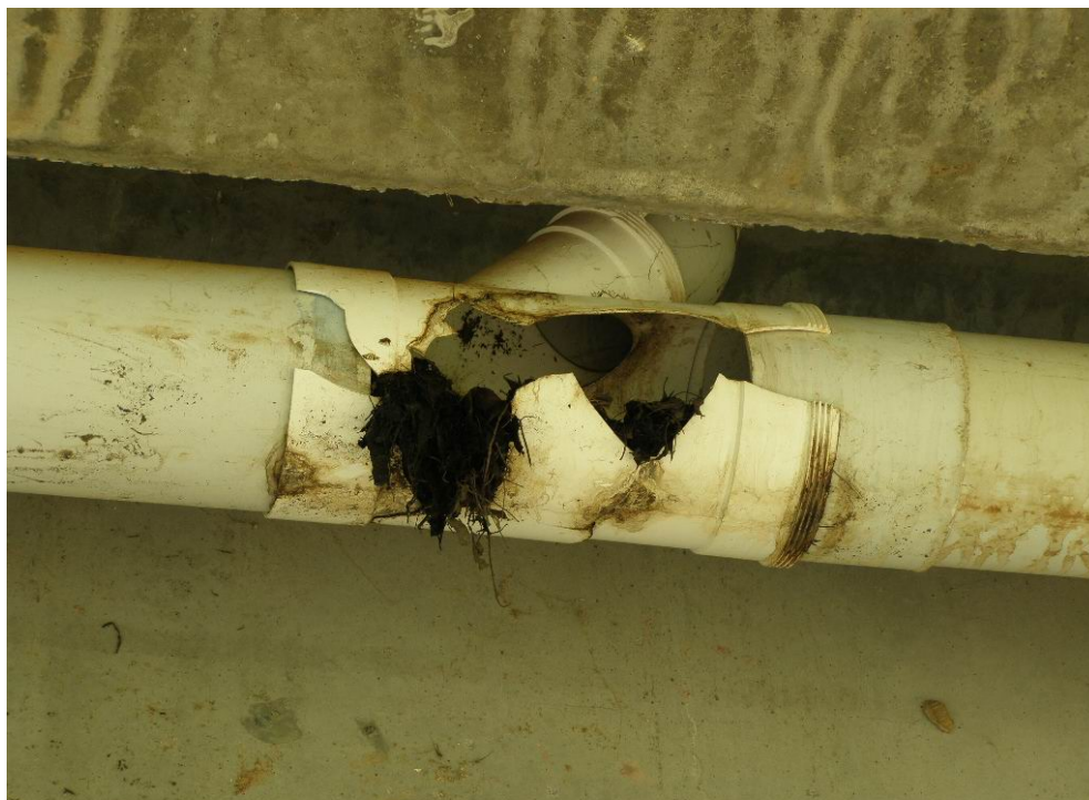
Broken joint in the drainage system.
