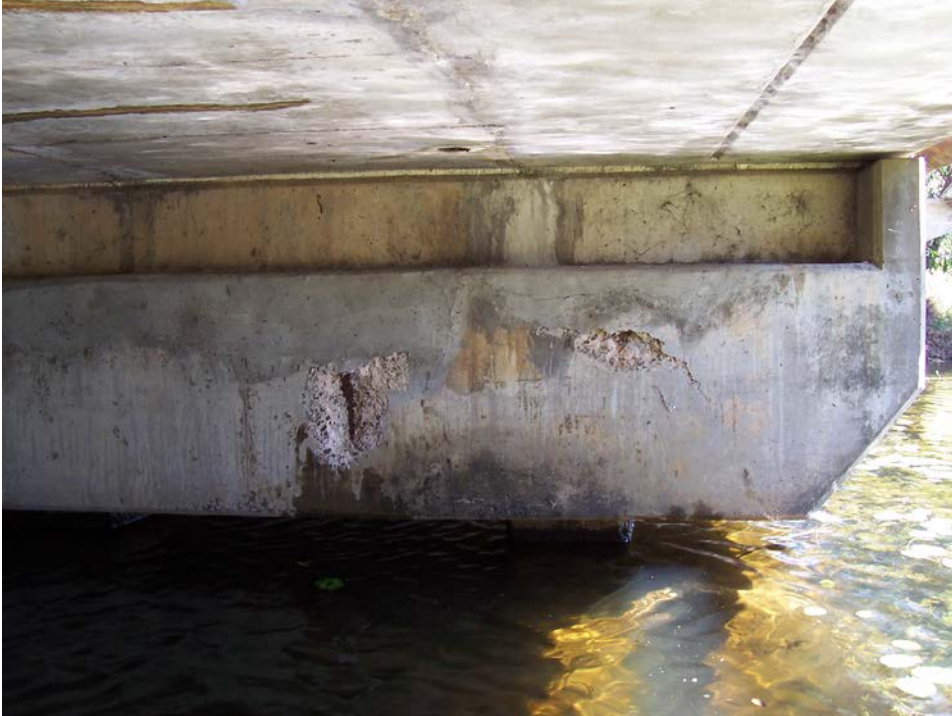
Spalling of the concrete with exposed reinforcement. Some previously repaired area cracking again.
