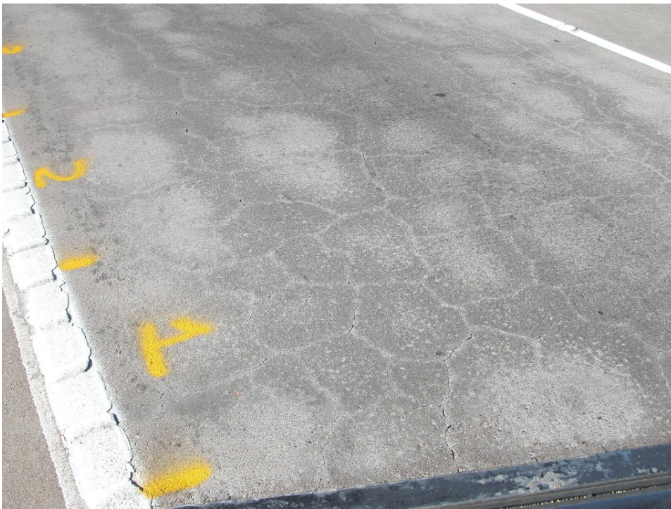
Significant fine cracking of deck slab.
