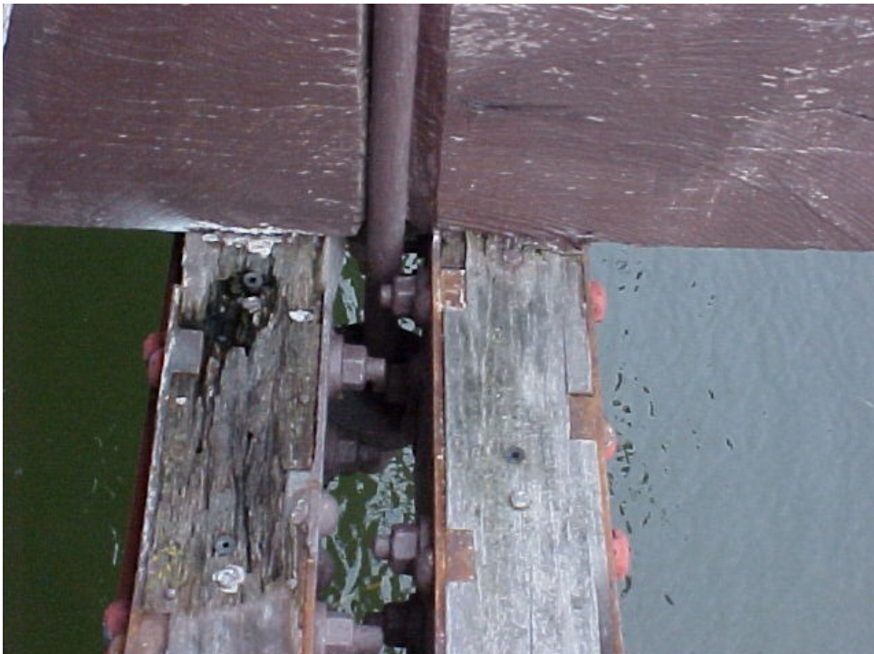
Rotten section of bottom chord.
