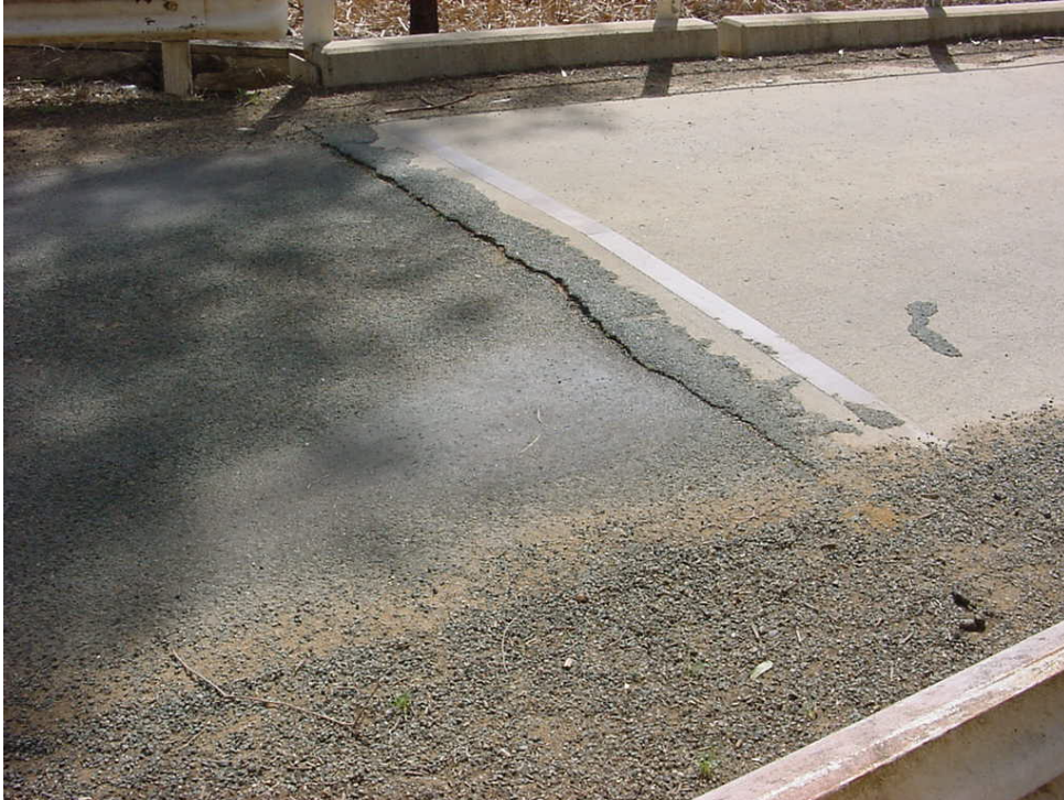
Nominal drop of the approach carriageway.
