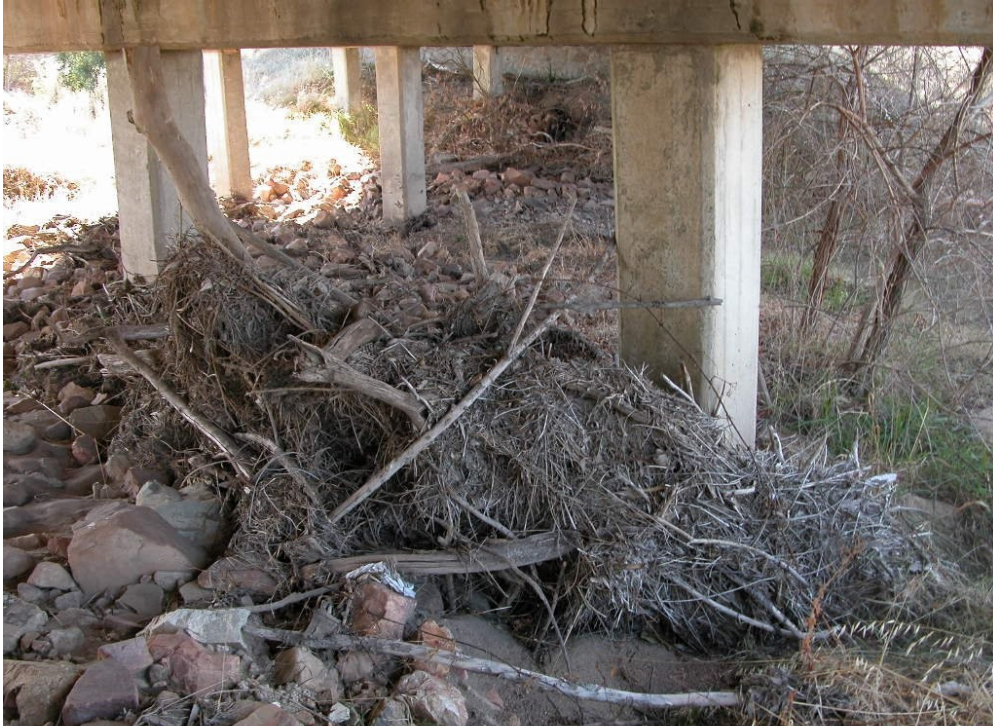
Waterway with some debris but not significant.
