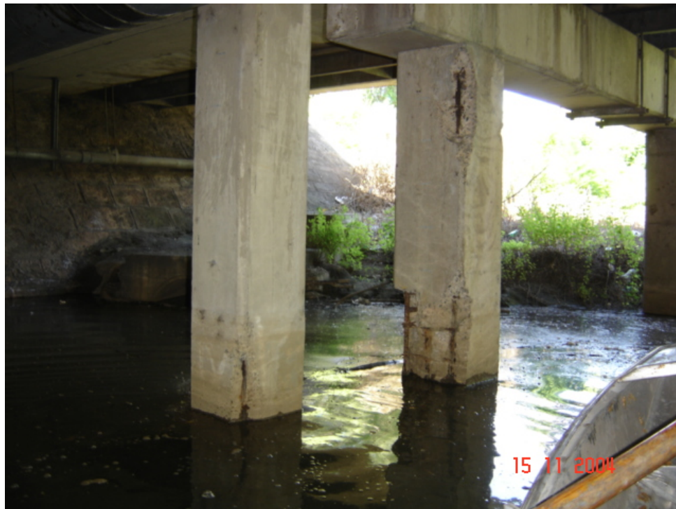
Advanced deterioration and significant loss of section.
