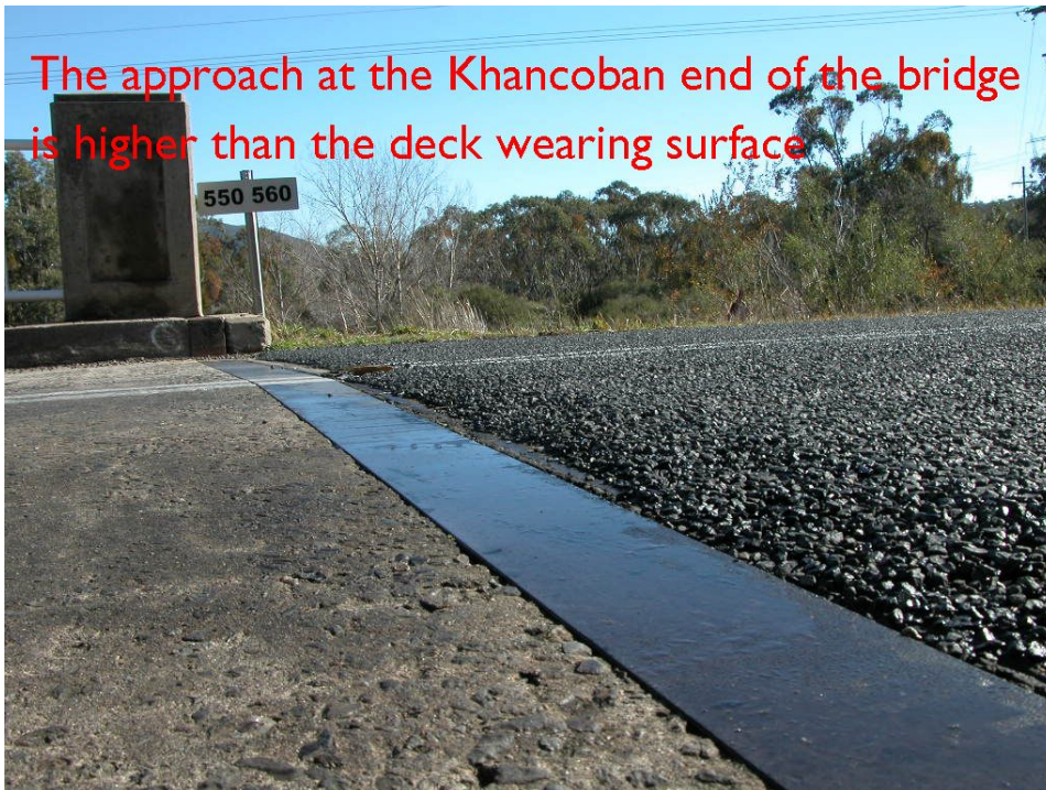
A noticeable drop of the approach carriageway wearing surface level at the bridge.
