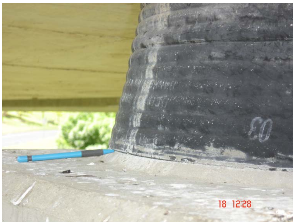
Elastomeric bearing showing excessive shear deformation.
