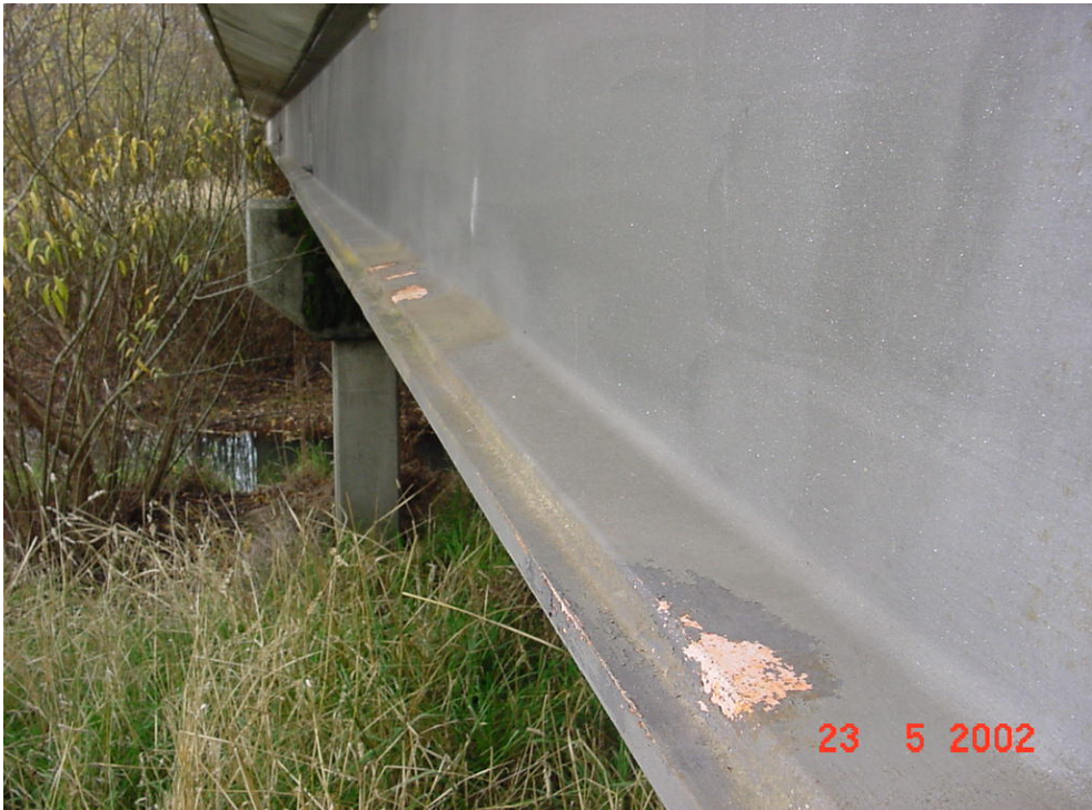
Minor coating deterioration but no steel deterioration.
