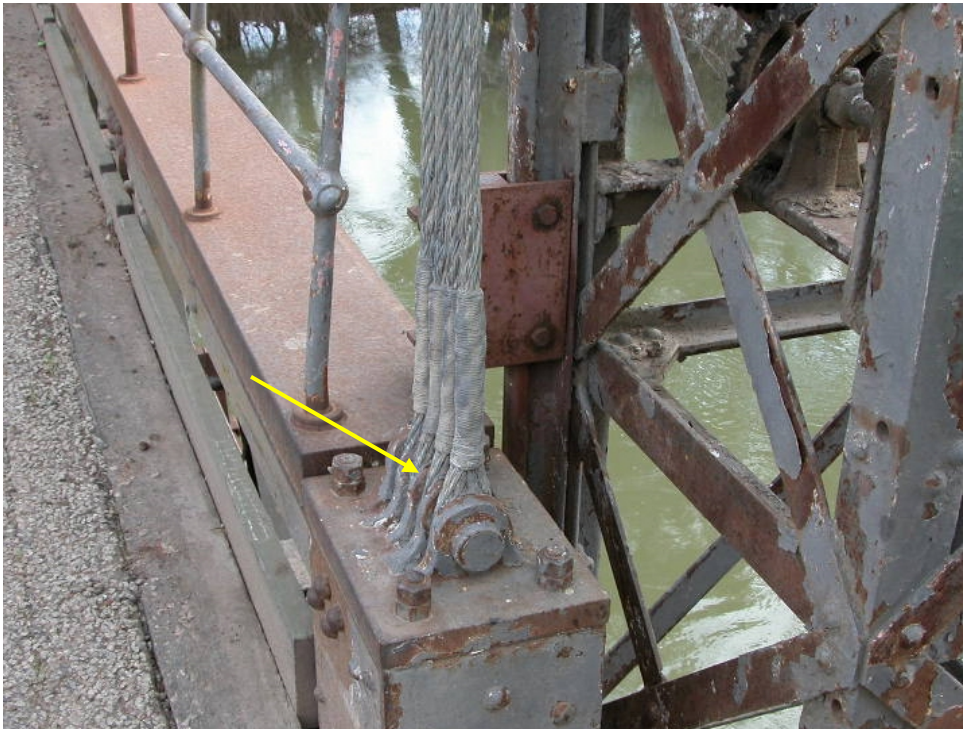
Surface rust on lift span wire cable and connection.
