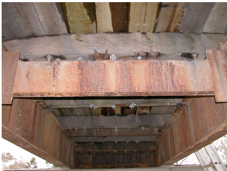
Extensive surface rusting.
