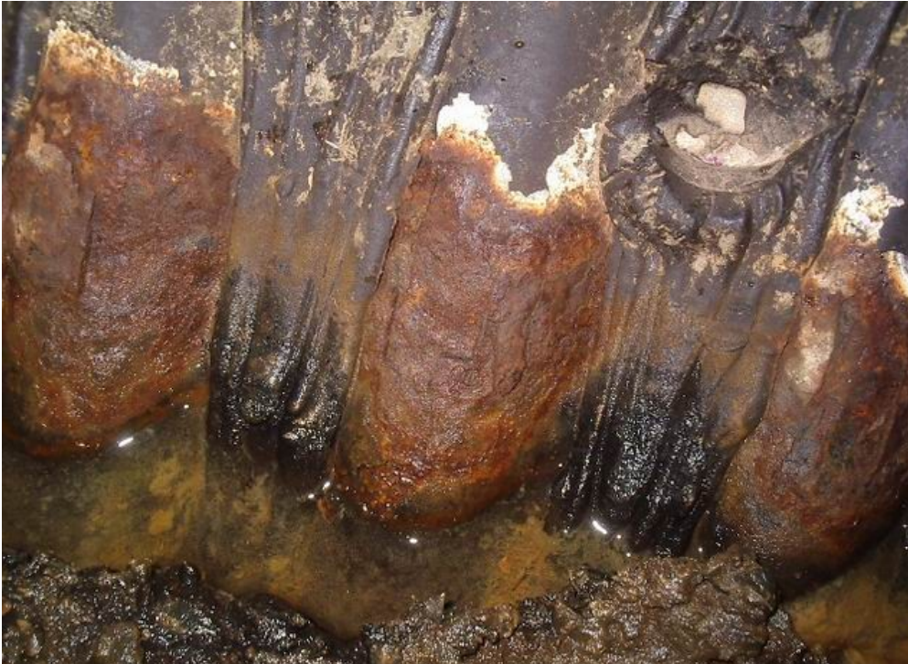
Major corrosion with some distortion.
