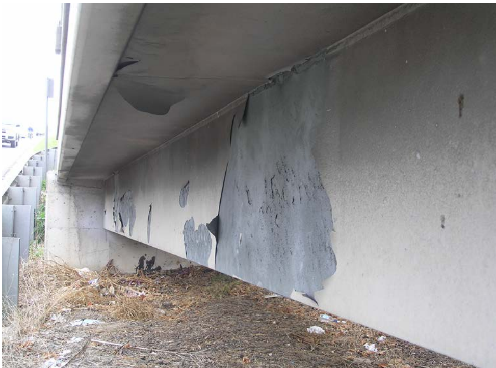
Large areas of delaminated coating. No longer providing effective protection.
