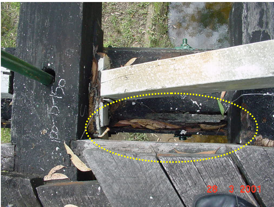
Medium decay of the bottom chord.
