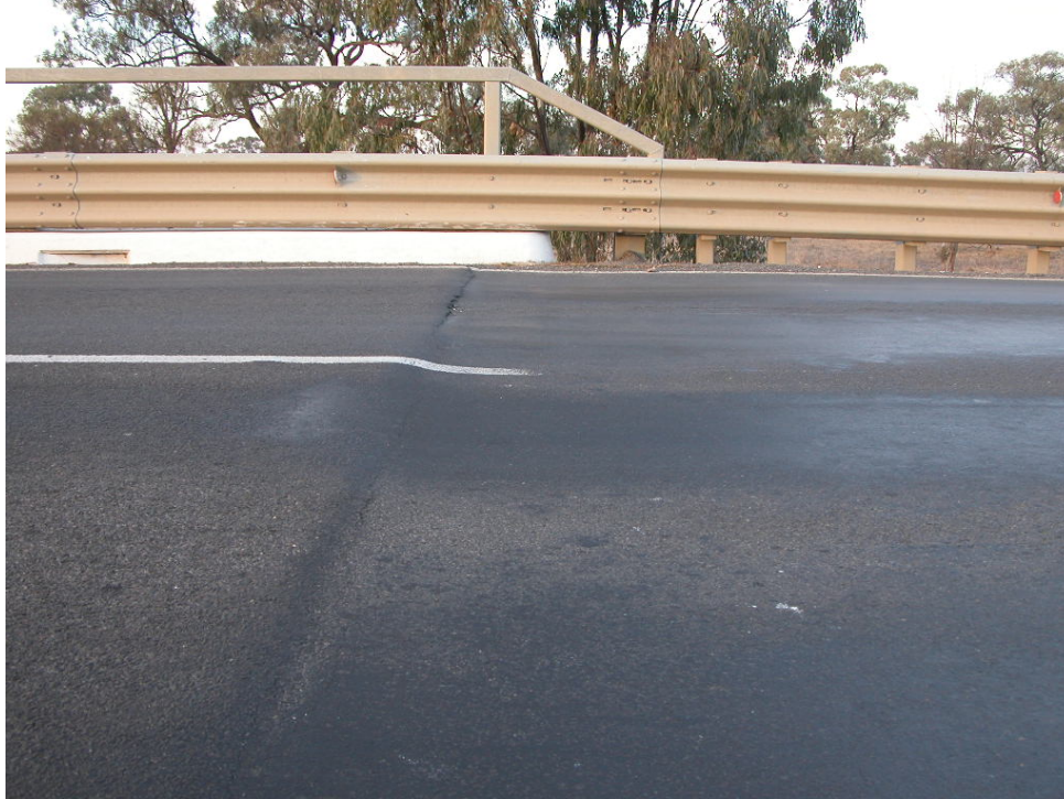
Significant settlement of approach carriageway.
