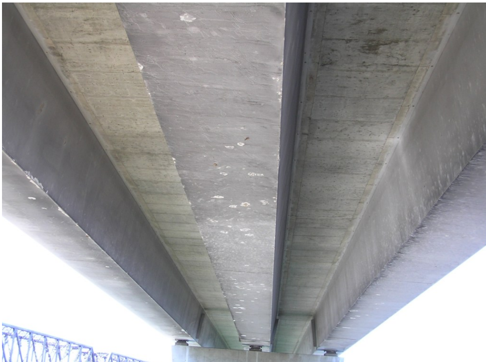
Localised failure of zinc primer.
