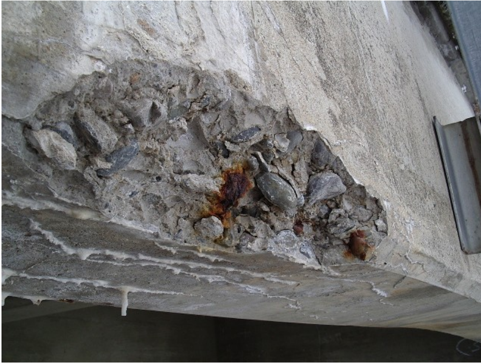
Spall on external girder. Exposed reinforcement with corrosion setting in.
