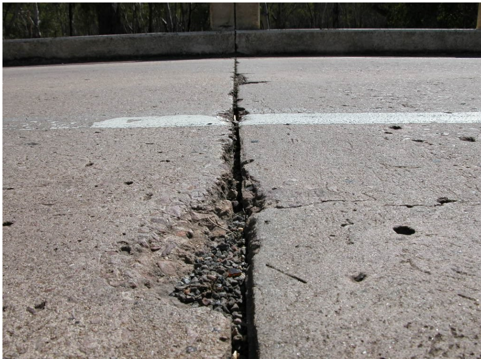
Large spall and debris blocking the joint.
