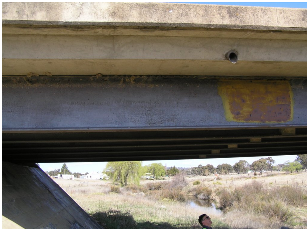
Failed patch of top coat.
