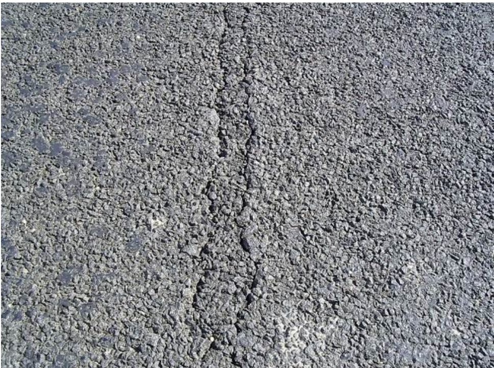
Asphaltic concrete above pourable joint is cracked indicating loss of adhesion
