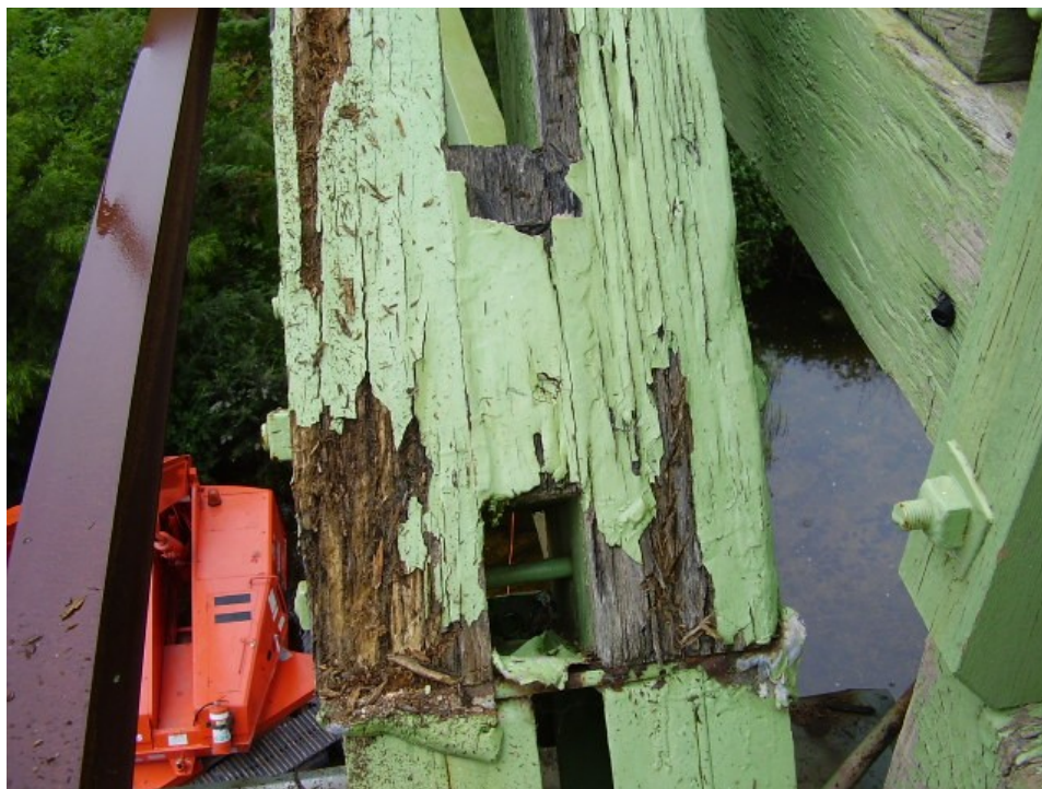
Rot on the principal
