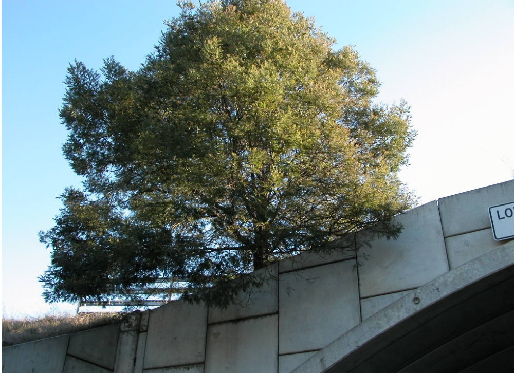
Tree close to the structure. To be removed.
