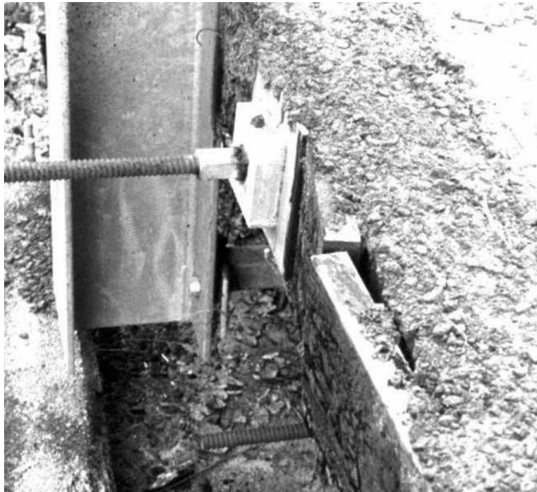
Edge laminates breaking away from the deck.
