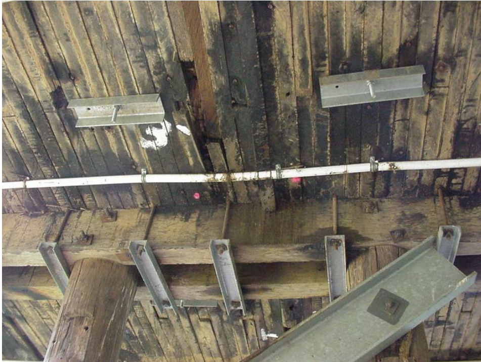
Stress laminated deck in poor condition.
