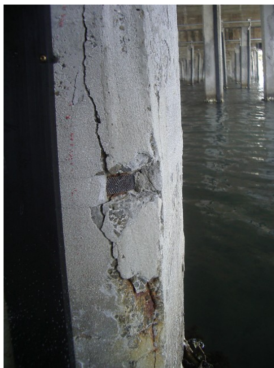
Major vertical cracking and extensive spalling. Cathodic protection mesh exposed. Signs of corrosion.
