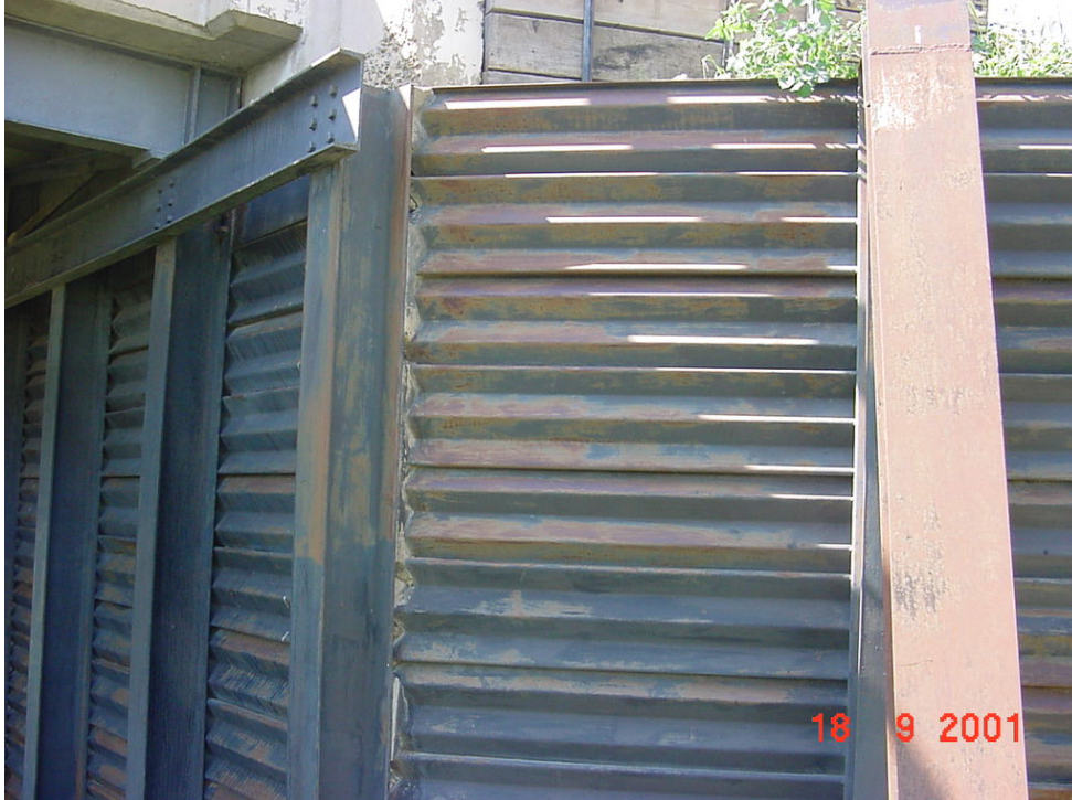
Light surface rusting on sheeting and supports.
