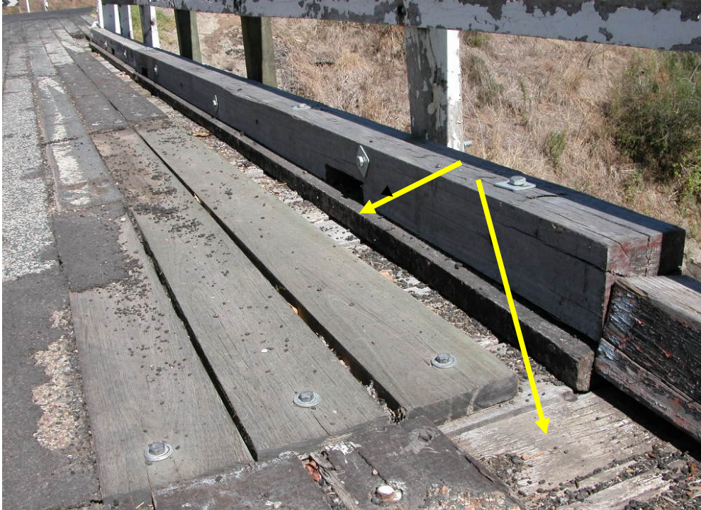
Longitudinal sheeting with minor splitting. Large gap near the kerb and a missing plank.
