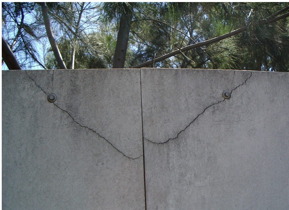
Noise wall attachment with cracks running along the holding bolts.
