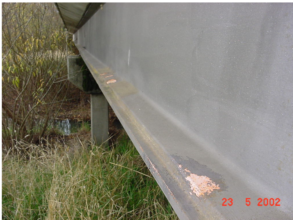
Localised patches of topcoat breakdown.
