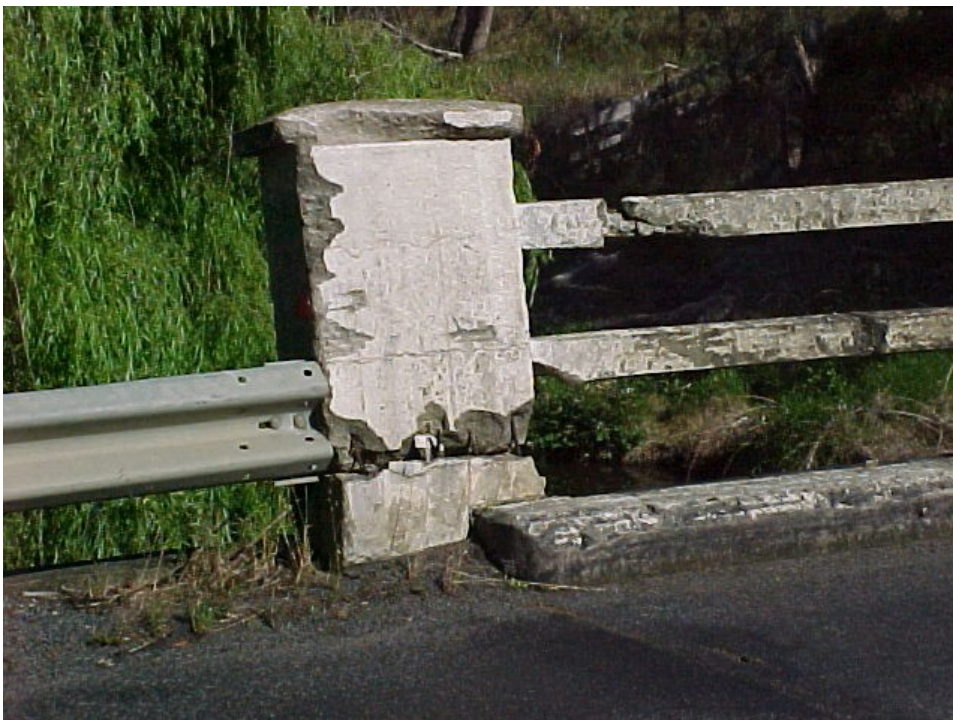
Badly damaged concrete end post and railing.
