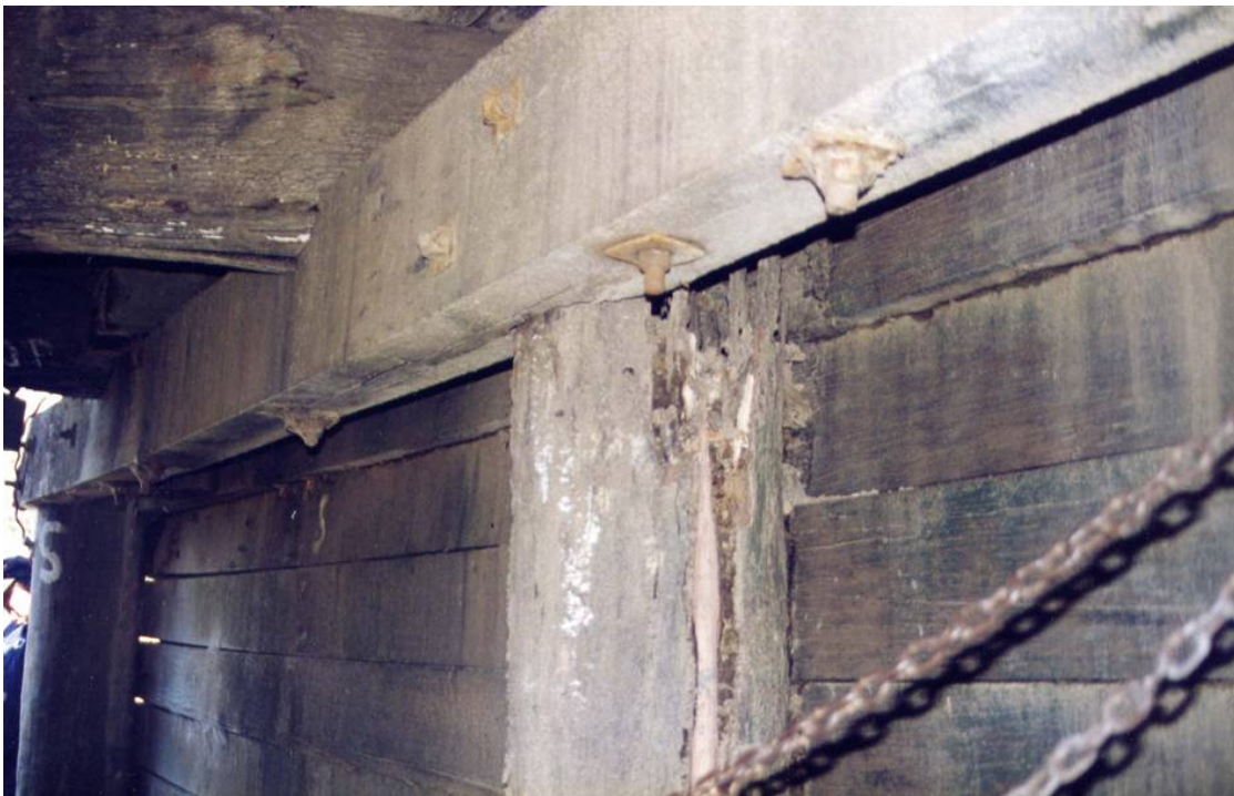
Badly rotten pile.
