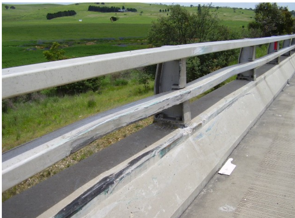
Moderate deformation of rails due to vehicular impact.
