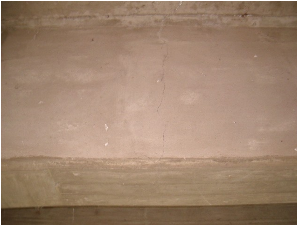
Reinforced beam with vertical crack.
