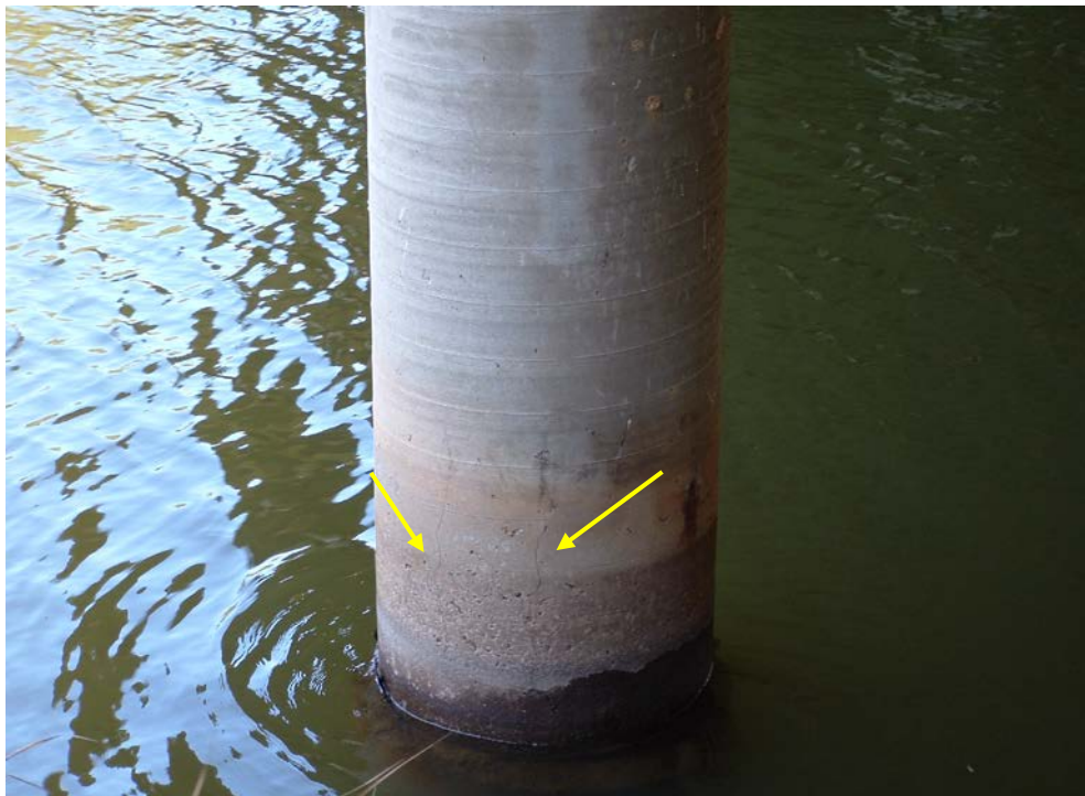
Fine cracks near the water level.
