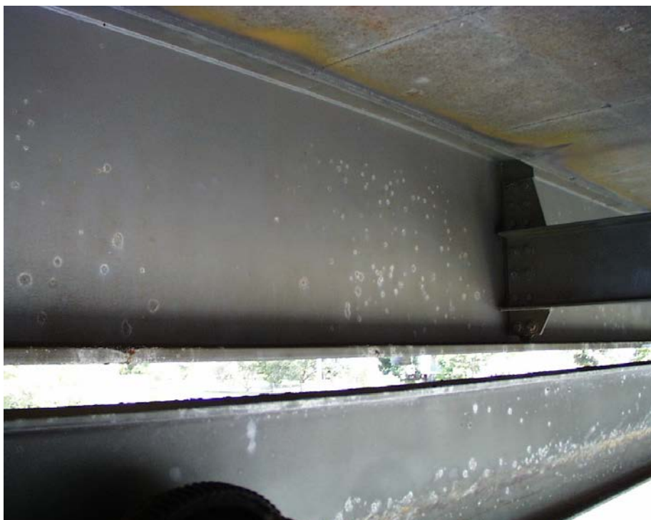
Localised failure of zinc primer with white salts evident.
