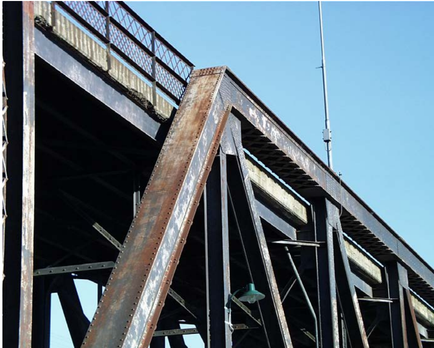
Breakdown of top coat with primer exposed over large areas.
