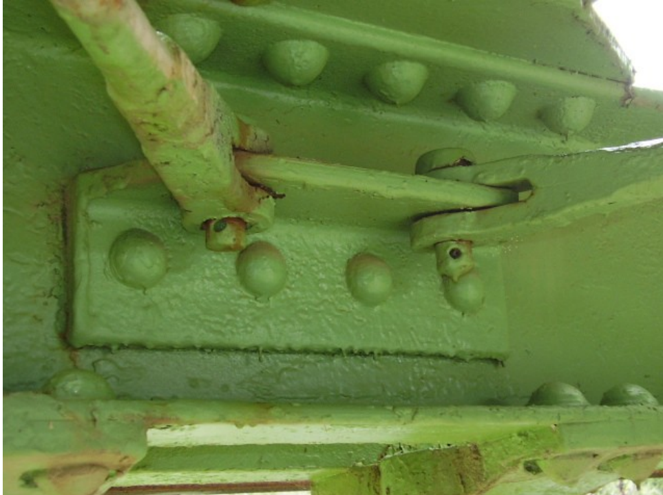
Brace tie rods with missing clips on pins.
