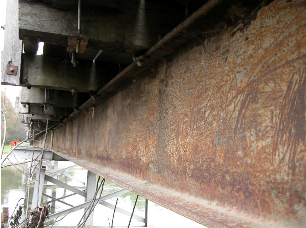
Coating no longer present.
