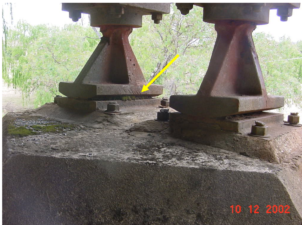
Surface corrosion and some accumulation material at the interface.
