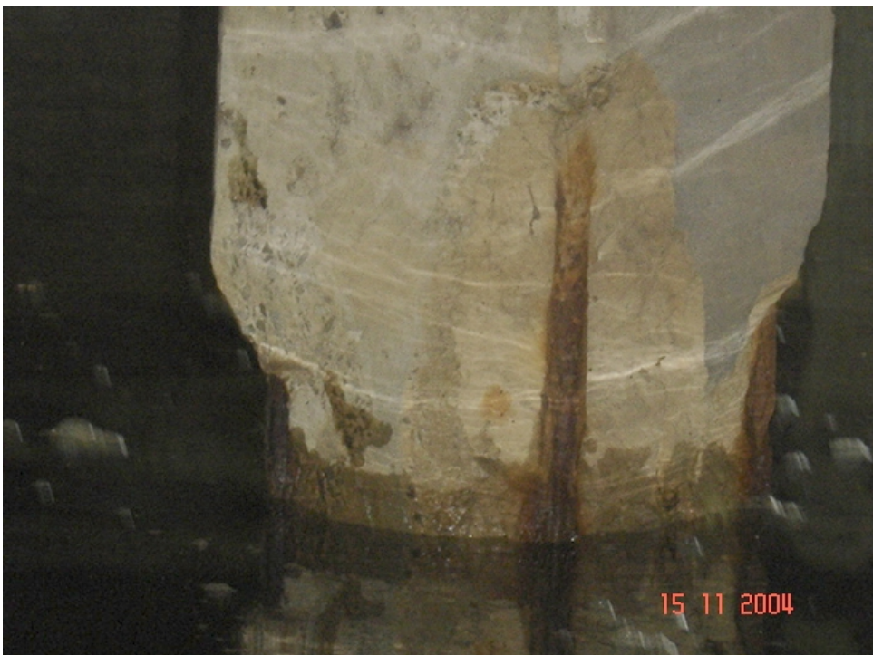
Significant loss of section of the pile and heavy corrosion of reinforcement.
