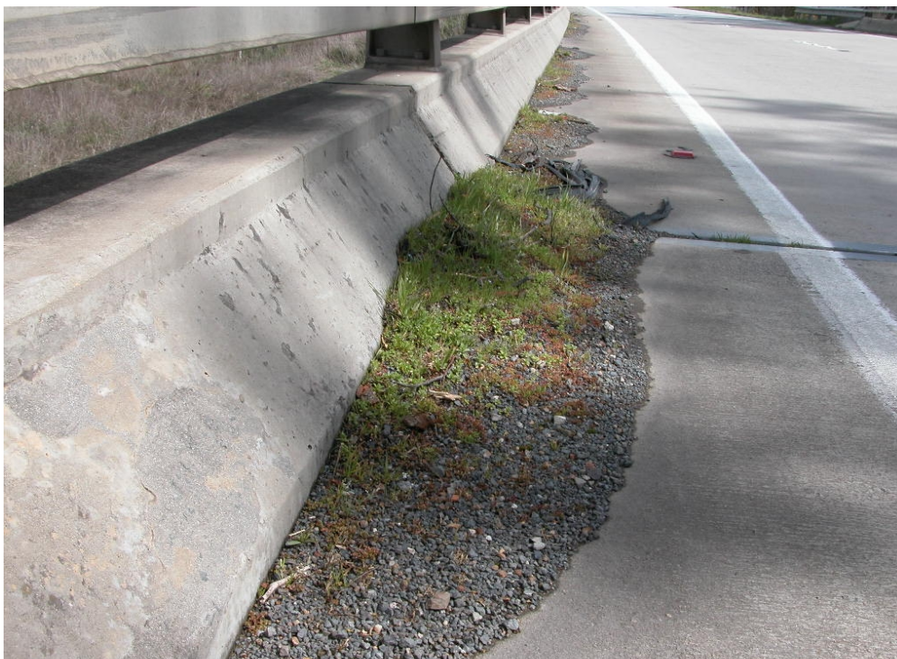
Significant buildup of dirt affecting drainage movement.
