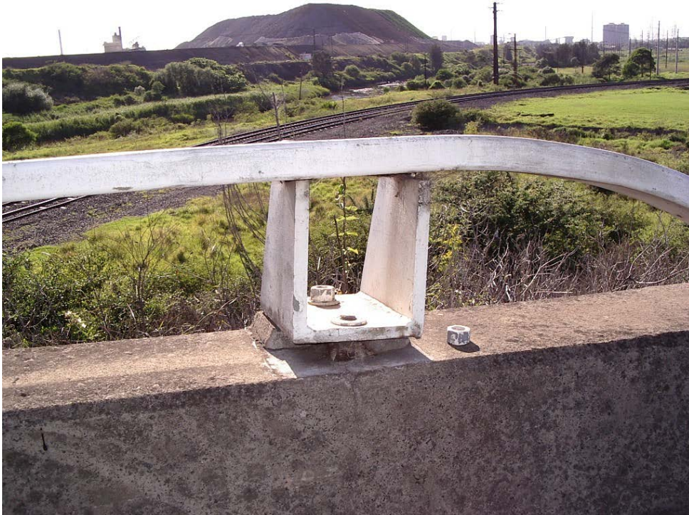
Significant damage to the metal rail base connection and moderate distortion at the end.
