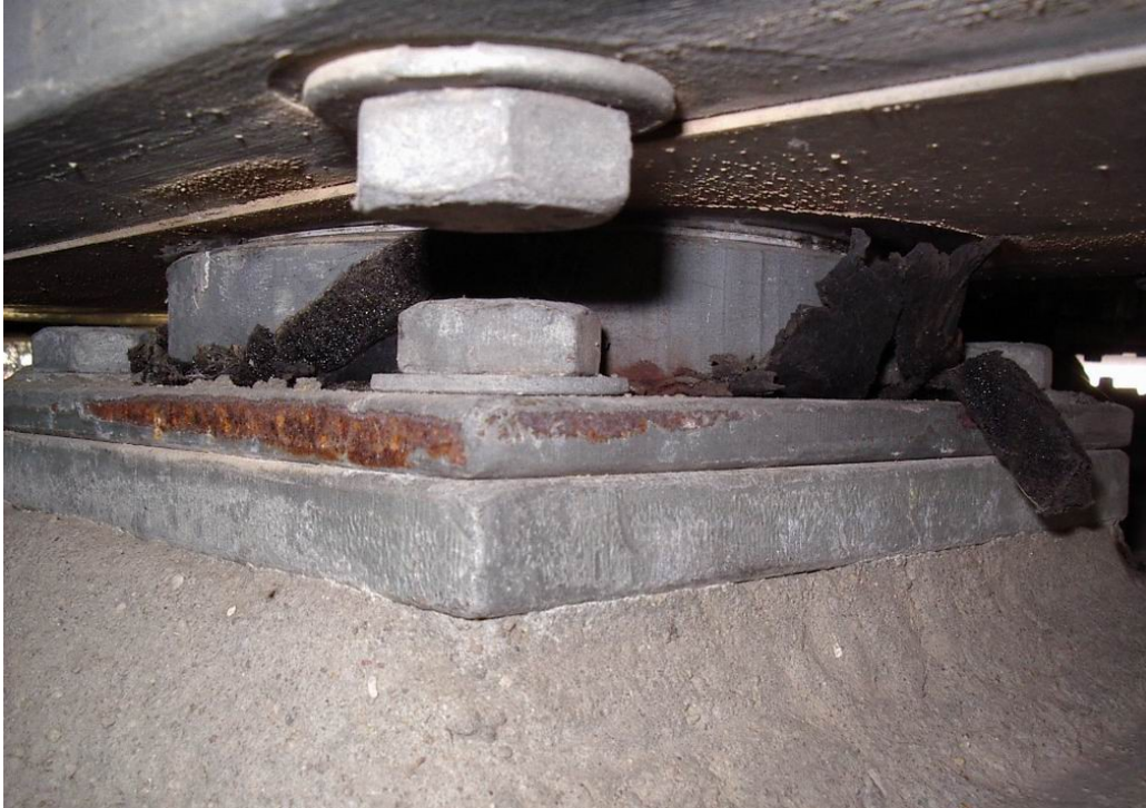
Significant leakage of rubber.
