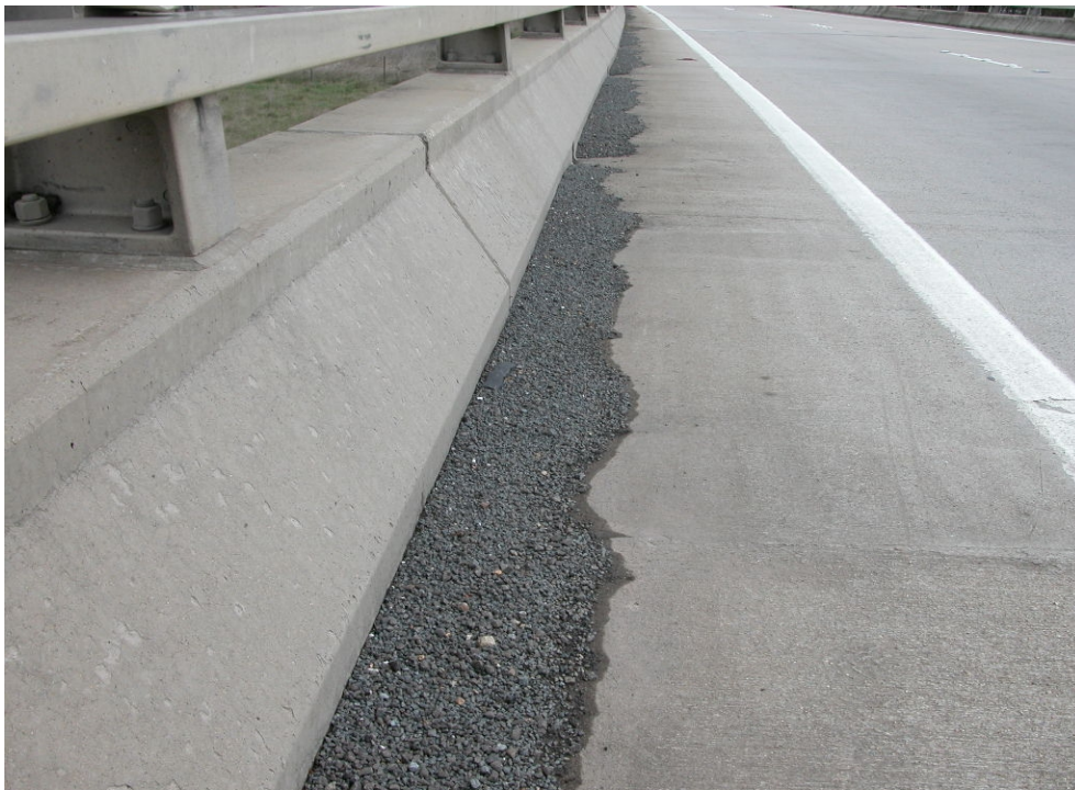
Moderate build up of dirt.
