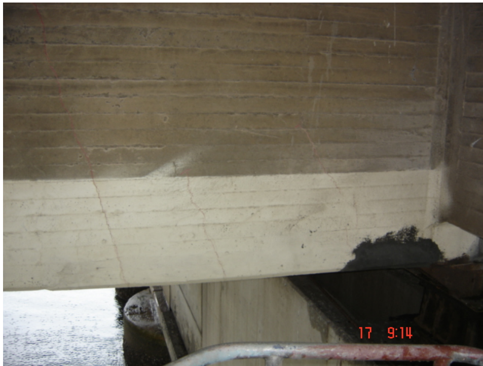
Diagonal shear cracks near support
