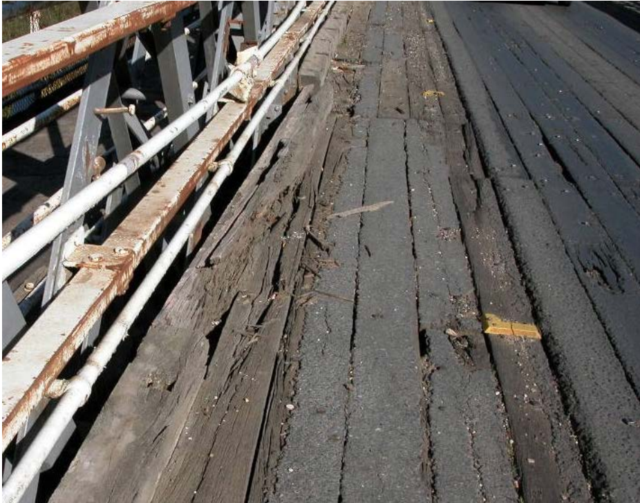
Timber kerbs split and rotten.
