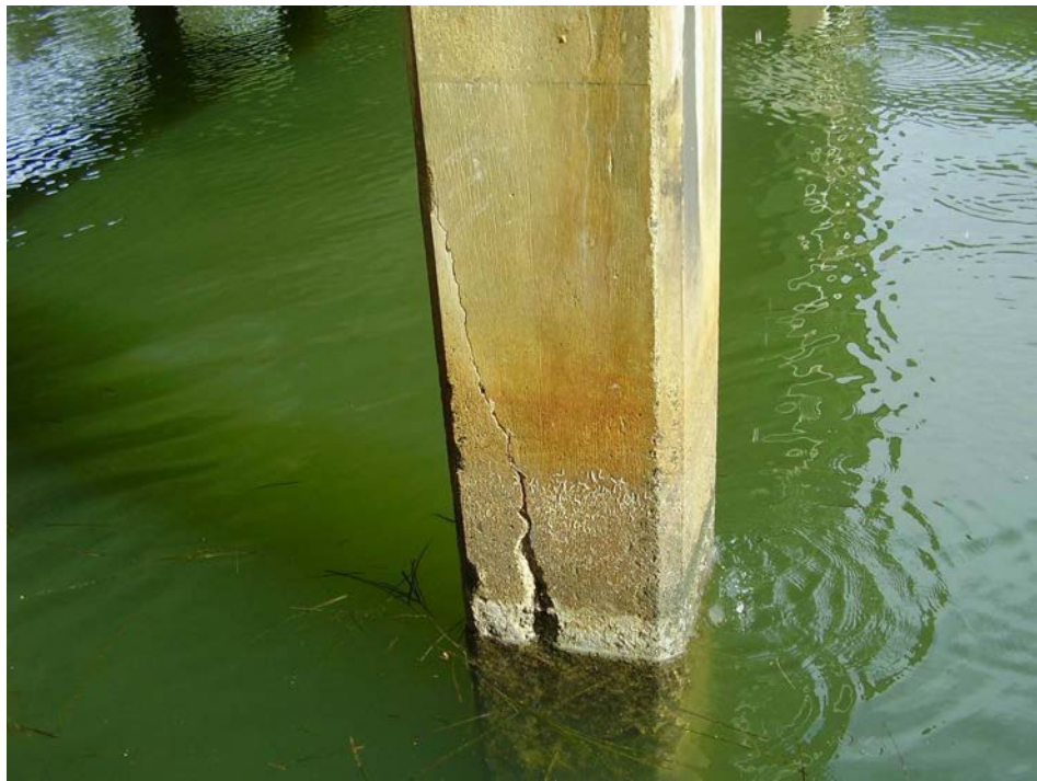
Major cracking of corner of a pile with damaged area extending up to 500mm under water.
