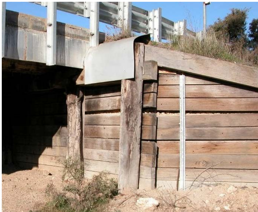
Timber abutment sheeting showing differential settlement.
