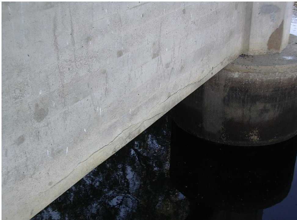
Horizontal crack along the bottom edge. No exposed reinforcement
