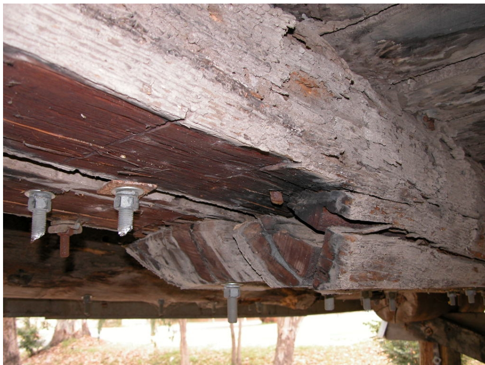
Vertically split girder with other horizontal splits at the snipe.
